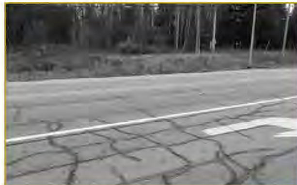
Six-year-old highway with premature cracks, in Coldwater, Ontario.
