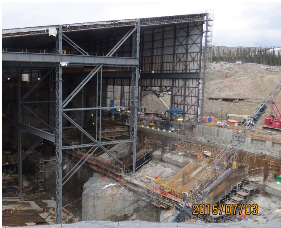
Photo 2: Intake structure (under ICS) status at end June 2015. ICS in place over units 1 and 2, with little concrete placed in the intake (towards the background of the photo).
