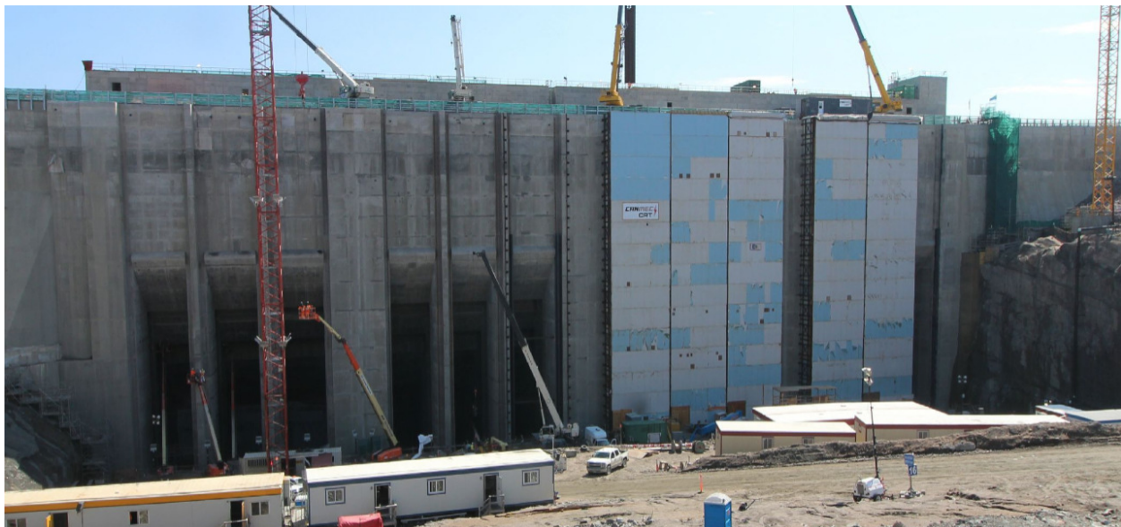
Photo 4: The intake structure as viewed from upstream on 31-July-2018. Civil construction nearing completion in units 3 and 4 on the left of the photo, while hydro-mechanical work is underway (behind construction shelters) in units 1 and 2. Bay 1 of unit 1 (far right of photo) has embedded parts work completed, and thus the shelter is removed in the photo.
