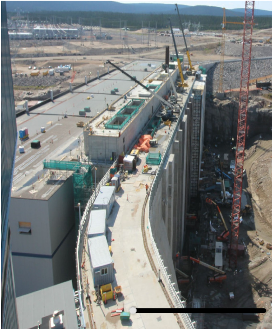
Photo 5: Top of intake structure, including Gate Hoist Building, as seen from the spillway hoist house on 31-Jul-2018. Civil work is completing in units 3 and 4 (foreground) while hydro-mechanical installation is underway in units 1 and 2 (embedded parts being placed via the cranes in the background).
