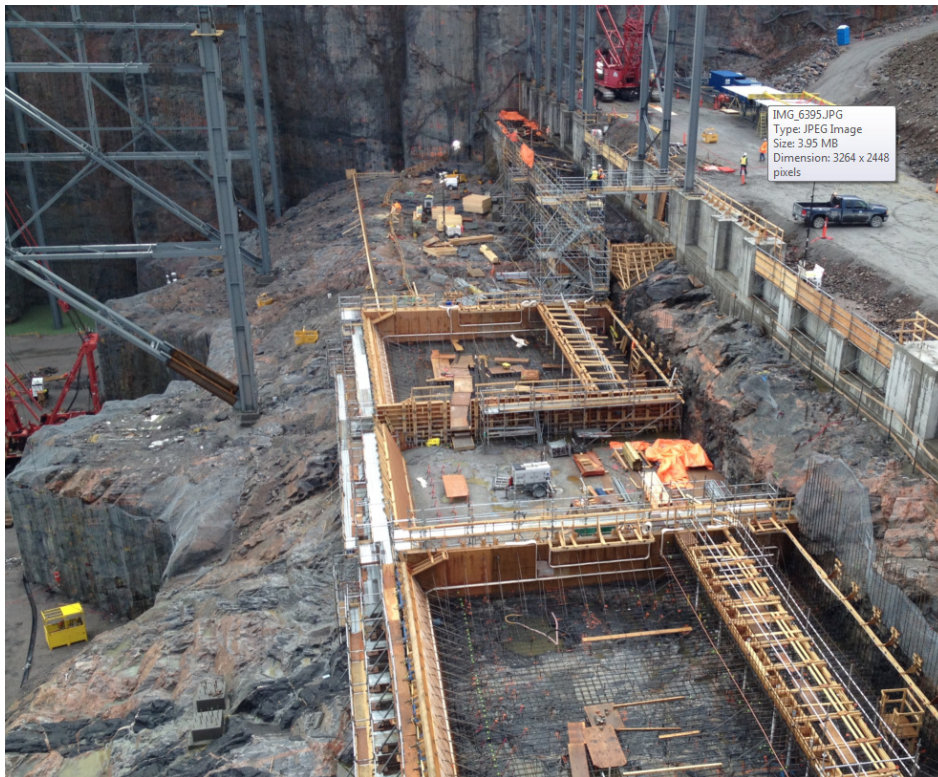
Photo 1: Intake actual status as of 10-Oct-2014. Intake 1 is in the background, next to the rock wall. Note that while formwork is being constructed, there is no concrete placed at this point.
