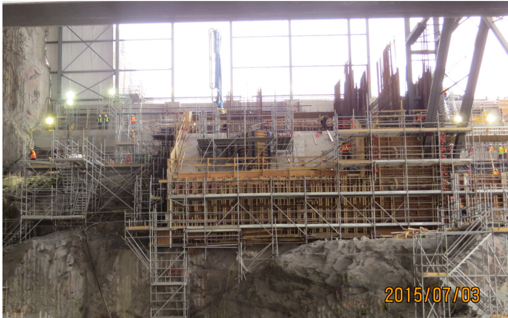
Photo 3: Intake Structure (Unit 1) status under ICS as of end June 2015. Access stairways, scaffolding and formwork, and small amounts of concrete placed.
