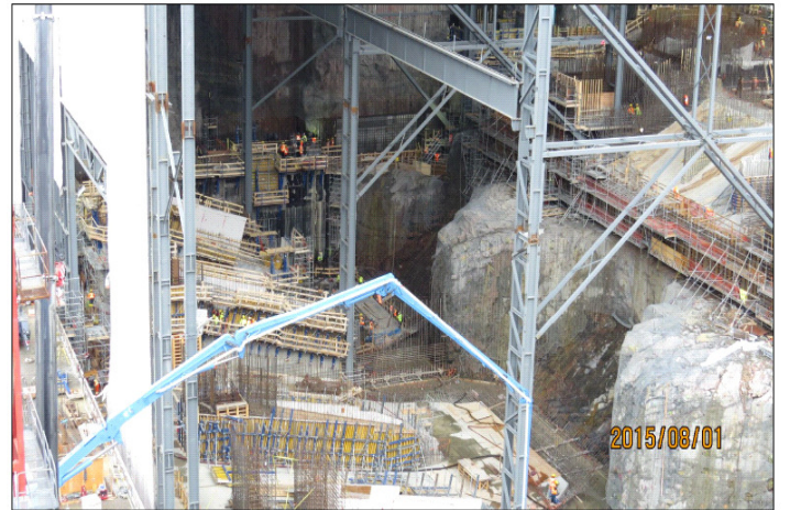
CH0007: Powerhouse Units 1 and 2
