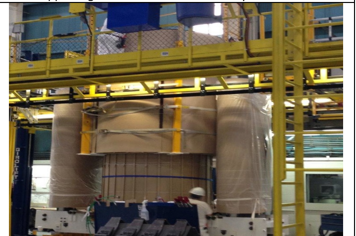
PD0537: Supply of Power Transformers, AC Substations at Churchill Falls-Autotransformer winding shop
