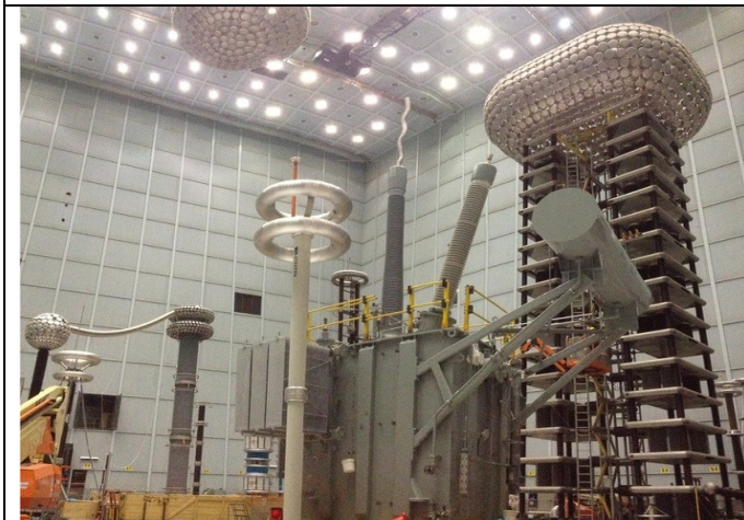
PD0537: Supply of Power Transformers, AC Substations at Churchill Falls-Factory Testing
