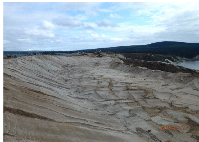
CH0008: Construction of North Spur Stabilization Works- Construction of temporary road on downstream slope
