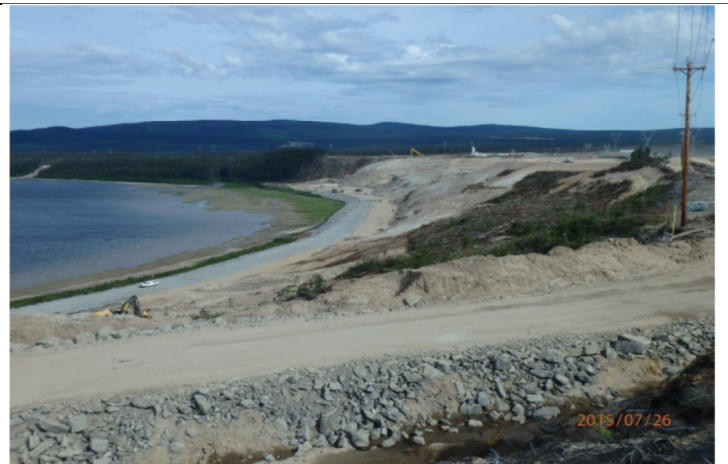
CH0008: Construction of North Spur Stabilization Works-CB cut-off wall temporary work platform
