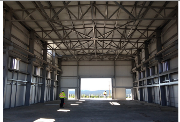
CD0502: Churchill Falls Switchyard
