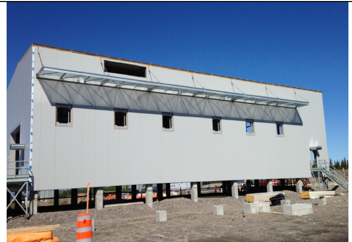
CD0502: Churchill Falls Switchyard
