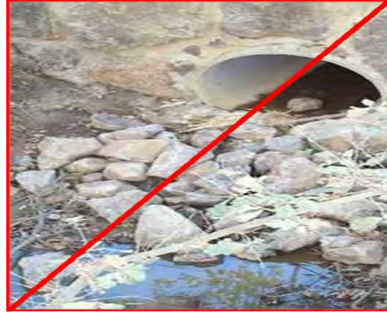
Figure 5-32: Incorrect Construction of Rock Energy Dissipaters
