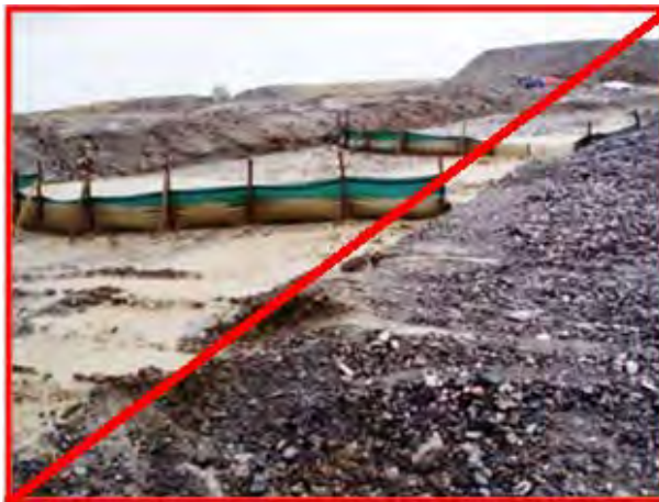
Figure 5-36: Examples of poorly installed silt fences
