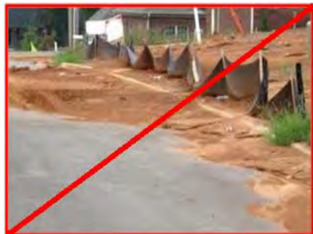
Figure 5-37: Examples of poorly installed silt fences
