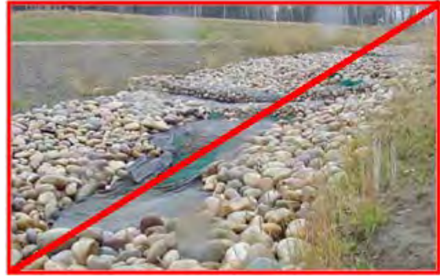
Figure 5-28: Photograph of failed Rip Rap Protection
