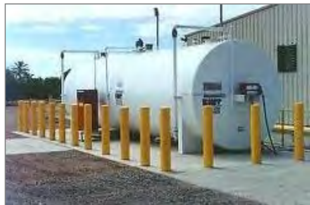
Figure 5-6: Fuel storage on concrete pad
