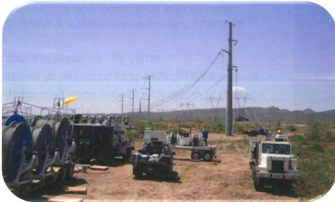
Full compliment of multi-bundled conductor and OPGW installation equipment, including wire pullers, tensioners, and stringing equipment.
