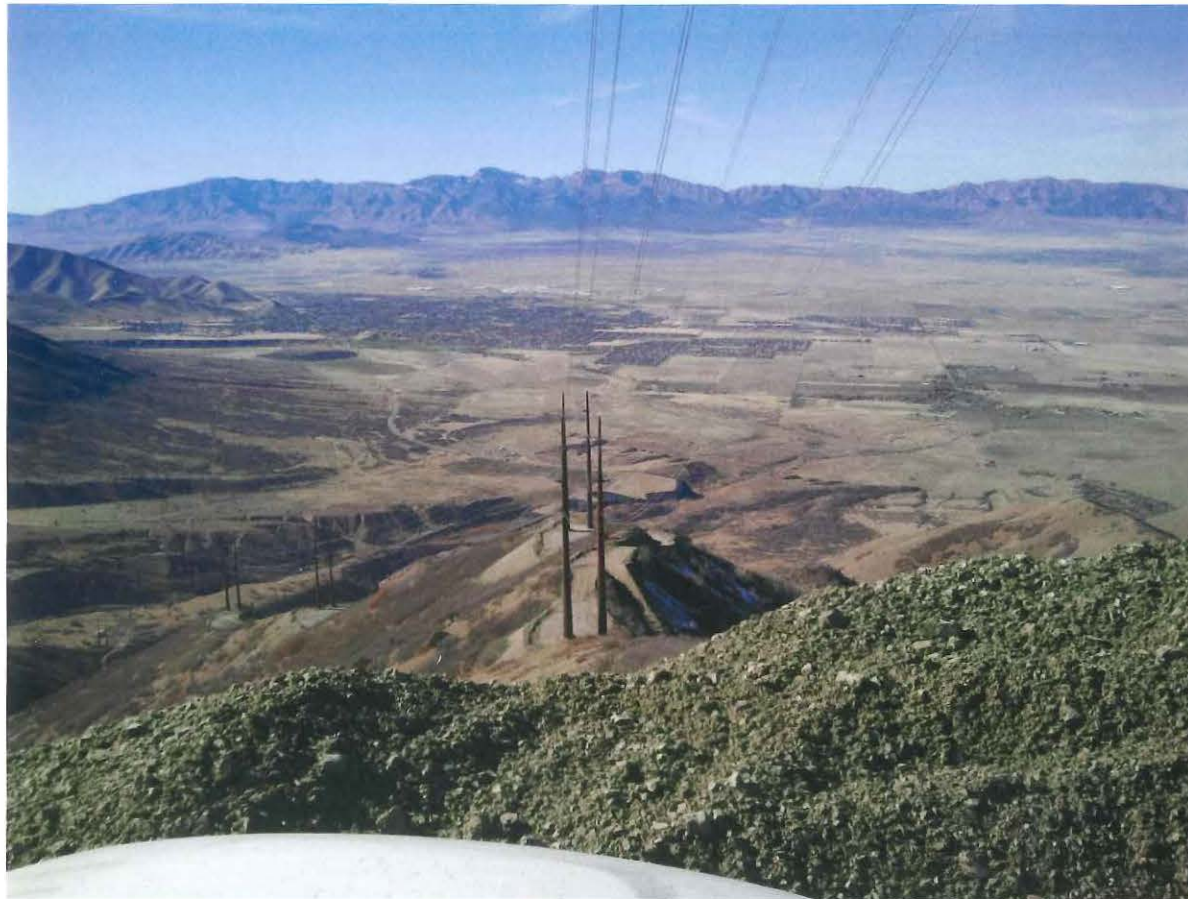
345kV steel erection on the 110 Mile EPC Mona to Oquirrh Transmission Line in Utah
