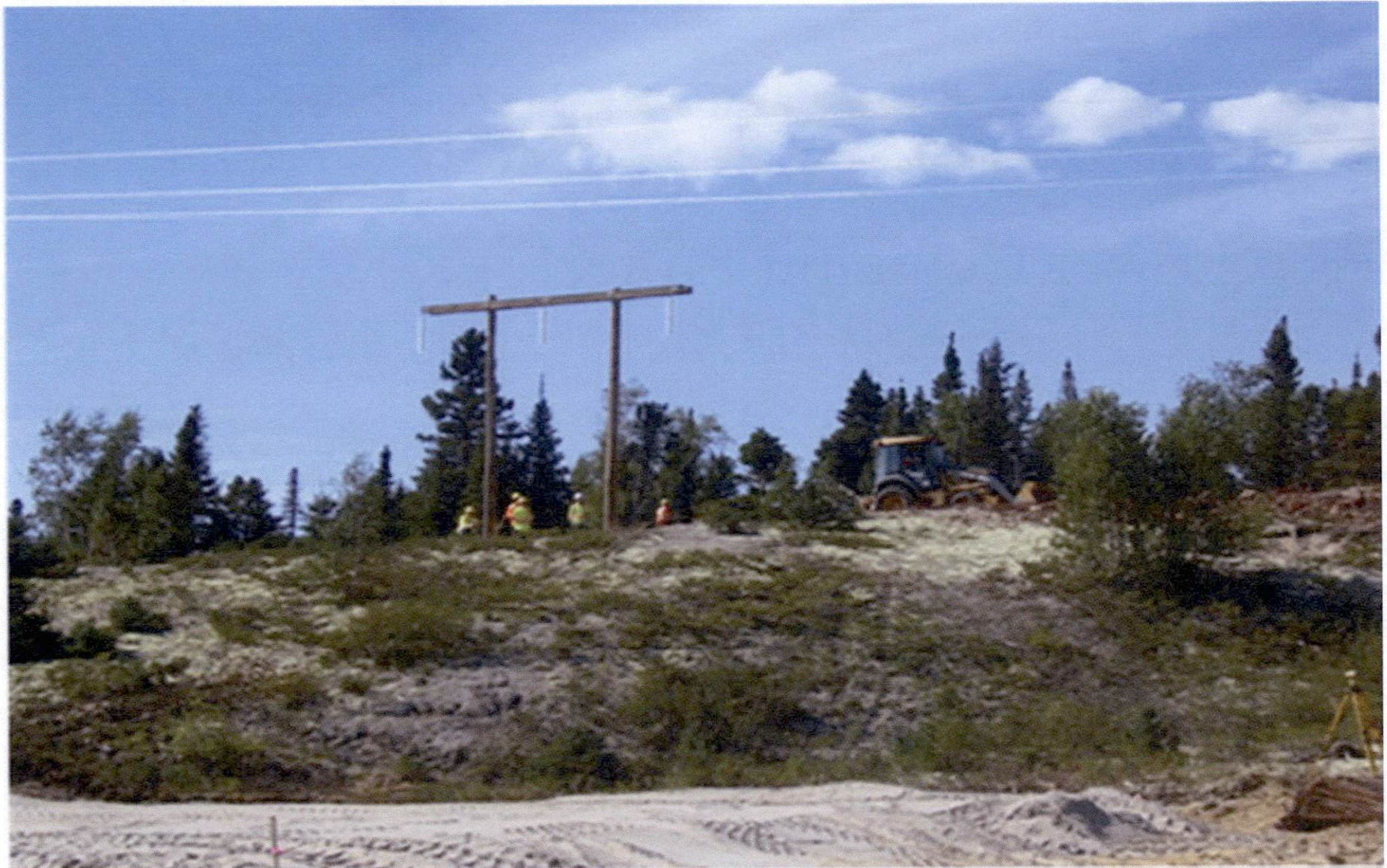
GJ Cahill Personnel Working Near 138kv line
