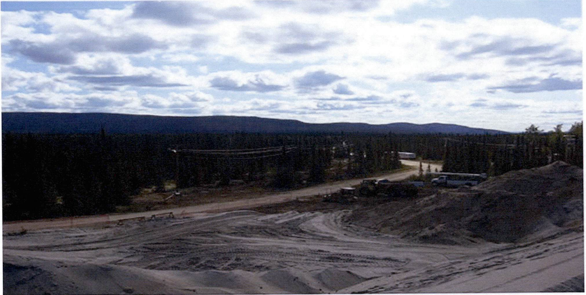
View from The Tap Station Looking Southwest On The 25kv Line
