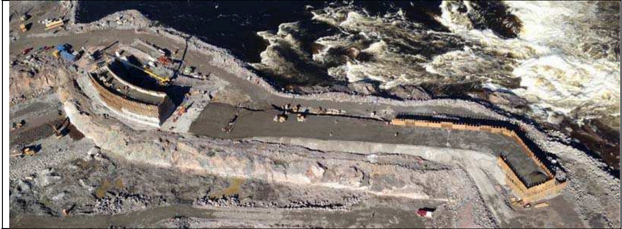
Photo 7: Aerial view of the RCC cofferdam (Aerial photograph taken by Nalcor on September 28, 2013)
