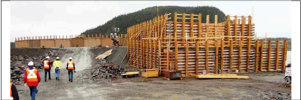
Photo 8: Formwork for downstream end of the RCC cofferdam. Note sloped RCC material in the section immediacy upstream of the formwork. (09/25/2013)
