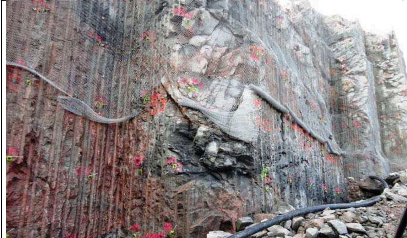
Photo 19: Powerhouse south wall. Contact between pink granitic intrusion and grey gneiss. Note excellent wall contours and the localized fallouts at the outside corner in the centre of the picture. Rock bolts are visible. Note the temporary wire mesh cover to ensure safety against rock falls. (09/26/2013)
