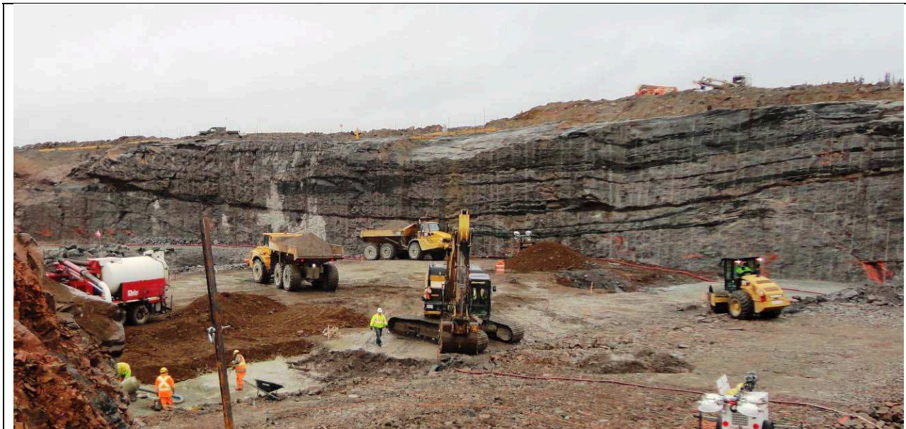
Photo 20: Spillway. South wall in in background showing the control drill half barrels and gently curved foliation and amphibolite layers. Foreground shows ongoing fill placement work for the upstream cofferdam. (09/25/2013)
