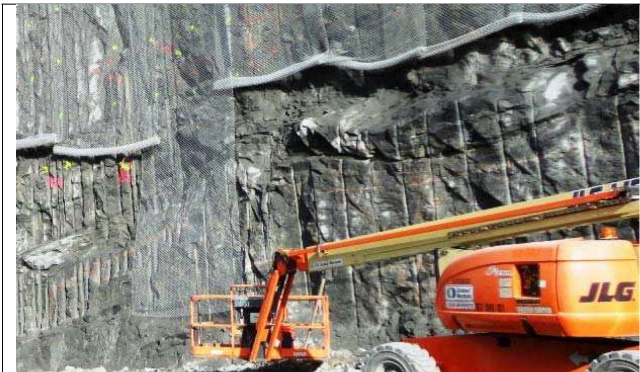
Photo 16: Powerhouse north wall. Line drilled face on left half and presplit face on right half of photo. Note the block sliding overbreak above the crane on the right. This sliding occurred along a moderately inclined S1 foliation plane. . Also note the wire mesh cover draped over the rock face to ensure safety against rock falls. (09/26/2013)
