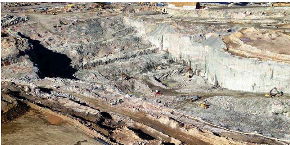
Photo 14: Powerhouse excavation. View looking upstream showing ongoing excavation and the north wall (Aerial photograph taken by Nalcor on September 28, 2013)
