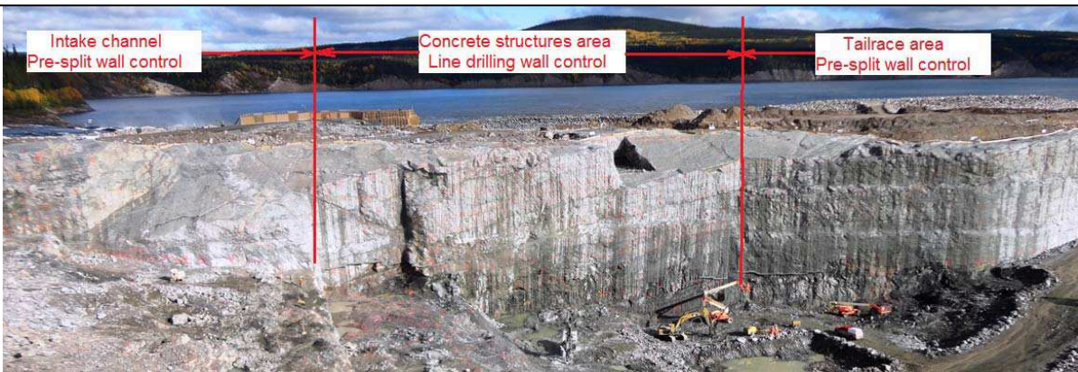
Photo 13: Powerhouse and tailrace excavation north wall. Areas of line drilling and pre-split wall control are shown. Note the 0.75m die berms at 10 m vertical spacing in the presplit area. On the right side of the photograph. (09/26/2013)
