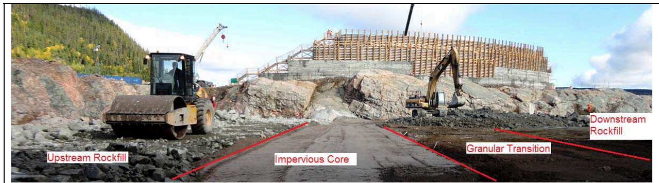
Photo 11: Zoning of upstream cofferdam No. 1. View looking north towards the river. Note upstream end of the RCC cofferdam in the background. (09/26/2013)
