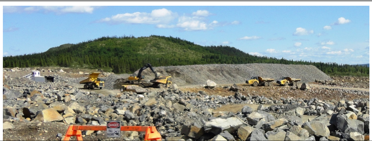
Photo 10.1: Churchill Falls New 315 kV substation and switchyard. Loading processed fill. Note stockpile of processed fill in the background and blasted rock in foreground. (July 18, 2014)
