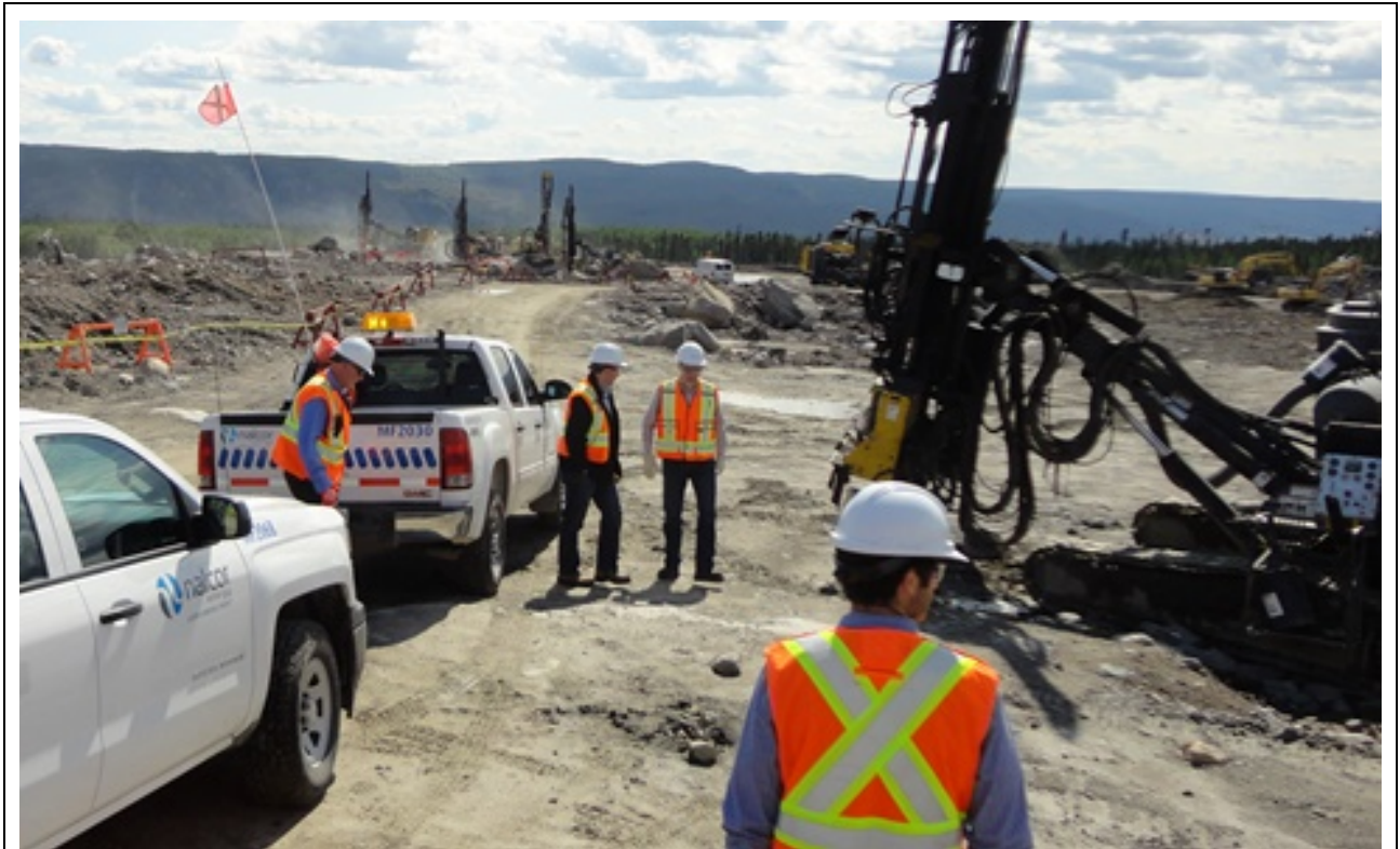
Photo 10.2: Churchill Falls New 315 kV substation and switchyard. Blast hole drilling in bedrock. (July 18, 2014)
