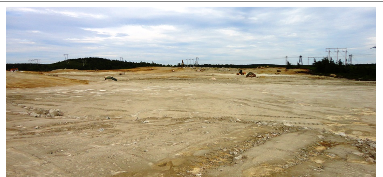
Photo 1.2: Soldier's Pond site; placing compacted fill to grade at east half of the site. (July 14, 2014)
