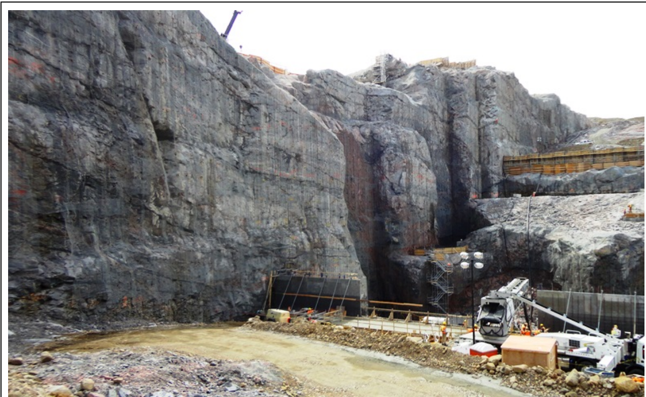
Photo 6.5: Right rock slope at powerhouse. Note the excellent quality of the line drilled excavated rock walls. A single fallout of a small wedges has caused a very localized overbreak feature. (July 17, 2014)
