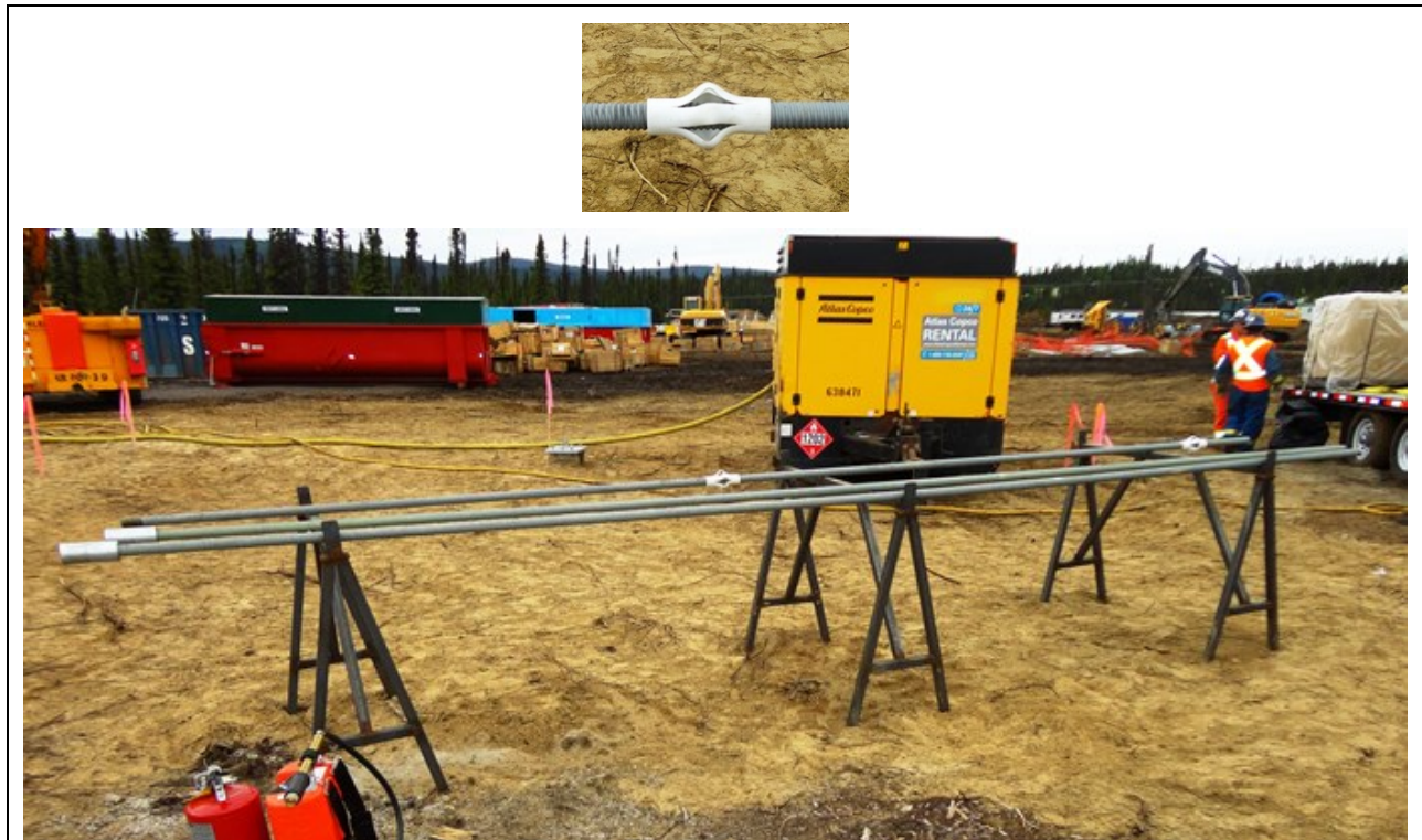
Photo 8.5: Transmission Tower Erection and Foundations. Ground anchorage assembly, complete with couplers. Inset shows a typical plastic centralizer (July 16, 2014)
