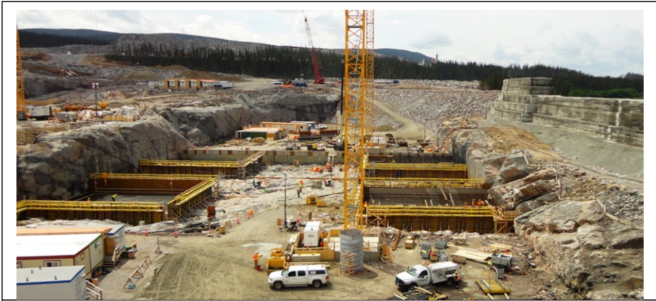
Photo 6.2: Spillway base slab. Formwork for first four blocks of the base slab. (July 17, 2014)
