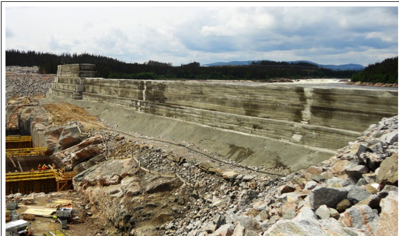
Photo 6.3: RCC cofferdam above the spillway left wall. Note the localized blasting overbreak of the spillway rock slope caused by block sliding along pervasive foliation planes. (July 17, 2014)
