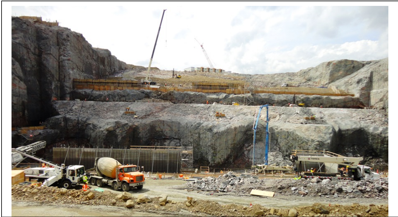
Photo 6.6: Powerhouse excavation, view looking upstream. The excellent control blasting results are visible in the rock noses between the unit cut-outs. (July 16, 2014)
