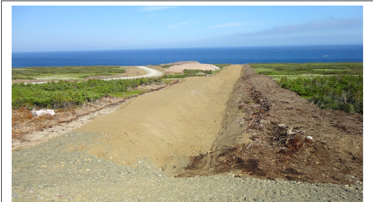
Photo 2.7: Forteau Directional Drilling. Excavated trench for the three cables between the transition compound and the drilling site. (July 15, 2014)
