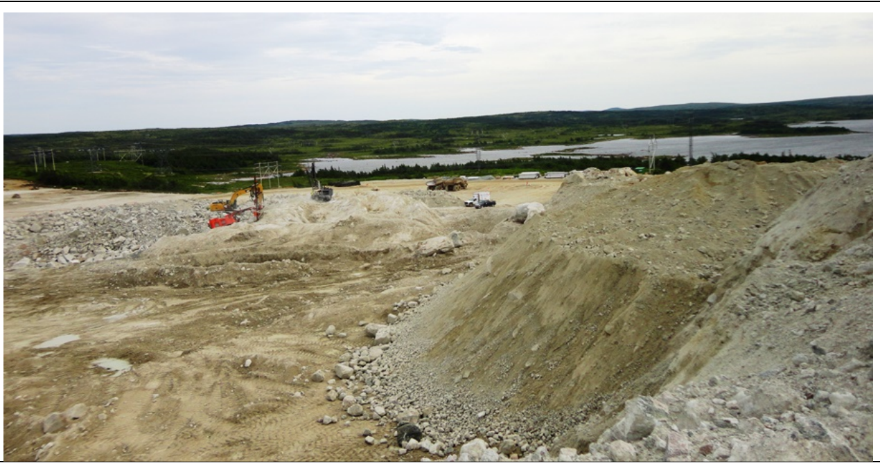
Photo 1.1: Soldier's Pond site; excavation work at the west end of the site. (July 14, 2014)
