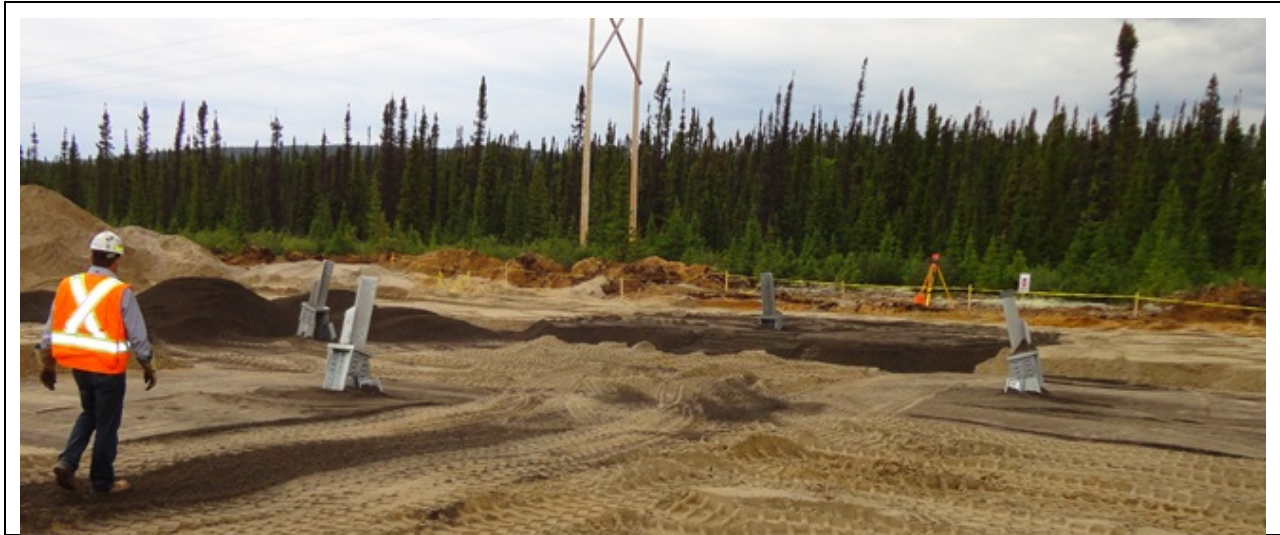
Photo 8.4: Transmission Tower Erection and Foundations. Tower footings installed and backfilled (four legged tower) (July 16, 2014)
