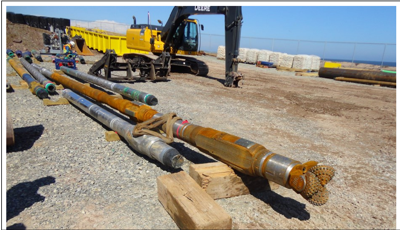
Photo 2.5: Forteau Directional Drilling. Drill bit and lower non-magnetic drill string components. (July 15, 2014)
