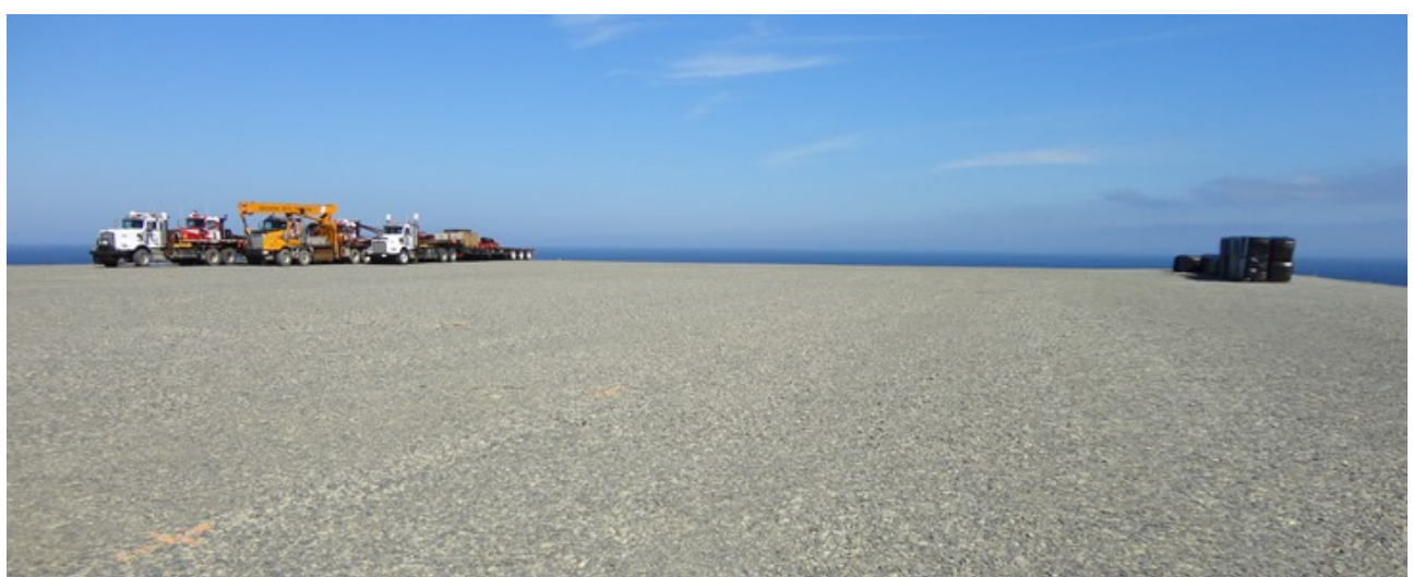
Photo 2.6: Forteau Directional Drilling. Graded fill at future transition compound site above the drilling site. (July 15, 2014)
