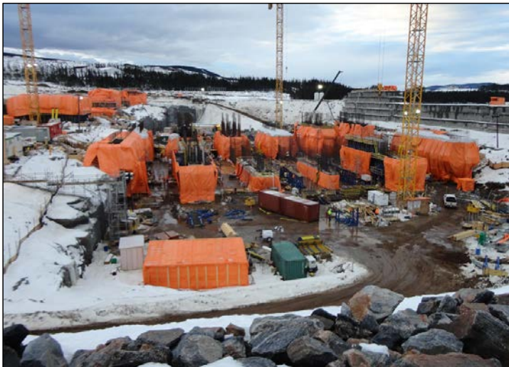
Photo 7.2: Spillway; view looking upstream towards the piers. RCC cofferdam is visible on the right side and the orange tarp covered transition dam is on the left. (November 25, 2014)
