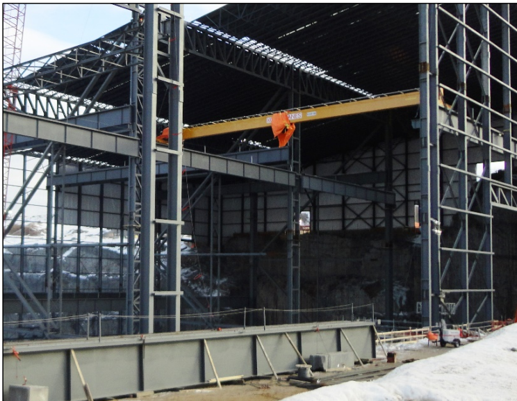
Photo 8.12: Powerhouse ICS. Beam crane above Unit 2. (November 26, 2014)
