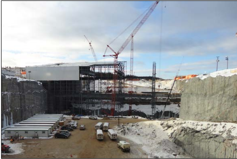
Photo 8.1: Powerhouse ICS looking upstream. Units 1 and 2 framework erection and first roof covering are substantially complete and almost half of the wall cladding has been erected. At Unit 3 the framework and first roof covering are substantially complete but no progress has been made on the wall cladding. No progress with the ICS in the area of Unit 4. . (November 26, 2014.)
