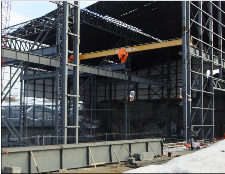
Photo 8.12: Powerhouse ICS. Beam crane above Unit 2. (November 26, 2014)
