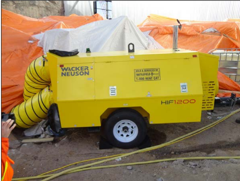
Photo 9.5: Wacker Neuson heating unit used for heating the works in the north service bay. (November 26, 2014)
