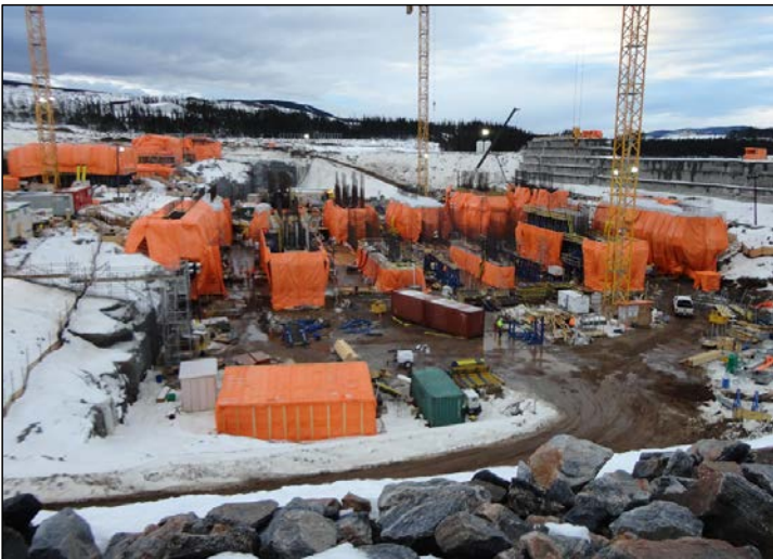
Photo 7.2: Spillway; view looking upstream towards the piers. RCC cofferdam is visible on the right side and the orange tarp covered transition dam is on the left. (November 25, 2014)
