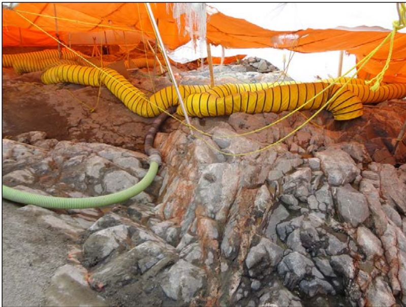
Photo 9.4: Powerhouse north service bay foundation. Cleaned surface in blocky granitic gneiss. (November 26, 2014)
