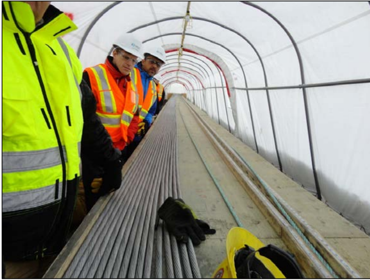
Photo 2.1: Laydown and preparation of guy cables for HV ac AC transmission towers. (November 25, 2014)
