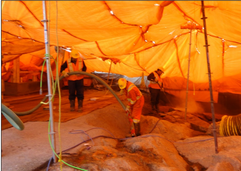
Photo 9.3: Powerhouse north service bay foundation. Cleaning the rock surface with an air vacuum and water jet. (November 26, 2014)
