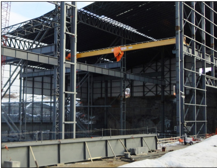
Photo 8.12: Powerhouse ICS. Beam crane above Unit 2. (November 26, 2014)
