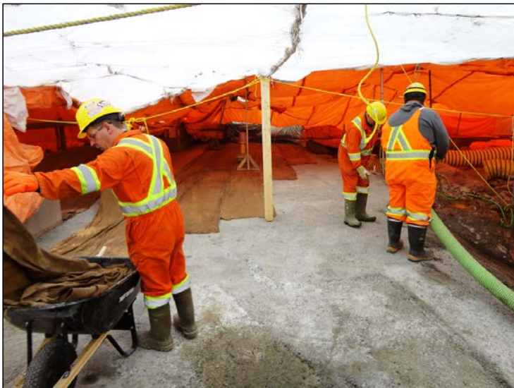
Photo 9.2: Powerhouse north service bay foundation. Note wetted burlap mats being placed on the surface of the base slab. (November 26, 2014)
