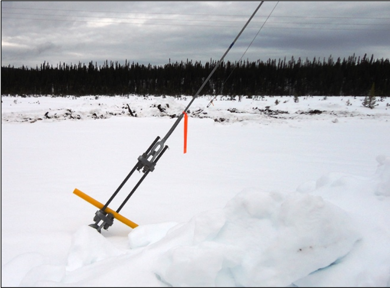
Photo 4.3: Lower connection of guy cable on single footing transmission tower
