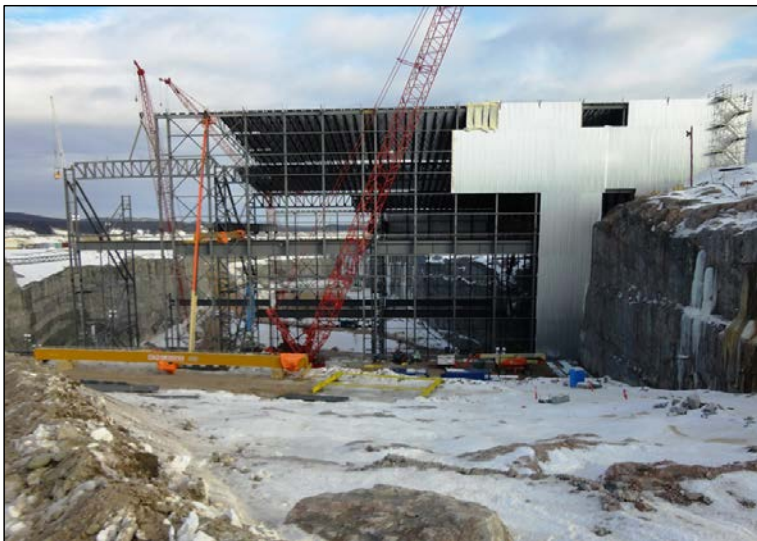
Photo 8.2: Powerhouse ICS looking downstream. Framework and cladding in Units 1, 2 and 3 can be seen. (November 26, 2014.)
