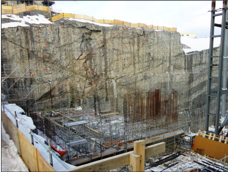
Photo 8.11 Powerhouse, Bay 4. Permanent concrete at base of intake structure at Bay 4. This is the only permanent concrete in the powerhouse/intake structures. (November 26, 2014)
