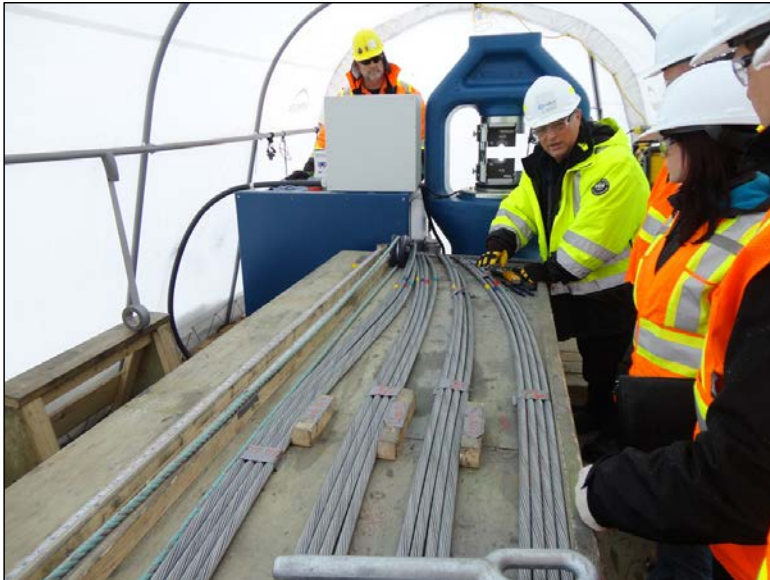
Photo 2.2: Laydown and preparation of guy cables for HV ac AC transmission towers. (November 25, 2014)
