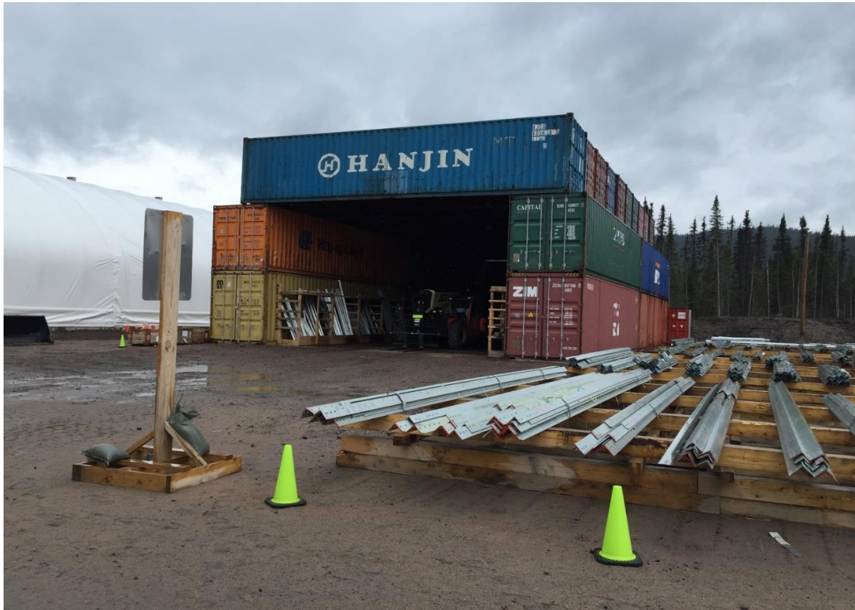
Photo 4.8 Transmission lines Marshaling Yard (July 8, 2015).
