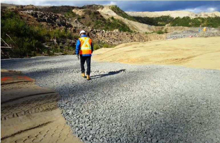
Photo 3.22: Downstream slope; finger drain near the toe of the slope. The finger drain filters extend is oriented across the slope.
