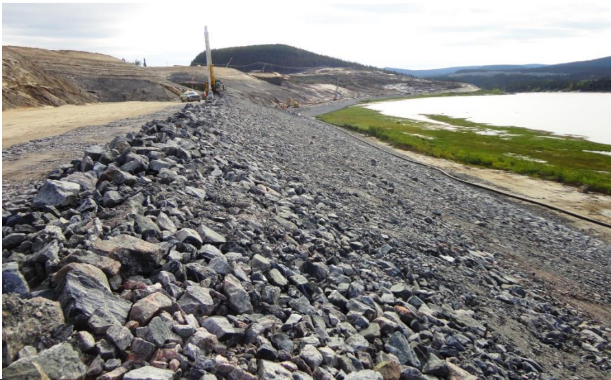
Photo 3.6: Upstream slope - Upstream rip rap blanket as viewed looking south from the el 24 m level.
