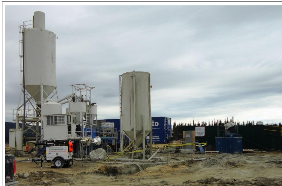
Photo 3.18: Plant for mixing the cement bentonite slurry concrete of the cut-off wall.
