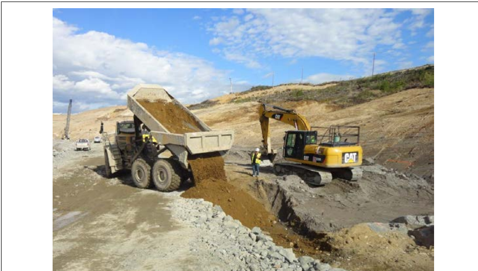
Photo 3.10: Upstream slope. Placing sand filter granular transition for the impervious blanket at the south end of the upstream
