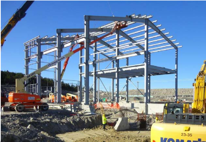
Photo 2.5: Synchronous condenser building
