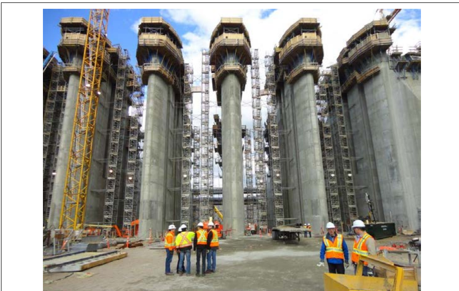
Photo 4.4: Spillway looking towards downstream. From right to left, Bays 1, 2, 3, and 4 are visible.
