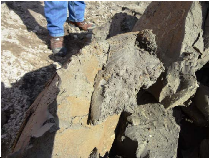
Photo 3.15: Upstream slope- Excavated greenish grey "lower clay" from the south end of the cut-off. The lower clay is a firm, plastic clay with low sensitivity. This material is at approximate el -5.14 to 5m along most of the upstream face and is the impervious material that the base of the cut-off wall is seated in.
