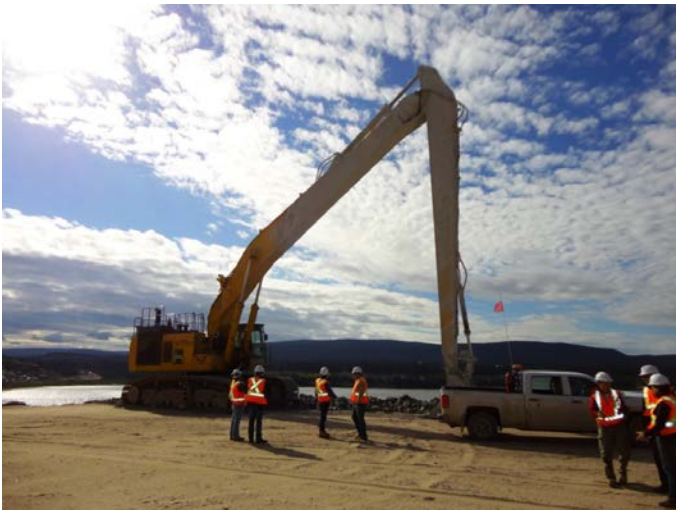
Photo 3.16: Upstream slope- Long stick backhoe excavator used to excavate most of the upstream slope cut-off wall to depths of about 15m
