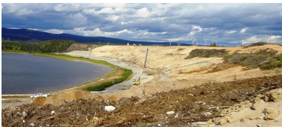
Photo 3.1: Upstream slope - Overall view of the upstream slope of the North Spur, showing the excavated slope and the cut-off wall line along el 20m the toe berm. View is looking towards the north. The el 10m berm is visible along the toe of the excavated and trimmed slope. In the back ground, the el 24m and el28 m fill intermediate placement berms can be seen.
