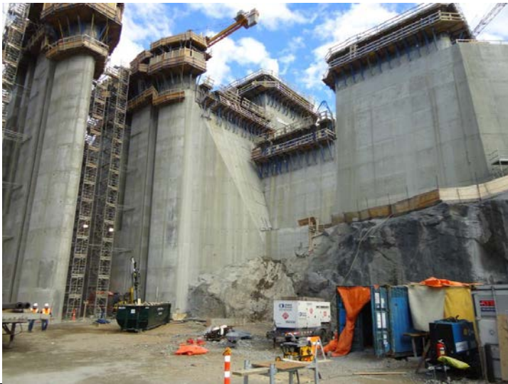
Photo 4.5: Spillway, view of upstream right corner. The left end of the concrete transition dam is visible in the upper central area of the photograph.
