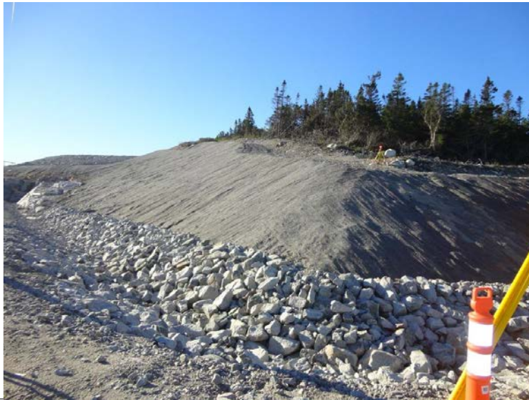
Photo 2.2: Cut slope in glacial moraine at west end of the facility. The upper slope is covered by porous coconut/wire mesh slope protection. No seeding has been done and this mat has deteriorated in many places. Rip rap layer in place on the lower slope.
