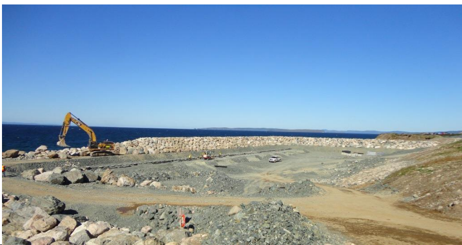
Photo 1.1: Dowden's Point dyke. Note the line of electrode wells at the base of the dyke.
