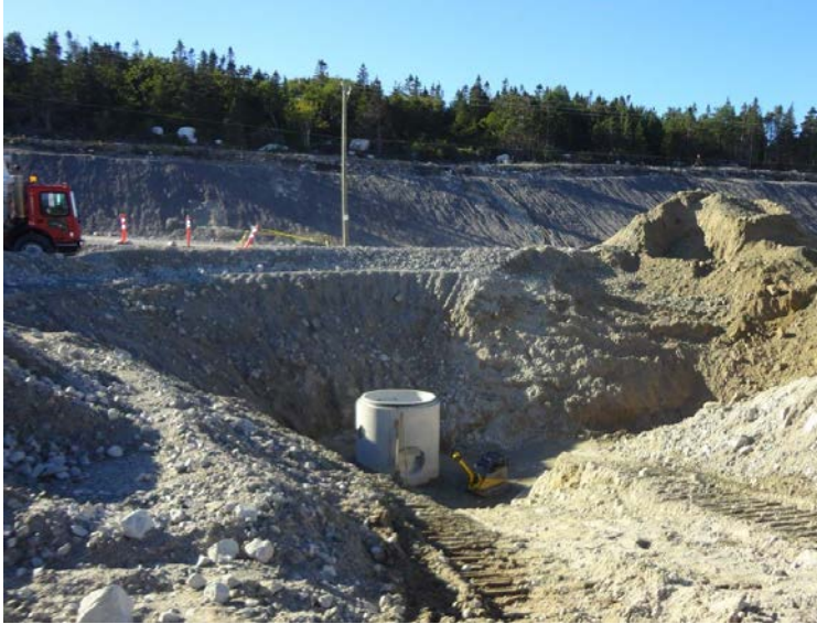
Photo 2.7: Manhole for the oil water separator for the synchronous condenser facility at the west side of the site.
