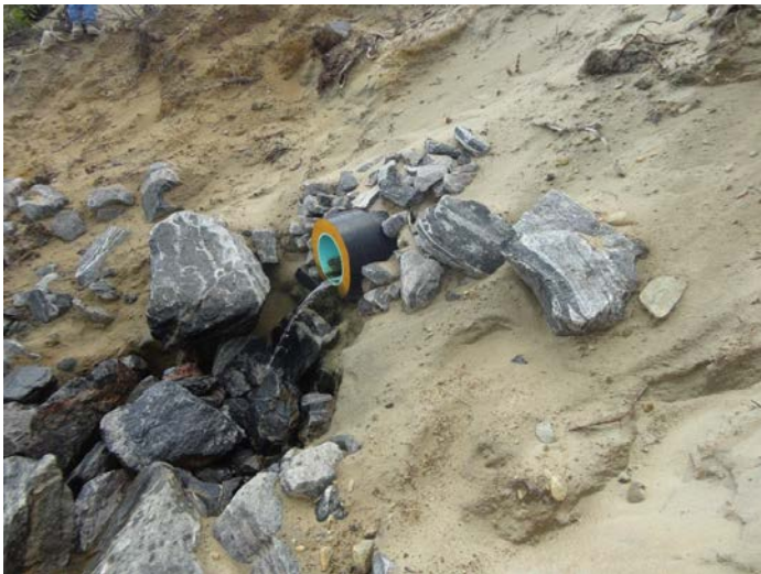
Photo 3.26: Pumped wells outlet pipe in the ravine downstream of the kettle lakes.
