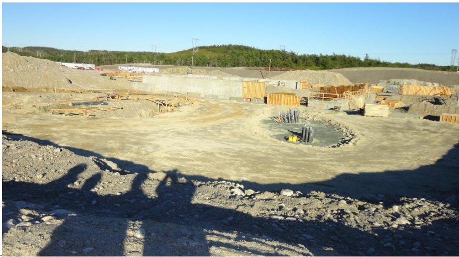
Photo 2.10: DC transformer foundation southern area
