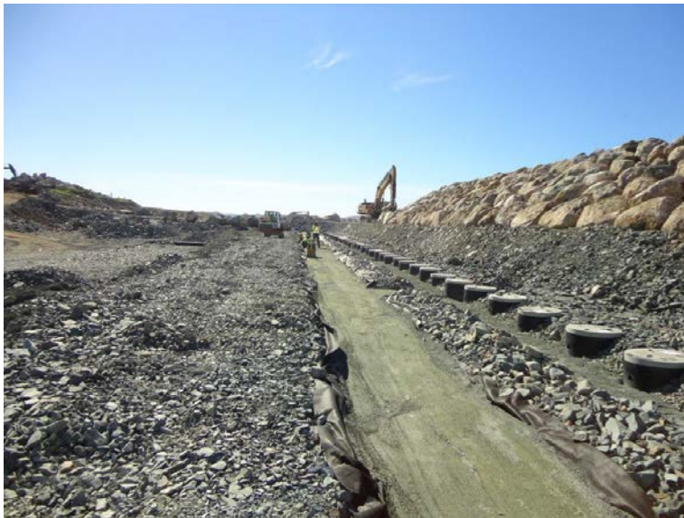
Photo 1.4: Looking west along the line of electrode wells and the conductor bedding trench.
