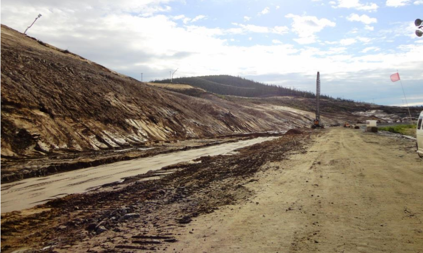
Photo 3.7: Upstream slope - Upstream toe at el 20m; top of cutoff wall, covered by a compacted till is visible running from the lower left corner of the photograph. View is looking south.
