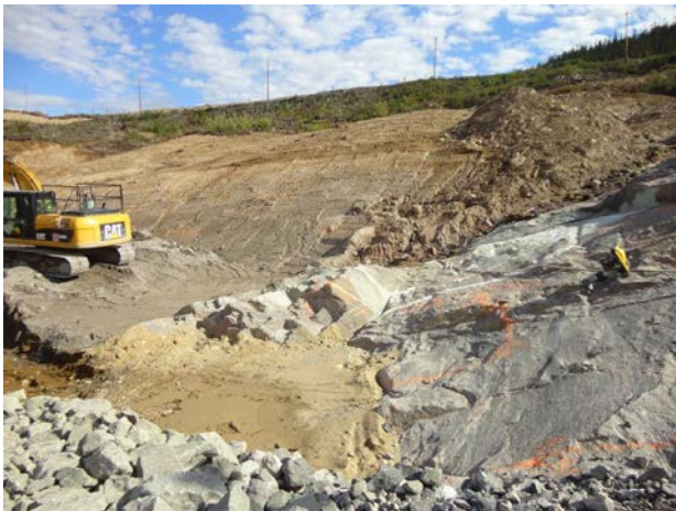
Photo 3.12: Upstream slope. Placement of fine grained till and sand filter granular transition on the bedrock outcrop at the south end of the upstream slope.
