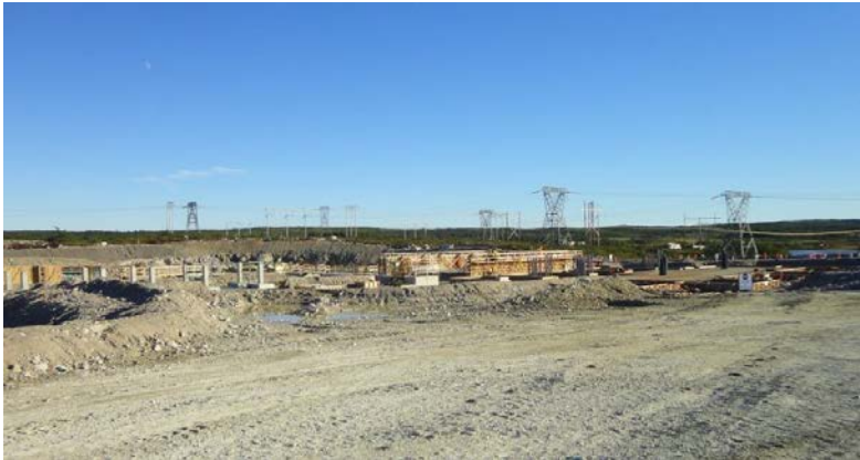
Photo 2.1: AC/DC converter site
