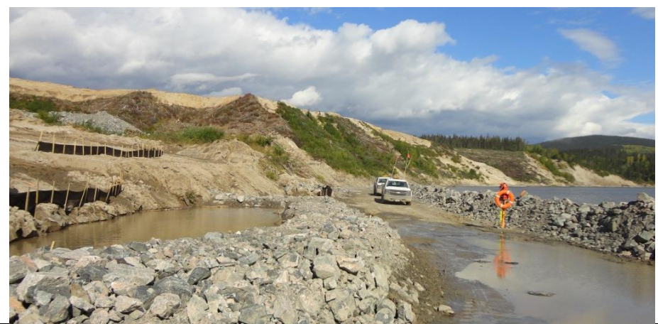
Photo 3.20: Downstream slope; water collection and silt fences at toe of slope. Some slope trimming has been done in the lower slope. Some debris from the 1978 slide are visible in the background (upslope from the white pick-up trucks).
