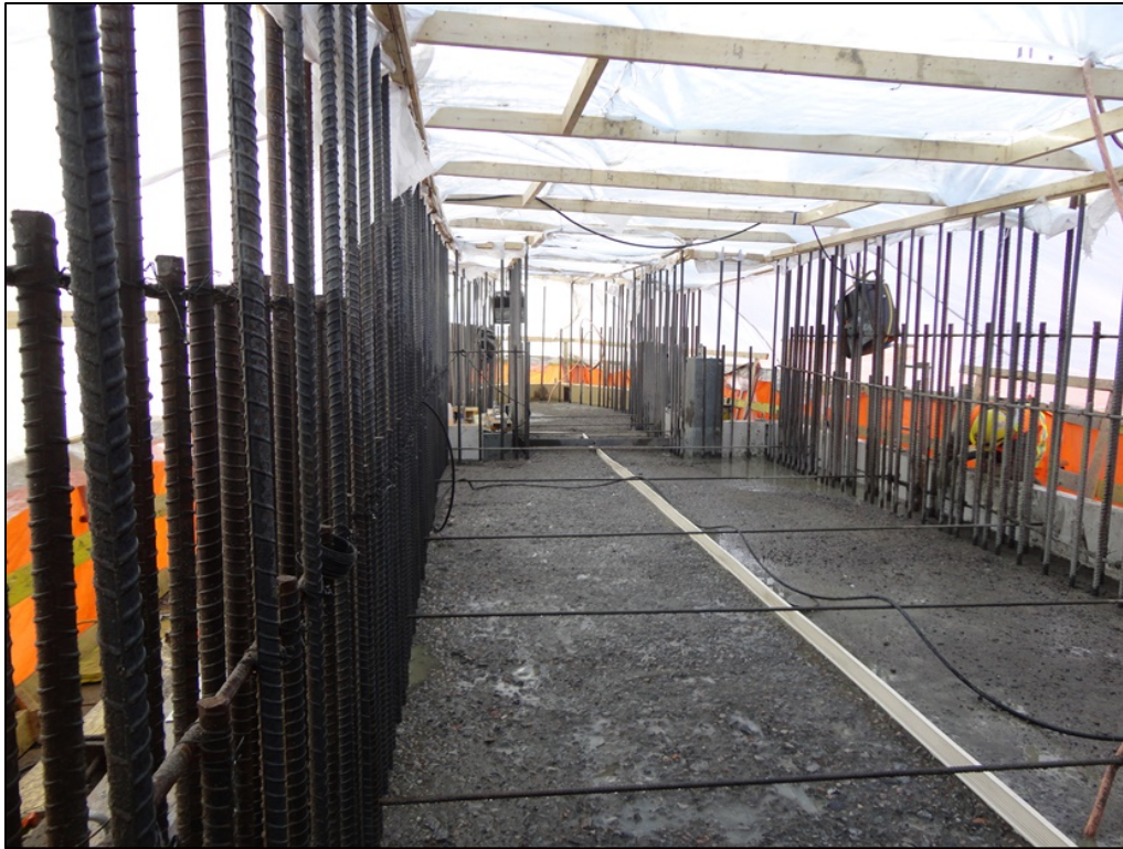
Photo 7.9: Current top of Pier 3 looking upstream. The concrete was green cut on the previous day and was currently being washed at the time of the photograph. Note the cut-out for the upstream stop logs in the background and the white water stop running down the centerline of the pier. (November 26, 2014)
