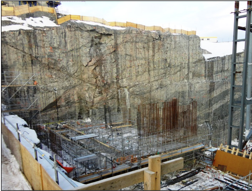
Photo 8.11 Powerhouse, Bay 4. Permanent concrete at base of intake structure at Bay 4. This is the only permanent concrete in the powerhouse/intake structures. (November 26, 2014)
