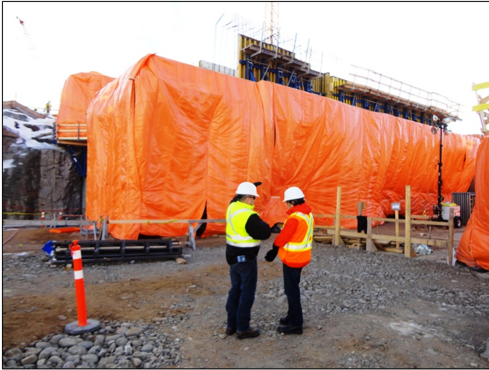
Photo 7.3: Right side of the spillway. Transition dam is visible at the top of the photograph. (November 26, 2014)
