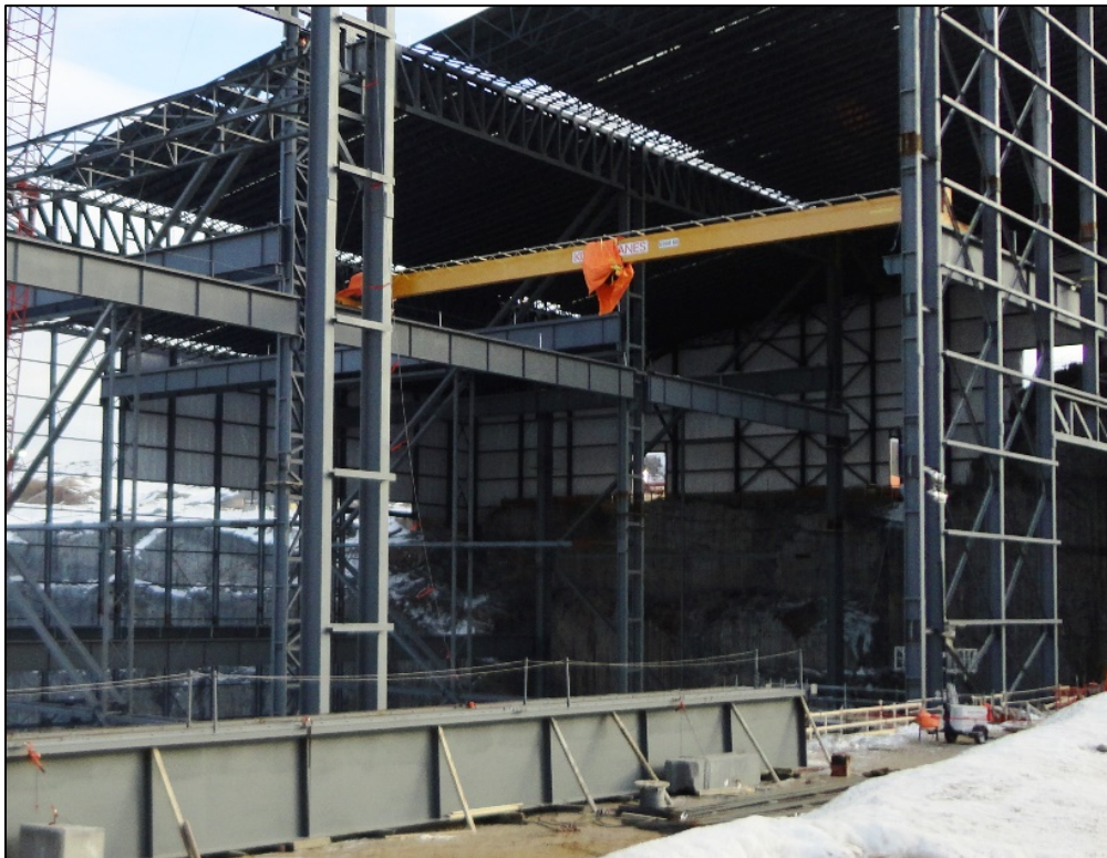
Photo 8.12: Powerhouse ICS. Beam crane above Unit 2. (November 26, 2014)
