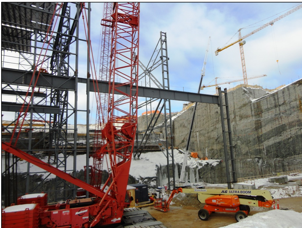
Photo 8.4: View looking upstream at the initial ICS framework erection over Unit 3 (November 26, 2014)
