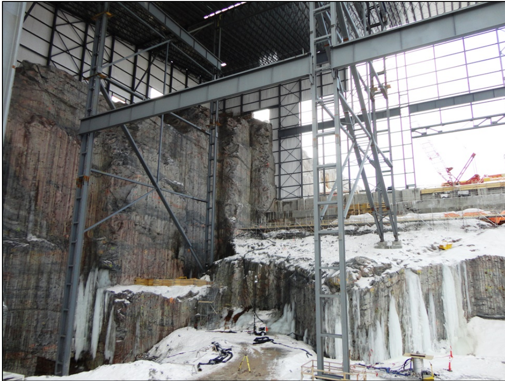
Photo 8.9: View looking upstream at the interior of the ICS over Bays 1 and 2. (November 26, 2014)
