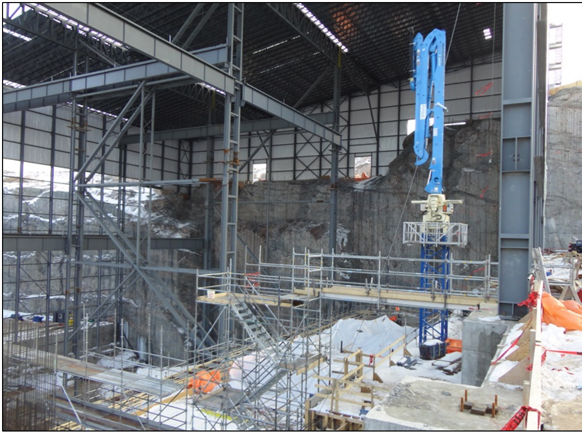
Photo 8.13: Putzmeister concrete pump on a fixed swivel mounting between Bays 2 and 3 in the Powerhouse. Additional pumps will be installed throughout the powerhouse to make sure that all areas can be reached. (November 26, 2014)
