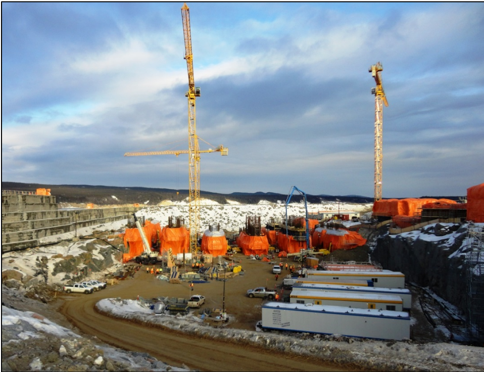
Photo 7.1: Spillway; view looking downstream towards the piers. RCC cofferdam is visible on the left side and the orange tarp covered transition dam is on the right. (November 26, 2014)
