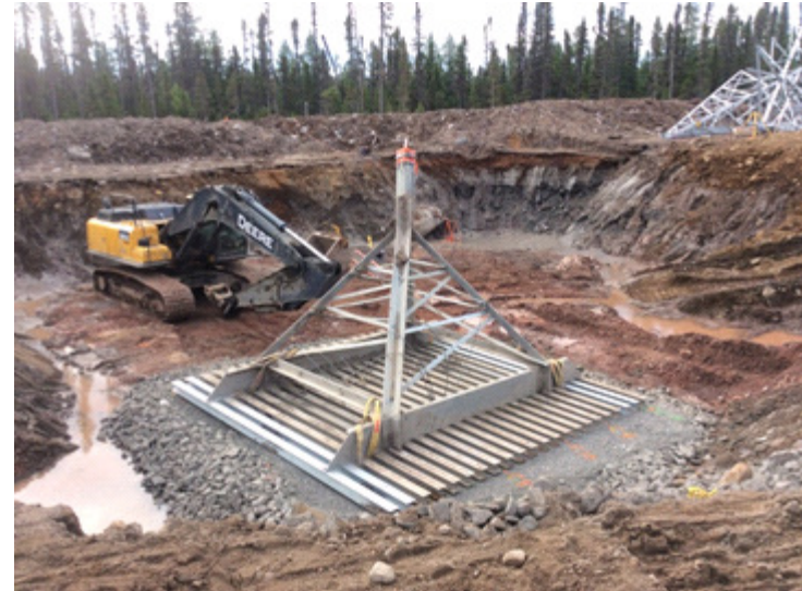
S1-70, Leg A, Grillage Placement on prepared founding base with groundwater control.
