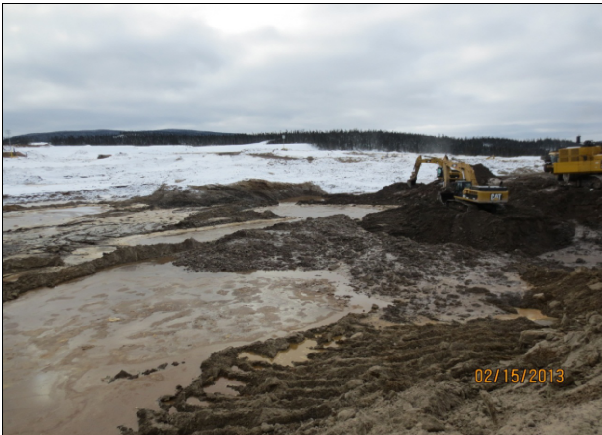
Figure 41: February 15, 2013 overburden excavation operations. The Contract and Company's Geotechnical Report did not represent swampy conditions such as these. Conditions such as these significantly affected IKC-ONE's overburden excavation means and methods.
