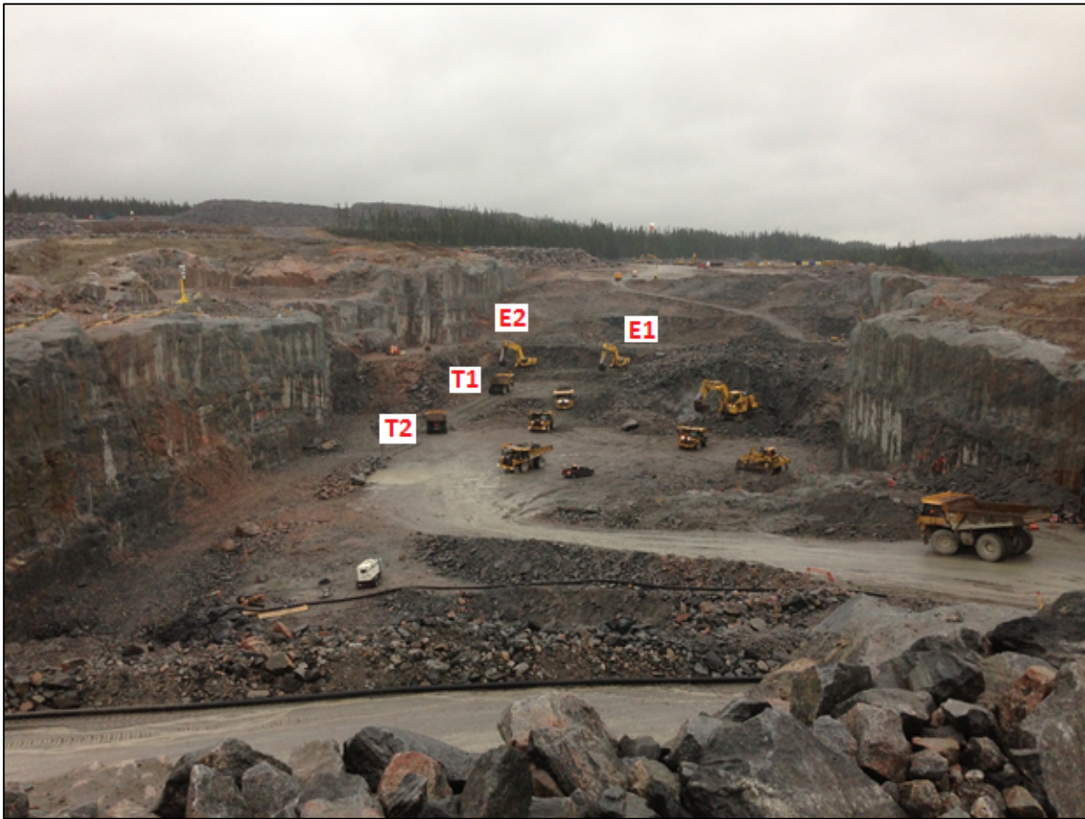
Figure 52: IKC-ONE's rock excavation productivity and production has been effected by acceleration. The above figure depicts a scenario where two pieces of equipment are ready to produce (E2 and T2), but must wait for two other pieces of equipment (E1 and T1) to produce. Company's direction to accelerate has forced IKC-ONE to execute many operations similar to these, which have resulted in inefficiencies.
