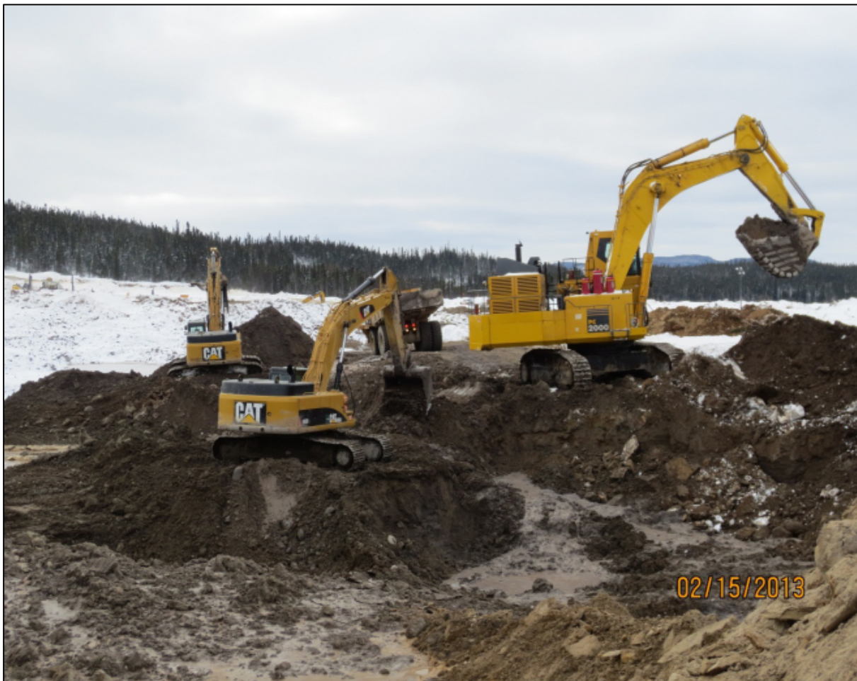
Figure 42: IKC-ONE's February 15, 2013 overburden excavation operations (representing a typical condition). IKC-ONE performed most of its overburden excavation operations in wet conditions such as these. Note that IKC-ONE is using an unplanned Cat 336 and an unplanned Cat 345 to cast wet material to the Komatsu PC 2000 in order to load trucks effectively.
