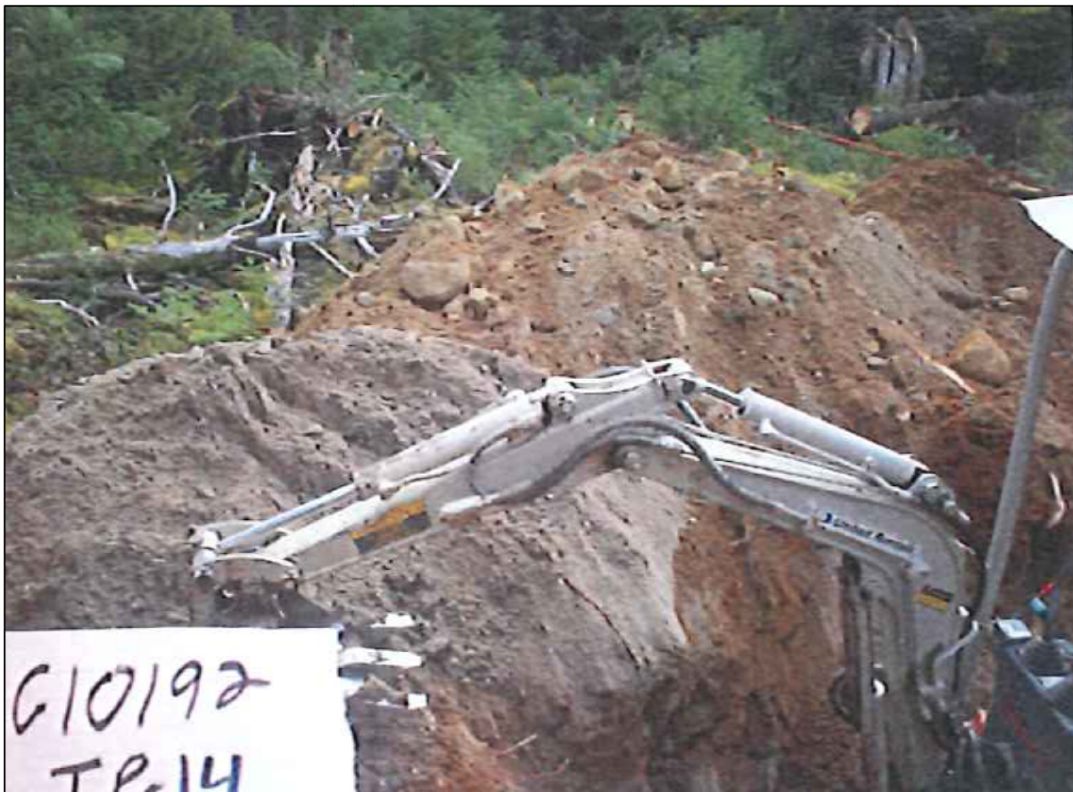
Figure 19: Sample test pit represented in the project Geotechnical Report. The test pit reports states "some water infiltration observed", however, note that the test pit and the test pit spoil pile is dry.
