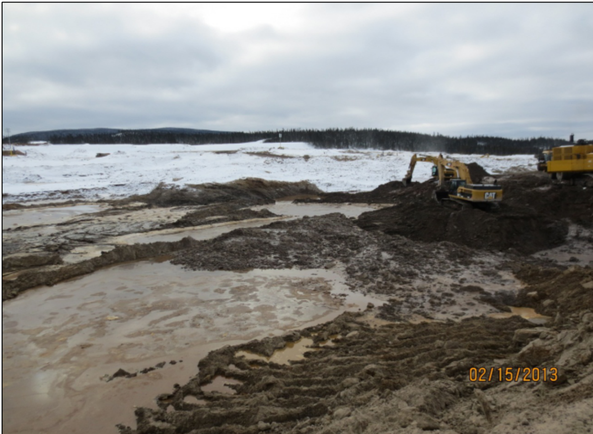
Figure 34: February 15, 2013 overburden excavation operations. As shown above, IKC-ONE had to utilize extra small size excavators, mid-size excavators, pumps, and pumping crews to perform the work.
