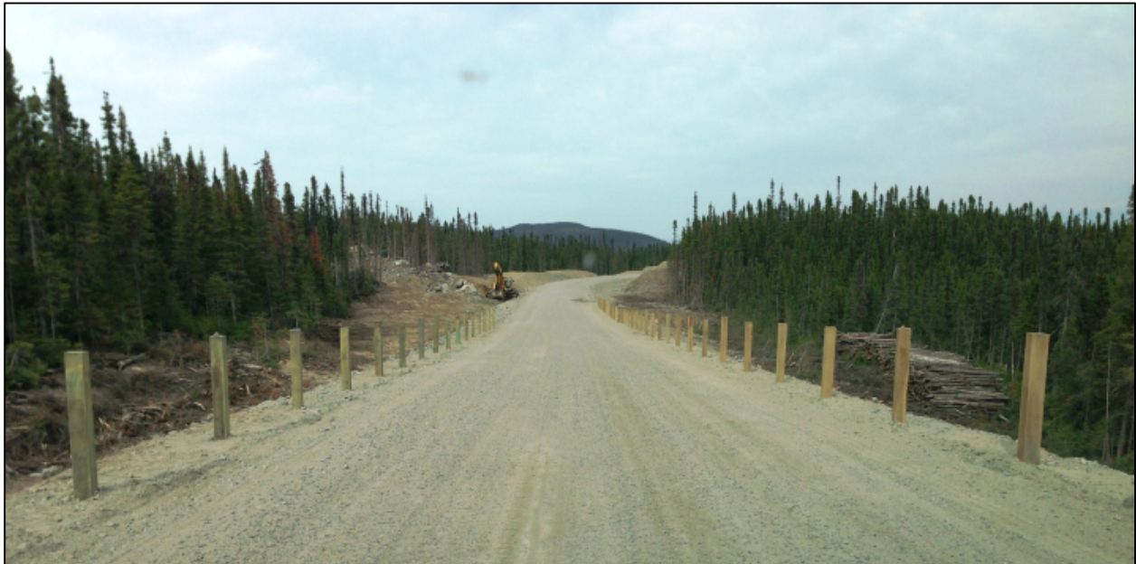
Figure 13: July 27, 2013. Lower Churchill Site Access Road complete (except for the guardrails). The condition of the site access road depicted here allows for safe and comfortable travel at an average speed of 60-80 km/hr.
