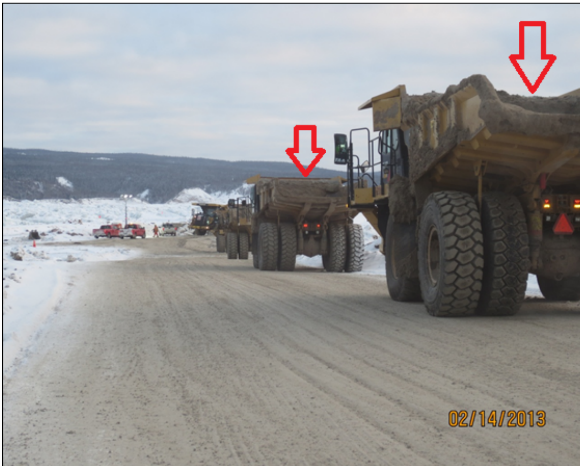
Figure 43: IKC-ONE's February 14, 2013 overburden excavation operation. Note that IKC-ONE's haul trucks are returning from a dump with mud frozen and stuck in their boxes. This typical condition resulted in lower “load factors” (less material could be loaded per each haul), and consequently reduced productivity.
