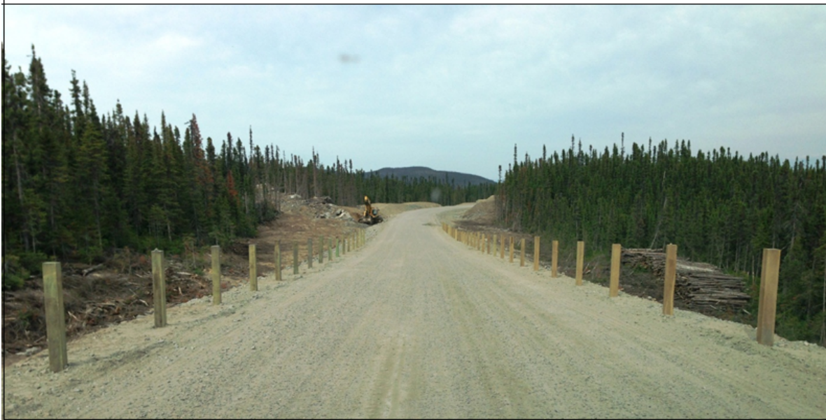
Figure 30: Top image shows condition of the Site Access Road on June 16, 2013. Bottom image shows the condition of Site Access Road on July 9, 2013. The bottom image depicts what Company promised and what the Contract warranted.
