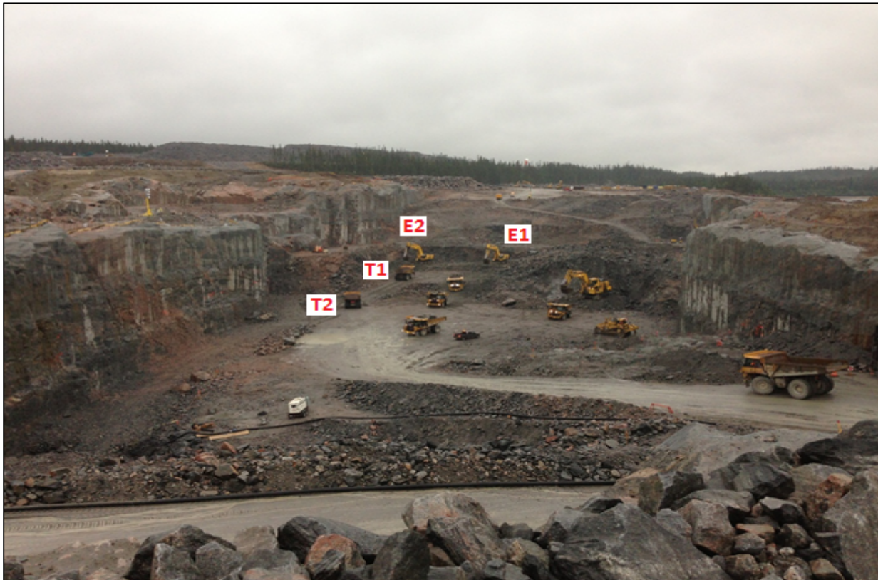
Figure 45: Rock excavation operations on August 14, 2013. IKC-ONE continues to accelerate to complete the project on October 25, 2013. IKC-ONE did not plan to have three mid-size/large-size excavators and one bulldozer in its rock excavation equipment spread. Additional equipment is designated as E2 and T2.
