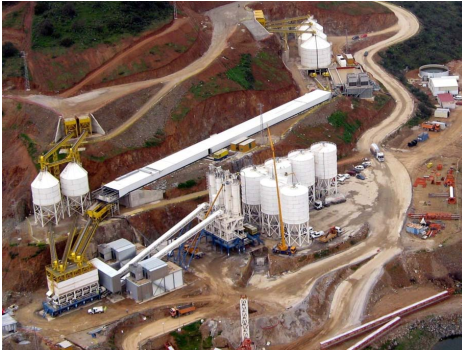
Figure 5: Concrete Plant (La Breña II Dam, Spain)
