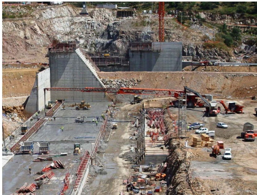
Figure 34: Creter-crane Type Machine, fed by Agitator Trucks, being used for RCC Dam Construction
