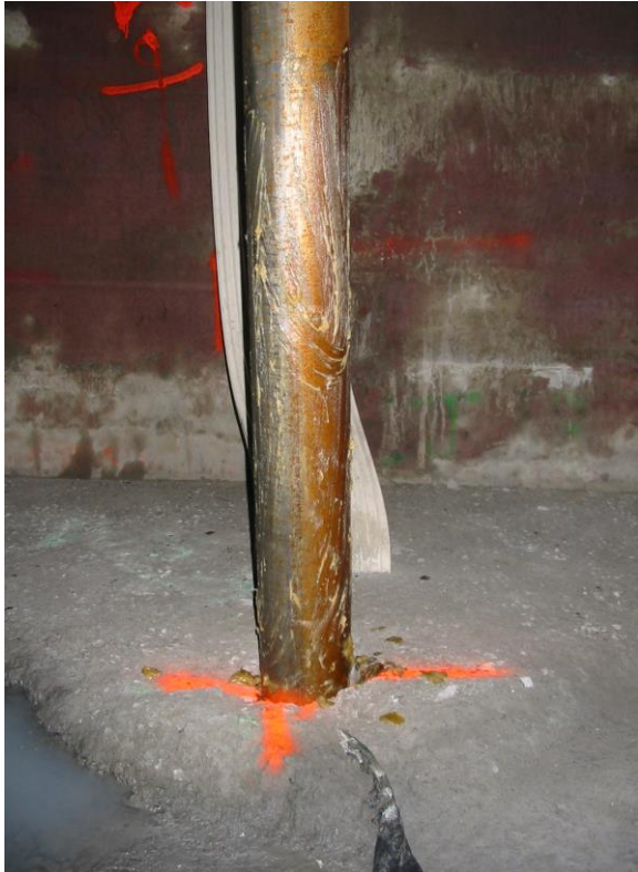
Typical waterstop and rear drain detail surrounded by either conventional concrete or grout-enriched RCC
