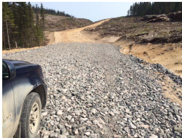
Figure 3-5: Crushed Rock Road Base Spread over-top of what appears to be Suitable Natural Road Base Materials
