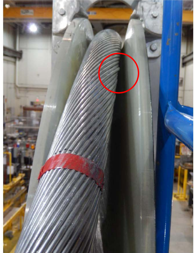
Figure 3b Slight protruding strand of the Conductor after Completing Sheave Test 2b (Note: the strand is just outside of the test section)
