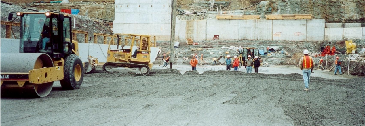
Spreading RCC with a Cat D5 dozer at North Fork Hughes River Dam. The laser detector is mounted on the blade for grade control.
