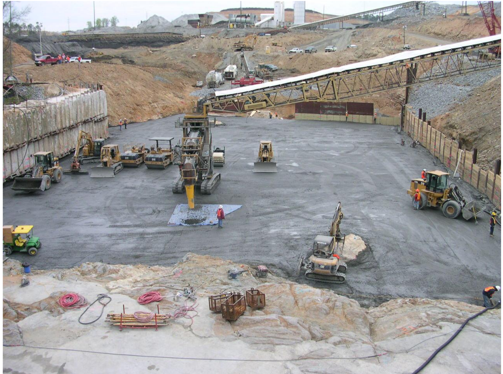
A crew uses a tarp to collect dry RCC as they prepare the lift surface for treatment
