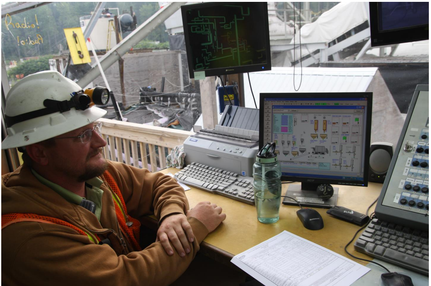
Plant Control Room at Gilboa Dam – Command Alkon Controls System
