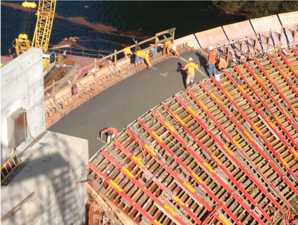
Ogee with Flip Bucket placed at the Crest of the Blue Lake Dam in Alaska, August 2014
