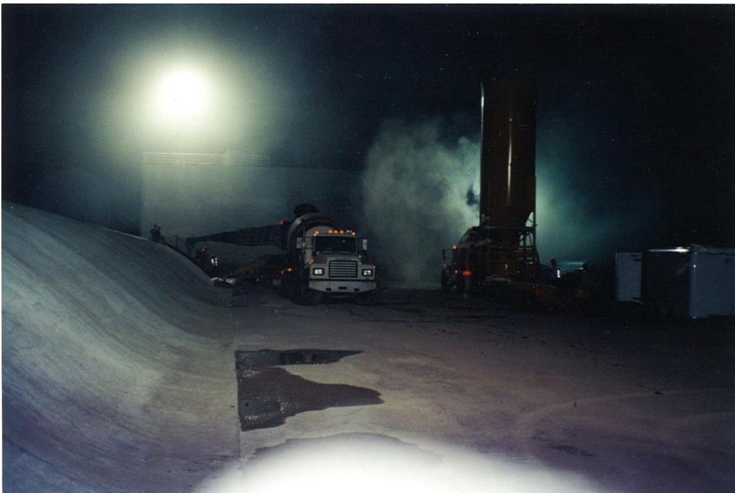
Ogee Crest placed over RCC at the North Fork Hughes River Dam
