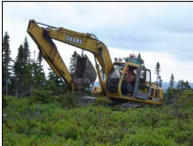
Photo 3: John Deere 160 LC track mounted excavator utilized in accessible areas of Lot 3.
