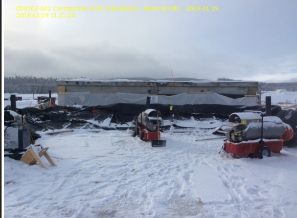
Control Building ( Pomerleau working on the hoarding from grid lines 3.1 to 3,5, in preparation for the formwork )
