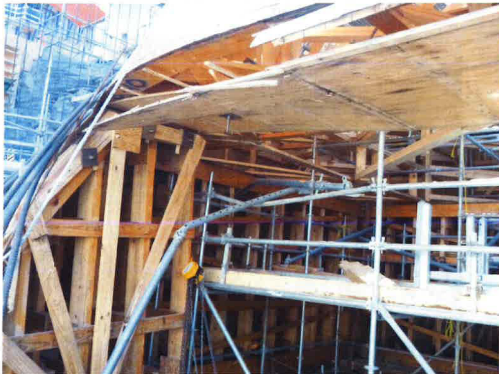
Figure 16: View of element A30 on the South side of collapsed A29
