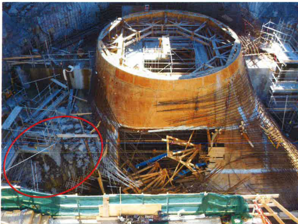
Figure 26: Non-conforming concrete circled in red.
