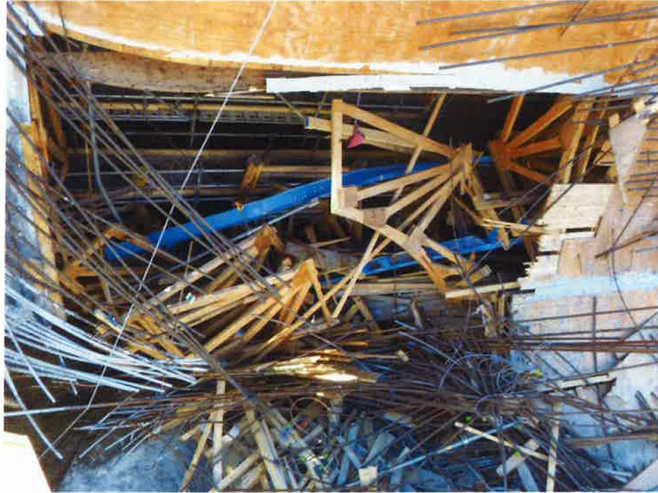
Figure 15: View from above of the hole left by the collapse of shoring towers supporting A29
