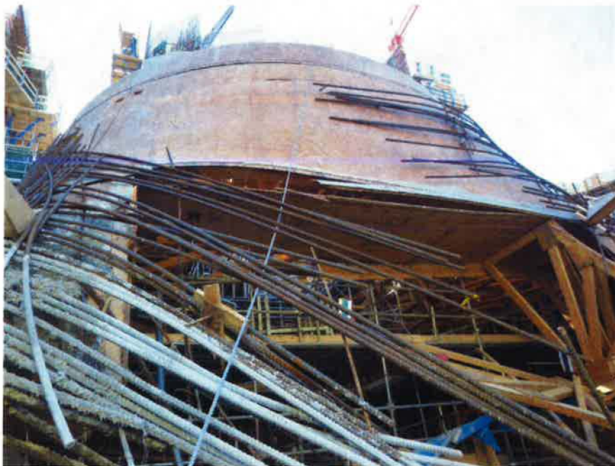
Figure 14: View from downstream of the hole left by the collapse of shoring towers supporting A29
