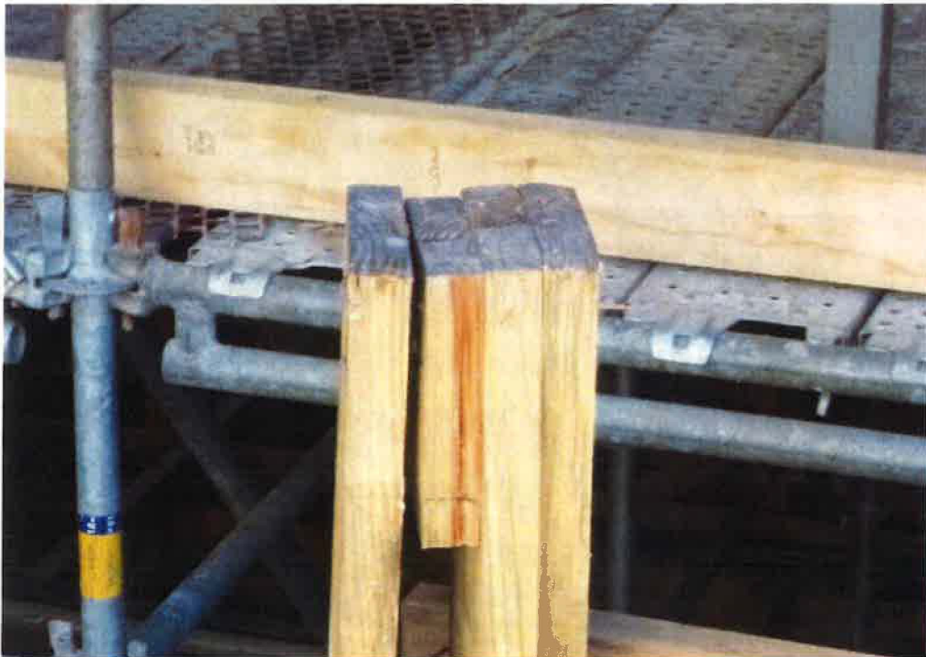
Figure 6: Shoring Tower C3, SW leg. Note compressed end grain in portions of leg.
