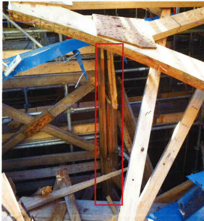
Figure 9: Tower C3 NW leg. Note separation of plies and missing elements
