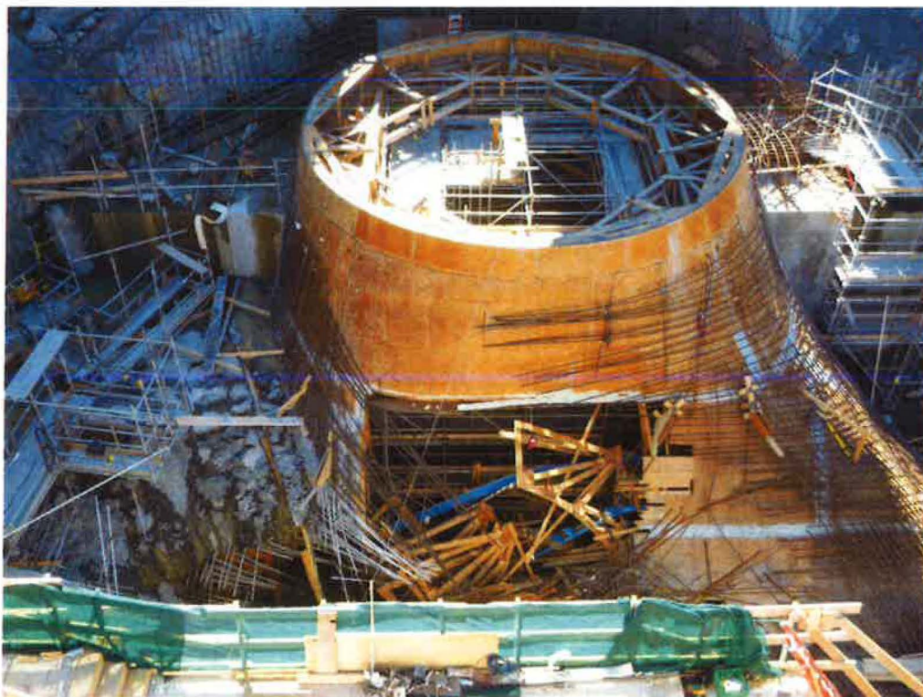
Figure 4: General view of the collapsed area taken from downstream.
