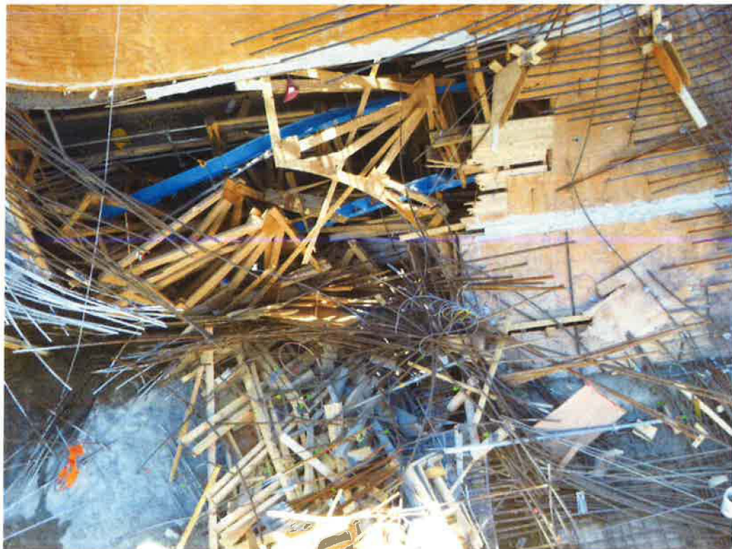
Figure 25: Debris, looking west.
