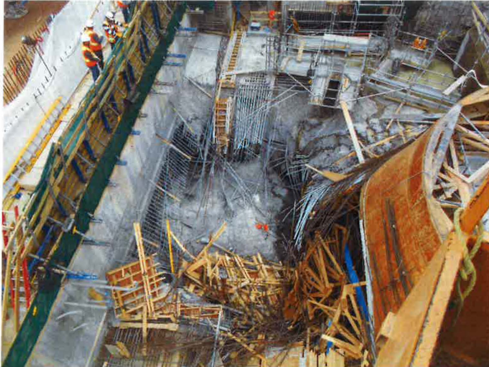
Figure 5: General view of the collapsed area taken from North
