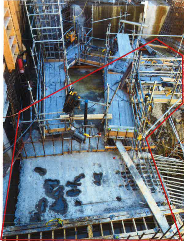
Figure 27: Approximate extents of non-conforming concrete, in red.
