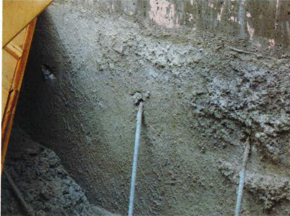
Figure 11: Ties remaining in the upstream face of pour D2USB-02
