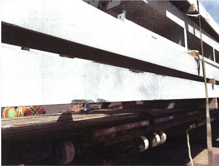
Figure 13 - Paint Damage at Shipment
