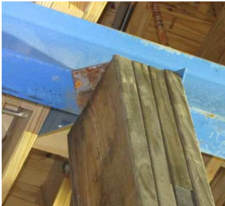
Figure 11: Inadequate shim plate (shifted plate)
