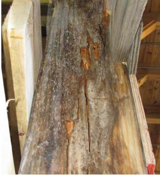
Figure 3: Highly weathered column member with extensive rot and damage due to overstress
