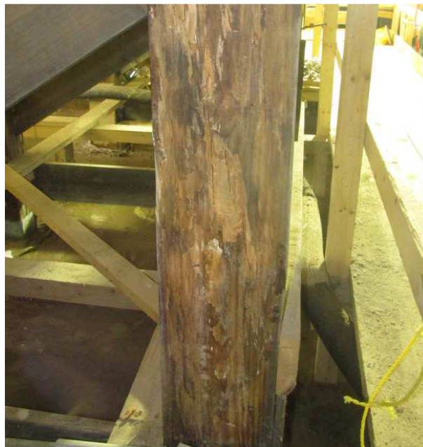
Figure 2: Highly weathered column member with extensive rot and damage due to overstress
