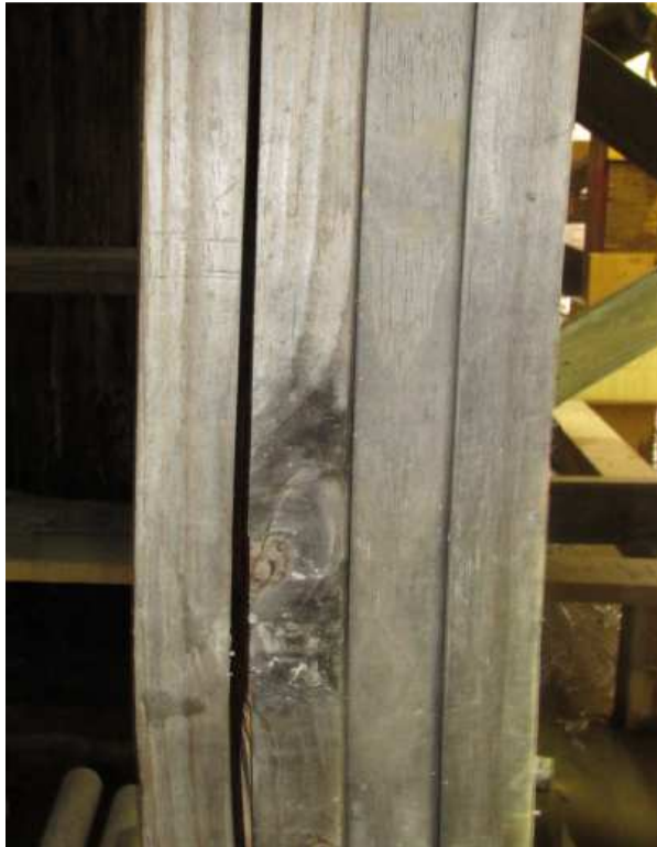
Figure 13: Inadequate nailing of column panels
