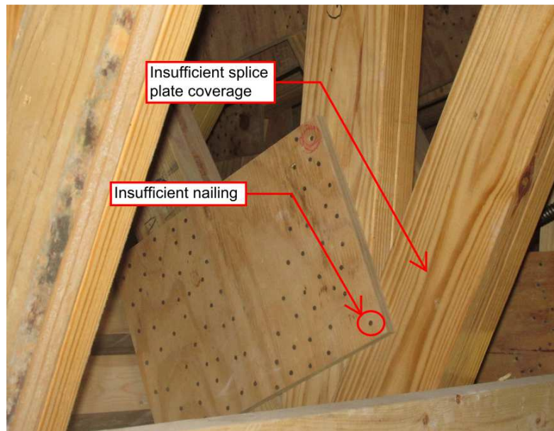
Figure 18: Inadequate splice plate coverage of structural member and insufficient nailing
