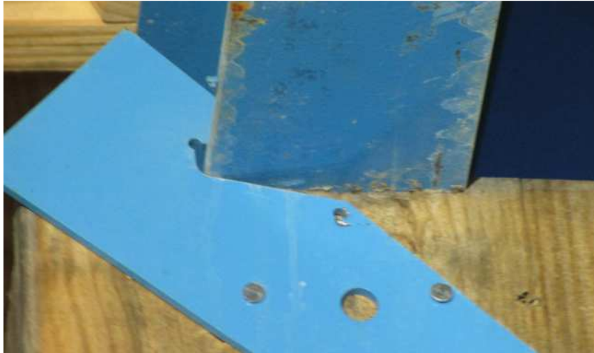
Figure 12: Localized end-grain compression due to lack of shim plate
