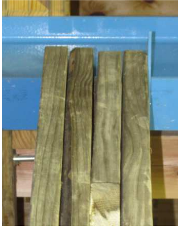
Figure 14: Inadequate nailing of column leg (tower B1)
