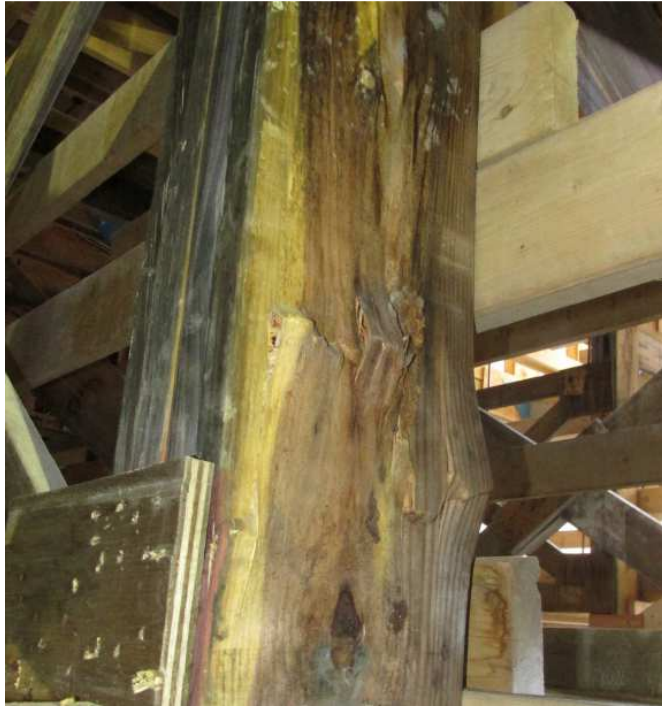
Figure 7: Compression failure of column member in tower B2
