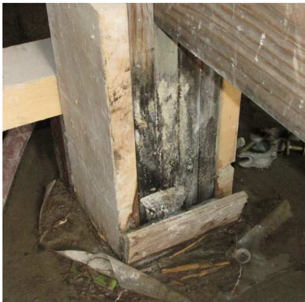
Figure 6: Highly weathered column base with moisture damage
