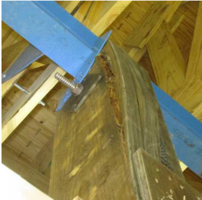
Figure 8: Compression failure of column member in tower B6
