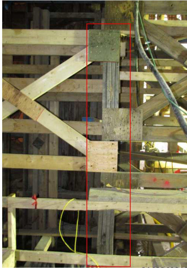
Figure 9: Buckling of column in tower B4
