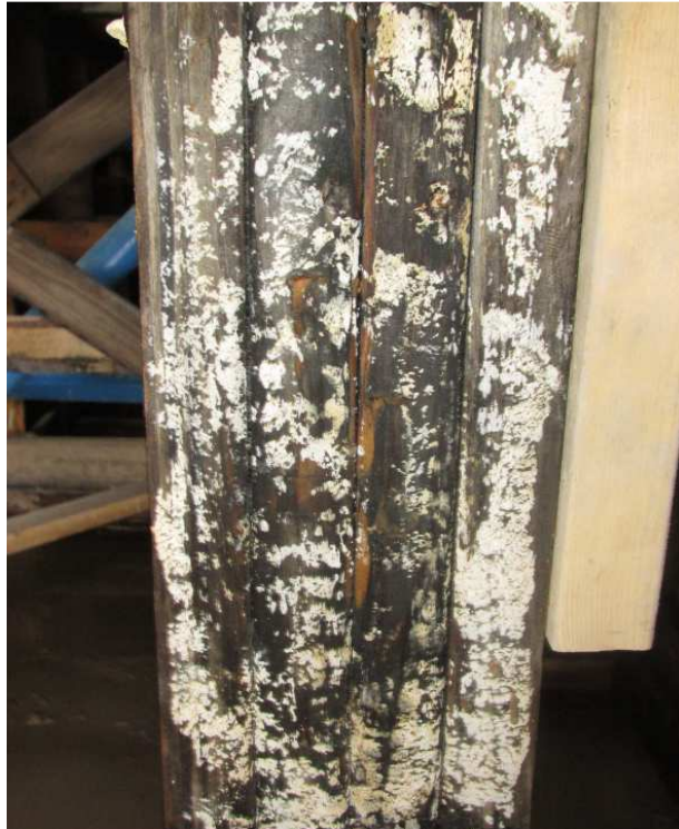
Figure 4: Highly weathered column member with mold growth
