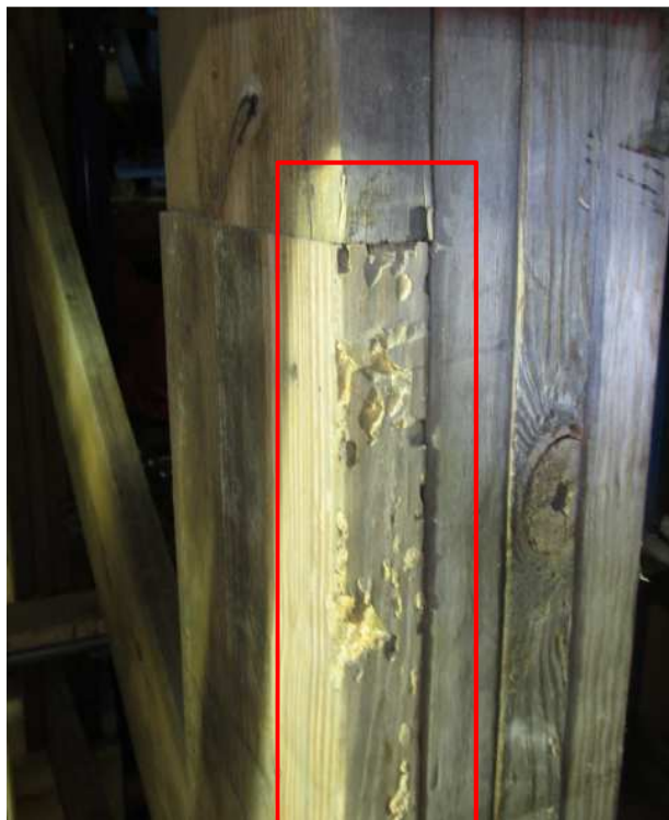
Figure 15: Termite damage on shoring tower leg with wood filler added
