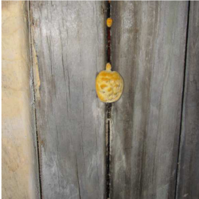
Figure 5: Weathered column member with fungal growth
