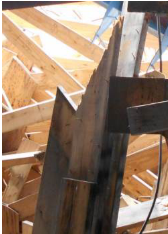
Figure 18: Inadequate nail length (did not penetrate all column laminations)
