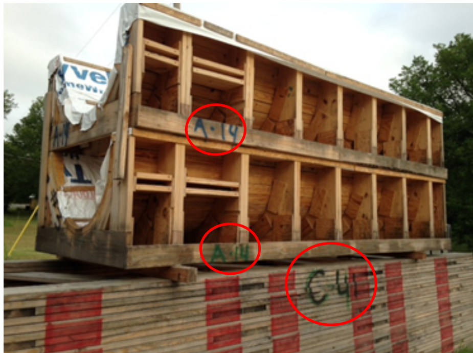
Figure 22: Formwork and falsework with multiple color markings "C41" and "A14" at CEI's facility
