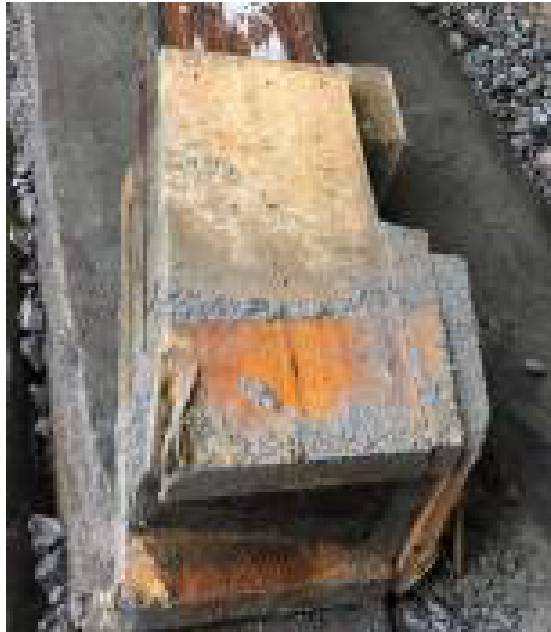
Figure 61: Alternate grout form at base of falsework tower leg. Recovered from Row C towers DT2
