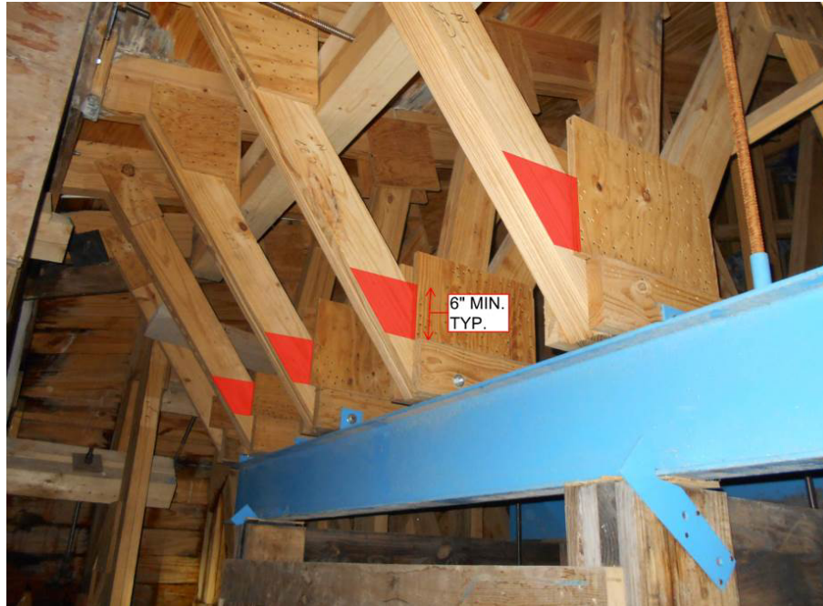
Figure 17: Inadequate splice plates should extend to area in red
