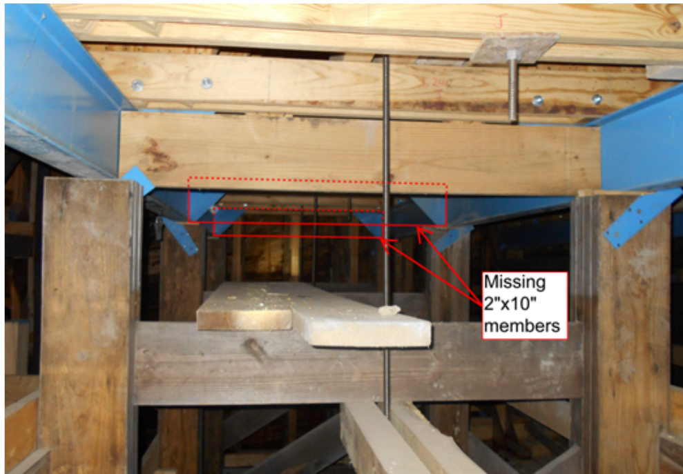
Figure 57: Missing members between beams. DT3 tower B1
