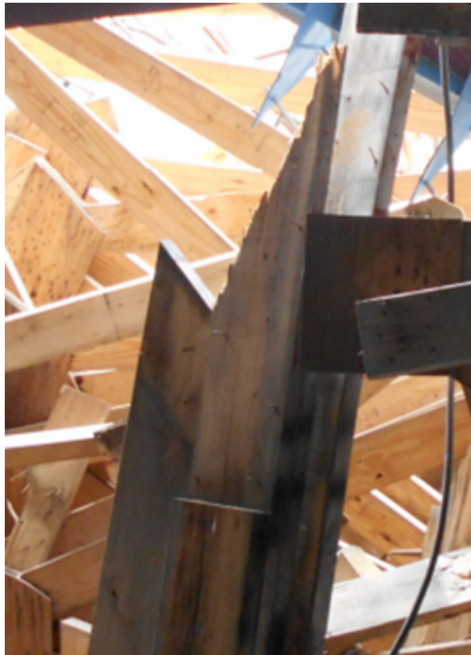
Figure 55: Inadequate joining of built-up member
