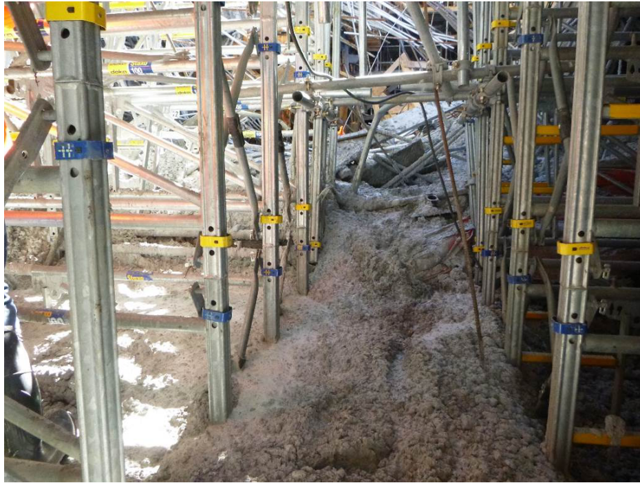
Figure 10: DT 2 south outlet looking upstream (west) into failure area
