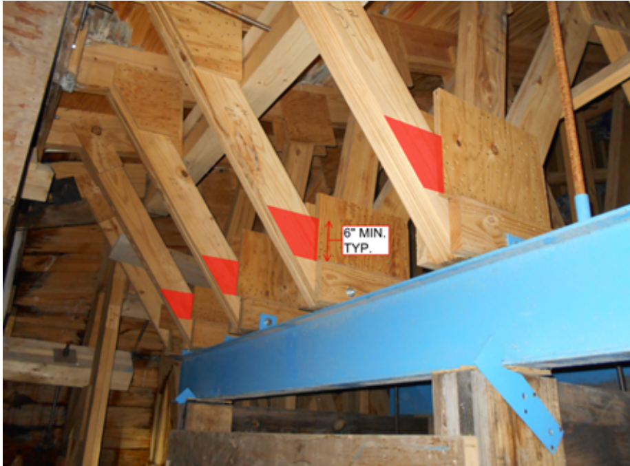
Figure 58: Inadequate splice plate size DT2
