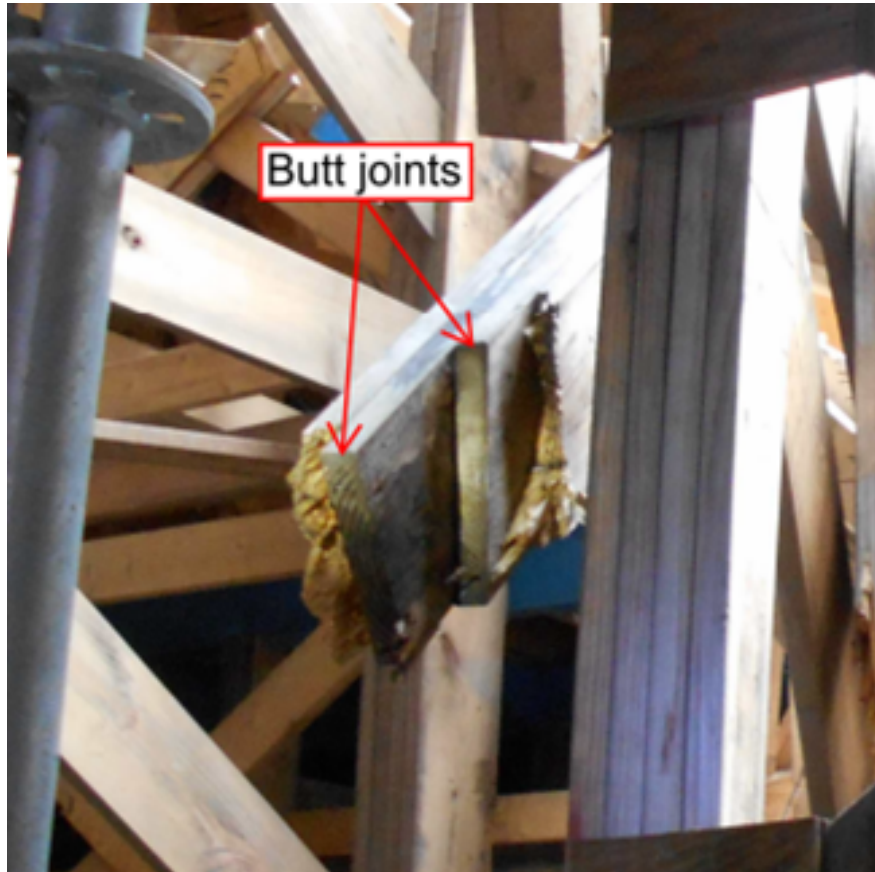
Figure 59: Close proximity of butt joints in broken tower leg
