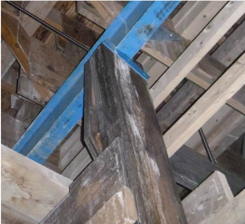
Figure 51: Local failure of tower leg at bracing penetration in DT1
