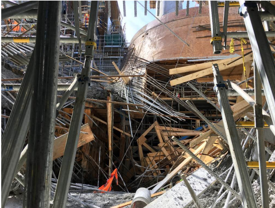
Figure 12: DT2 failure area looking west from northern portion of DT2 south outlet
