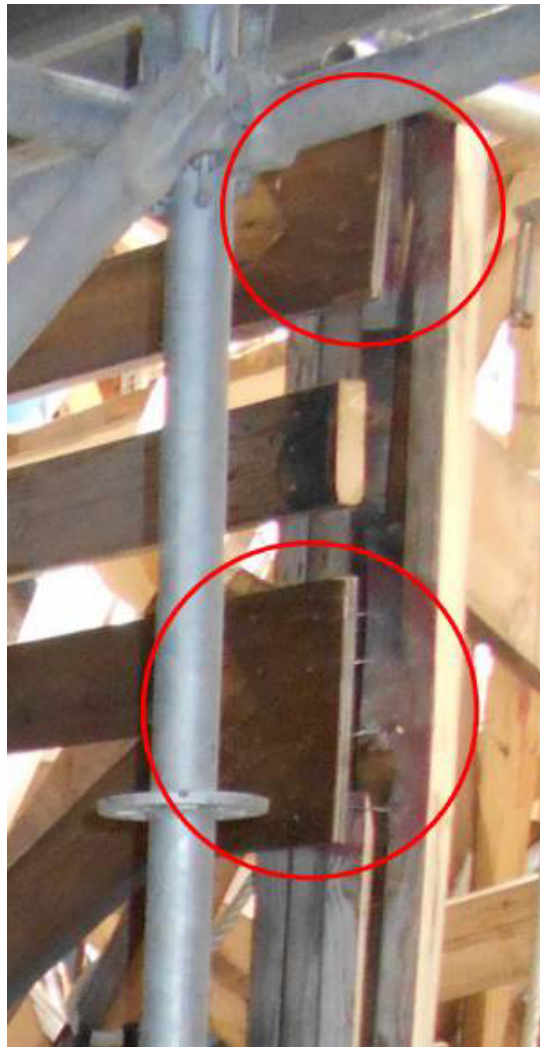
Figure 25: Splice plates pulling away from column legs
