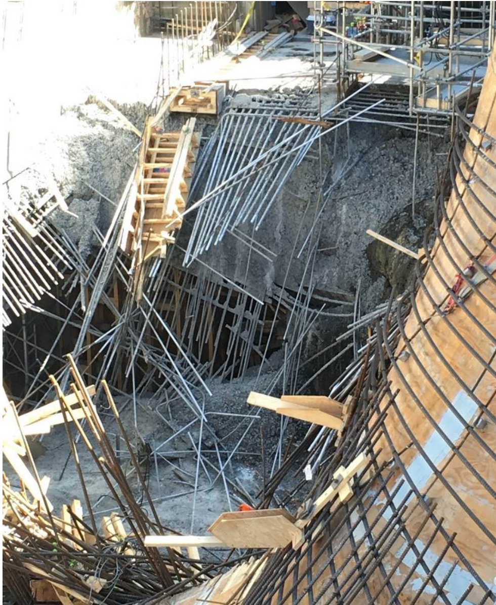
Figure 9: DT2 failure area looking southeast
