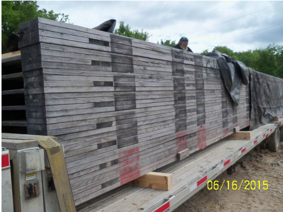
Figure 65: June 16, 2015 at CEI yard. Left hand view of falsework towers believed to be installed in DT2
