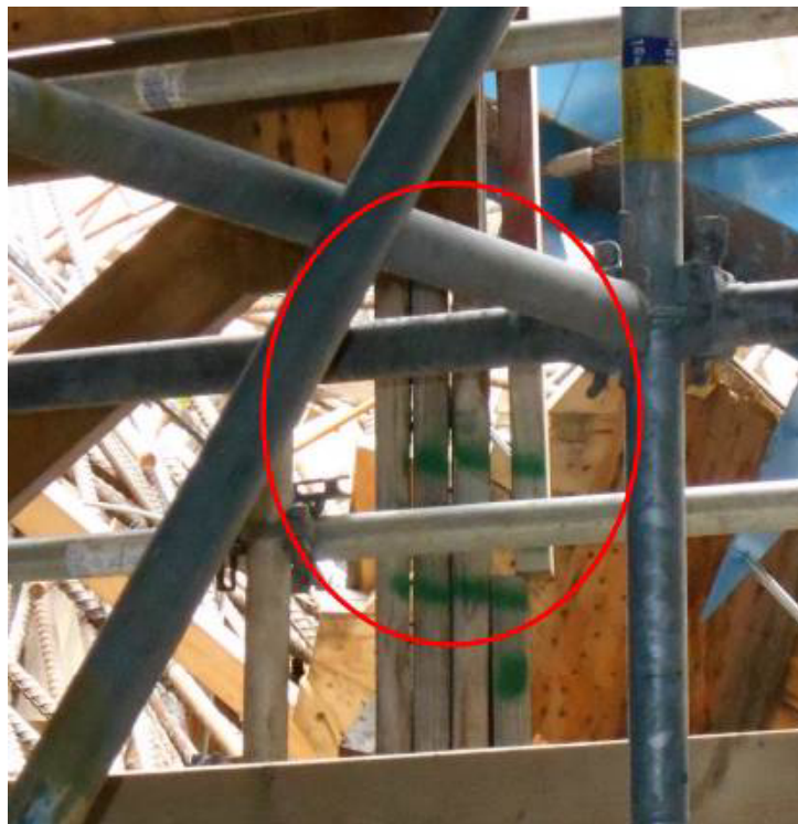
Figure 19: Built-up column members separating due inadequate joining
