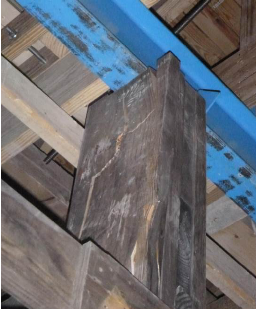
Figure 52: Local failure of tower leg at beam interface and bracing penetration in DT1
