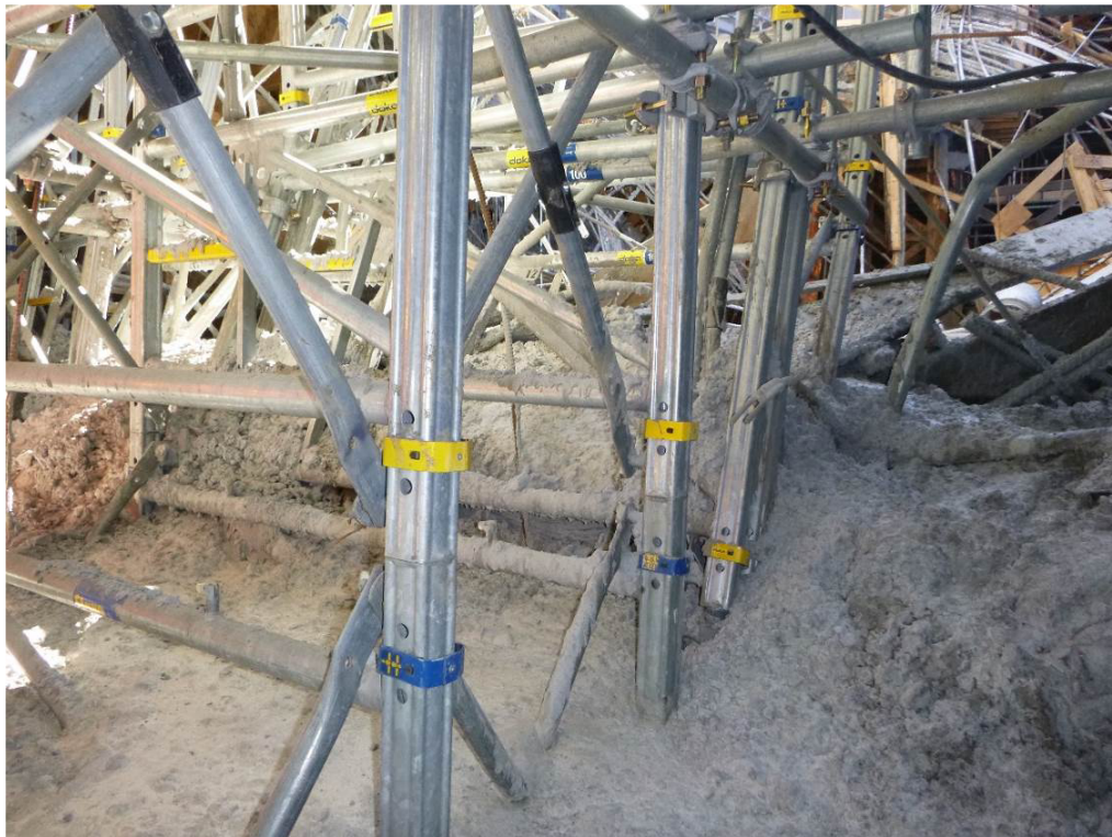
Figure 11: DT2 south outlet looking west-southwest into failure area
