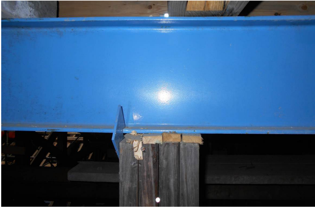
Figure 28: Inadequate shimming on top of falsework towers. No bearing plate installed.
