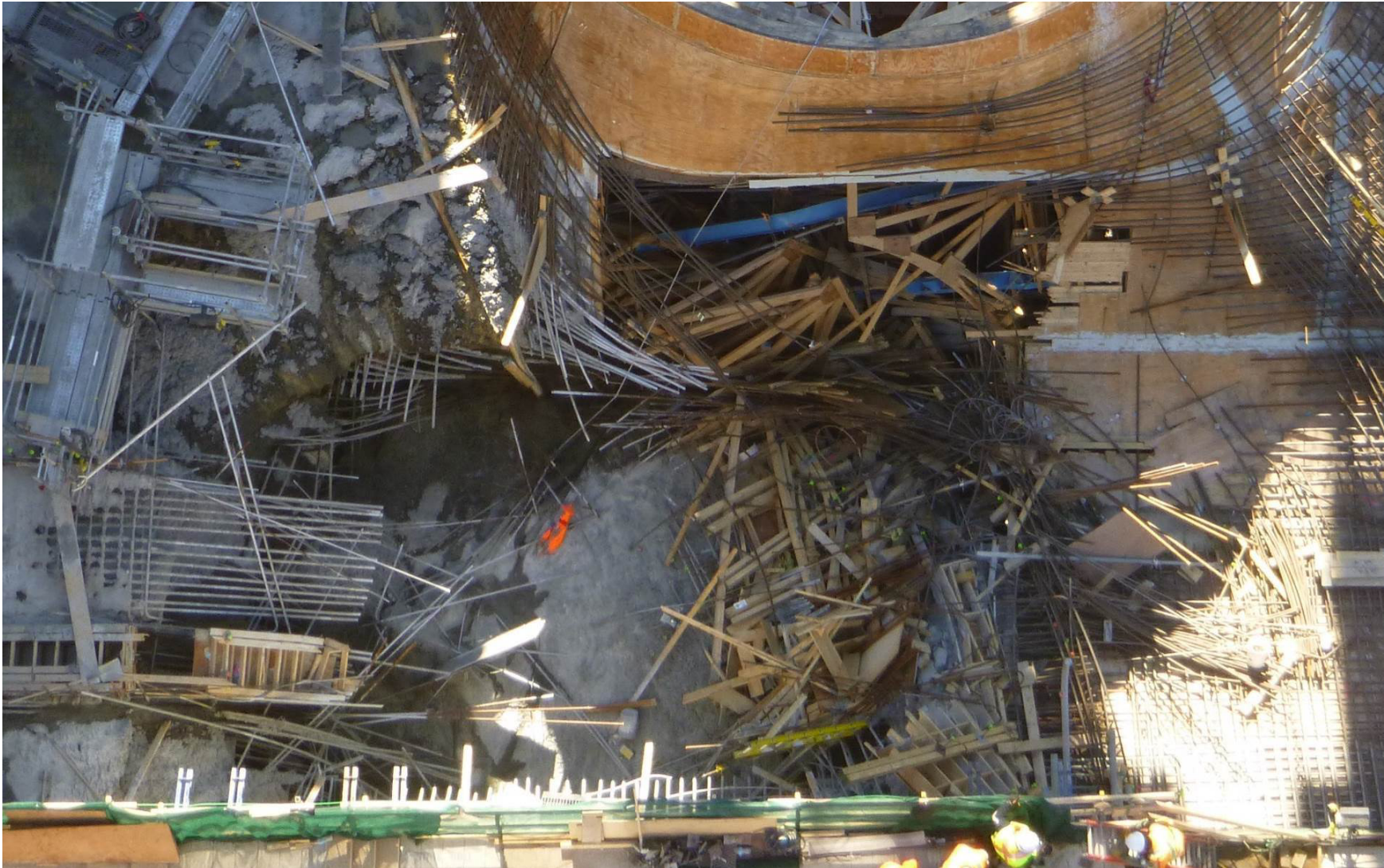
Figure 15: DT2 failure area from man basket
