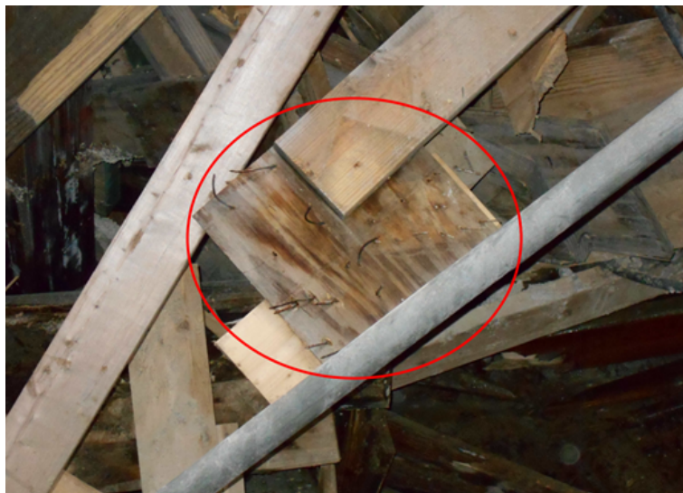
Figure 54: Inadequate nailing of splice plate in DT2
