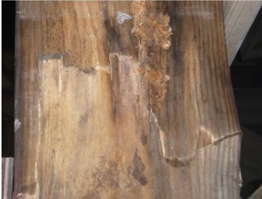
Figure 50: Local failure of outer ply of tower leg in DT1
