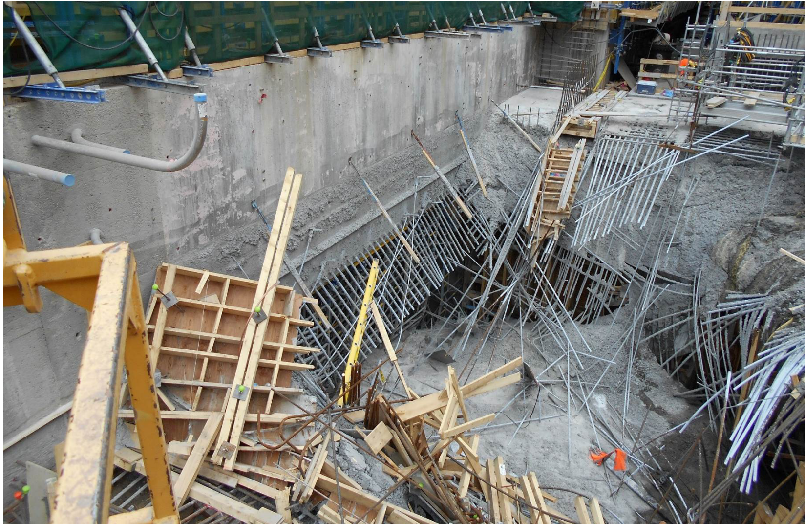
Figure 16: DT2 failure area from man basket looking southeast
