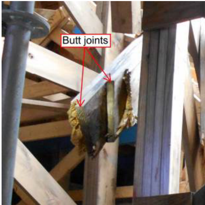
Figure 21: Close proximity of butt joints in broken tower leg
