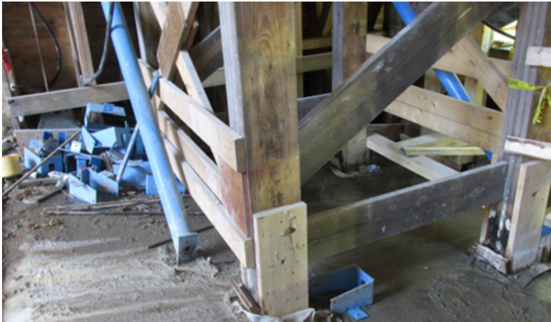
Figure 60: DT1: Uninstalled tower base anchors (blue steel clips) in foreground and piled in background. Alternate grout pad with form installed in foreground left and right.
