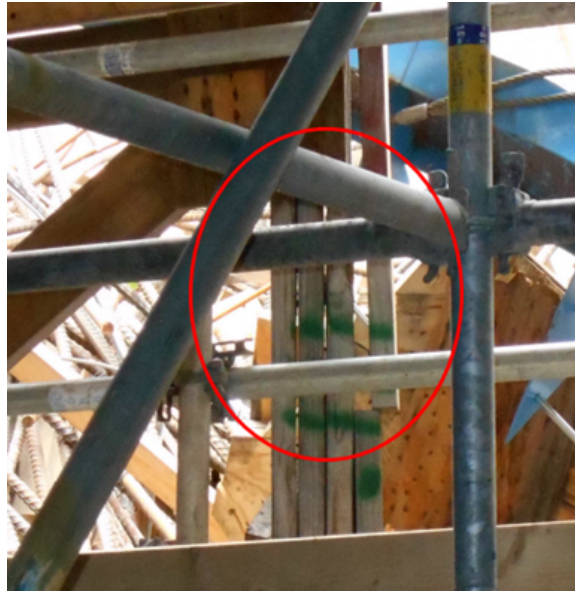
Figure 56: Inadequate joining of built-up member, members separating
