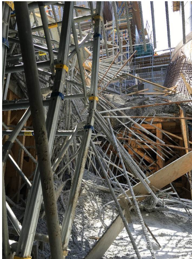
Figure 13: DT2 failure area looking west from southern portion of DT2 south outlet
