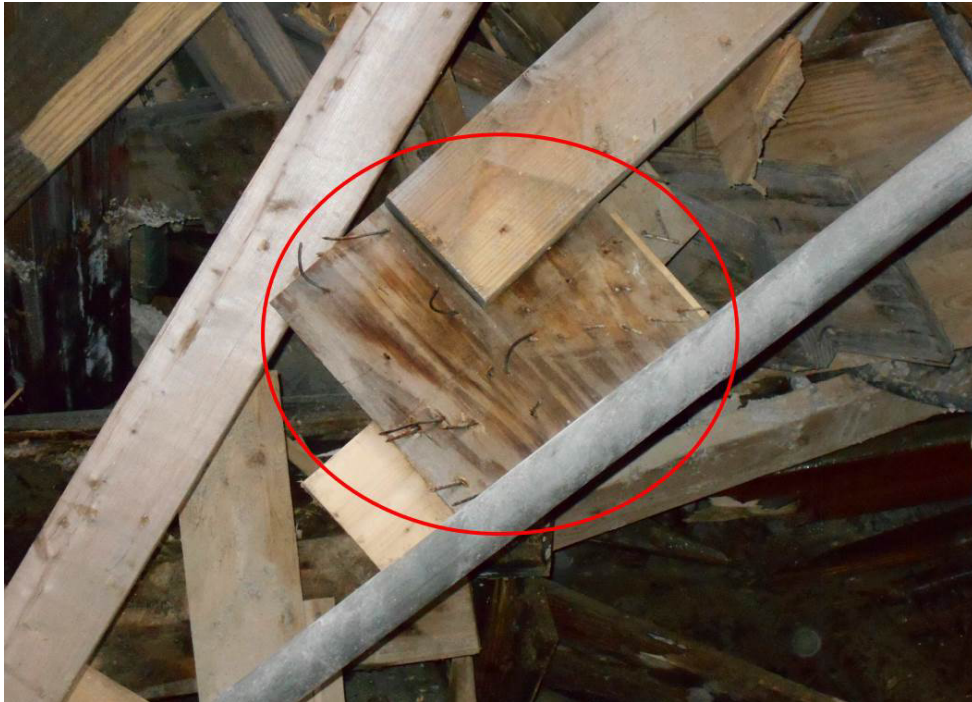
Figure 26: Splice plate pulled away from tower leg
