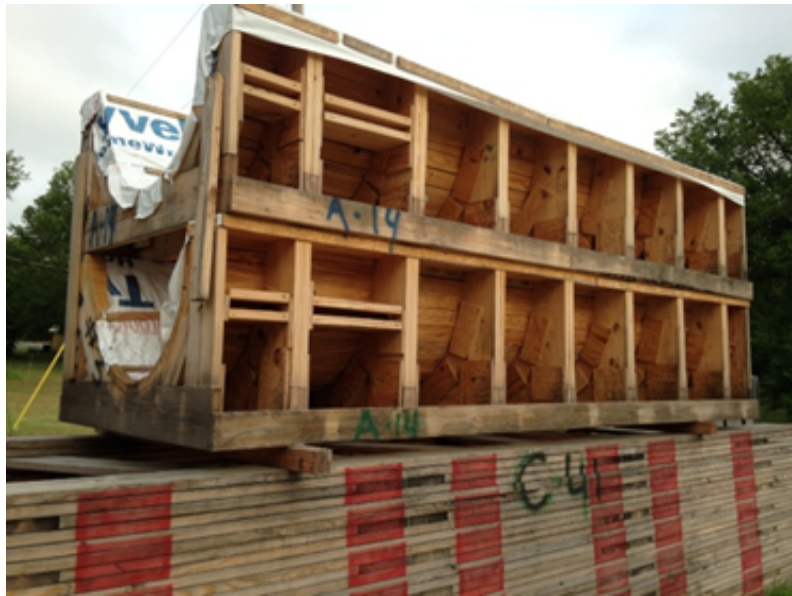
Figure 63: July 23, 2014. Formwork and falsework at CEI facility. Note weathering of wood compared to same material in Figure 62.
