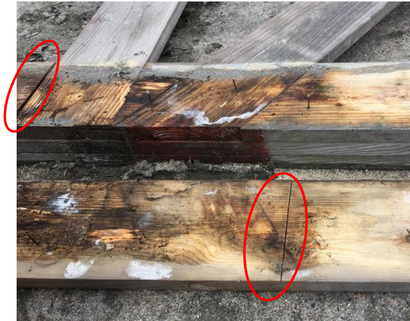
Figure 43: Gaps in Tower Leg Butt Joints (left) and saw kerfs (right) from DT3
