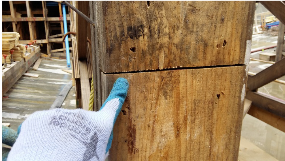
Figure 44: Gap in Tower Leg Butt Joint in DT3
