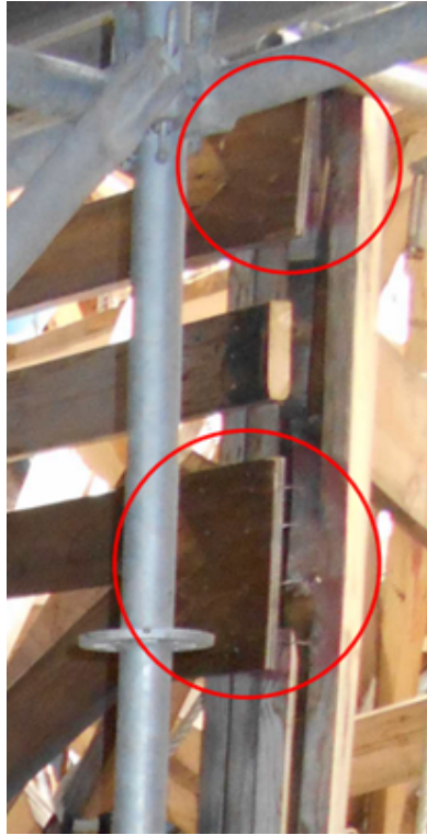
Figure 53: Splice plates pulling away from column legs in DT2
