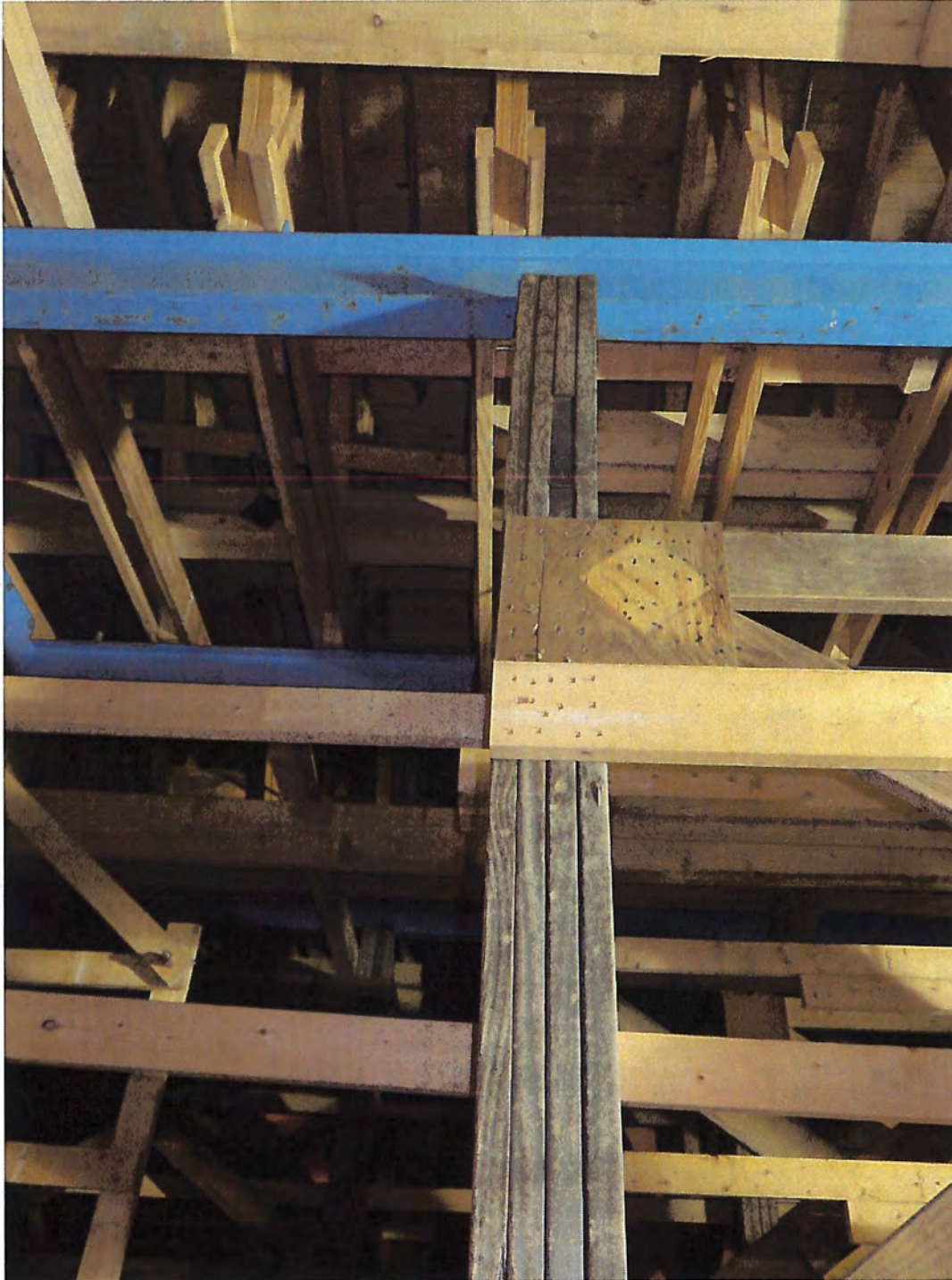
Unit 1 - Tower B2, buckling at top of post
