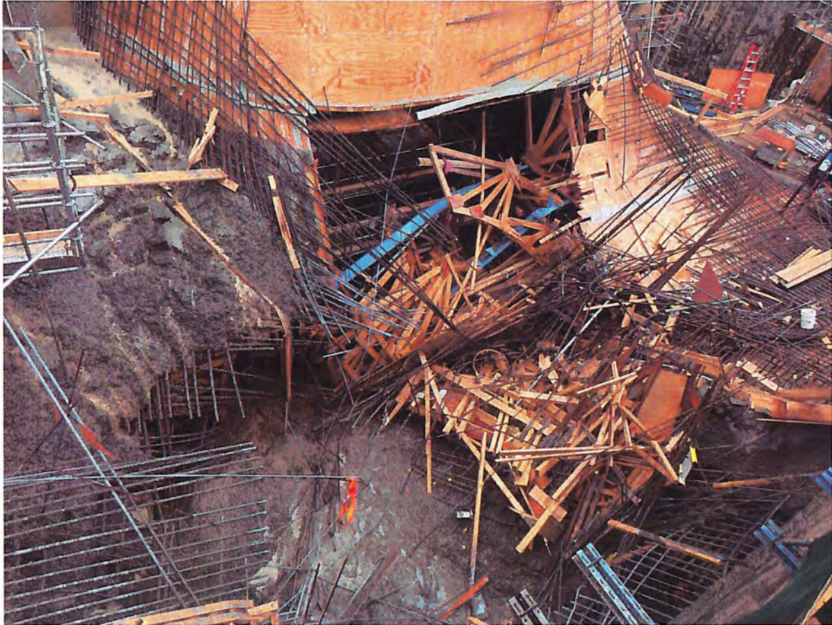
Unit 2 draft tube - View of South East corner of unit, looking below
