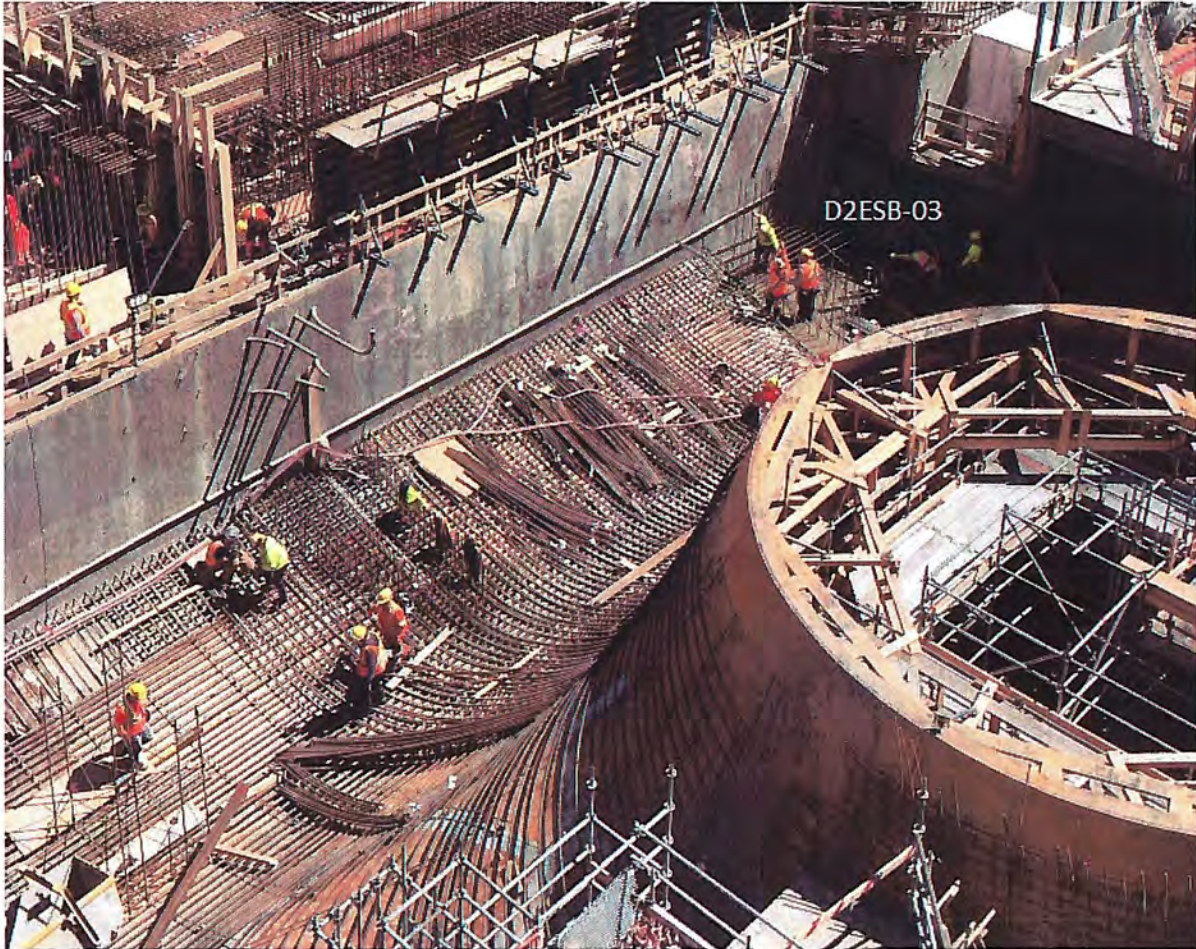
Unit 2 draft tube - View from the North West corner of unit, looking below
