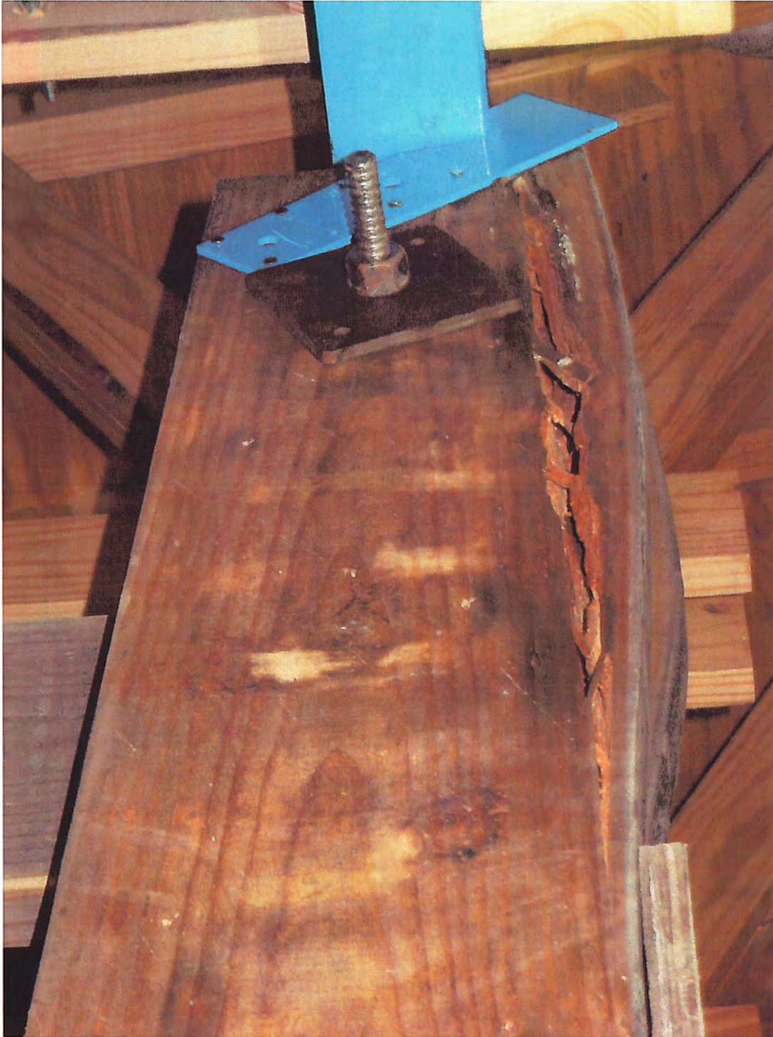
Unit 1 - Tower B1, compression failure below steel beam
