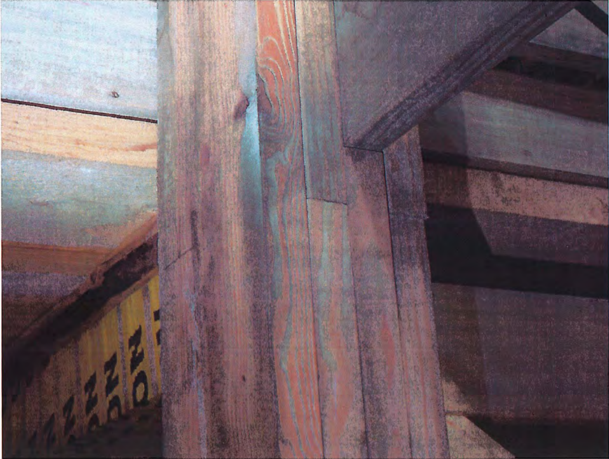
Unit 4 - Inappropriate location for built-up column joint
