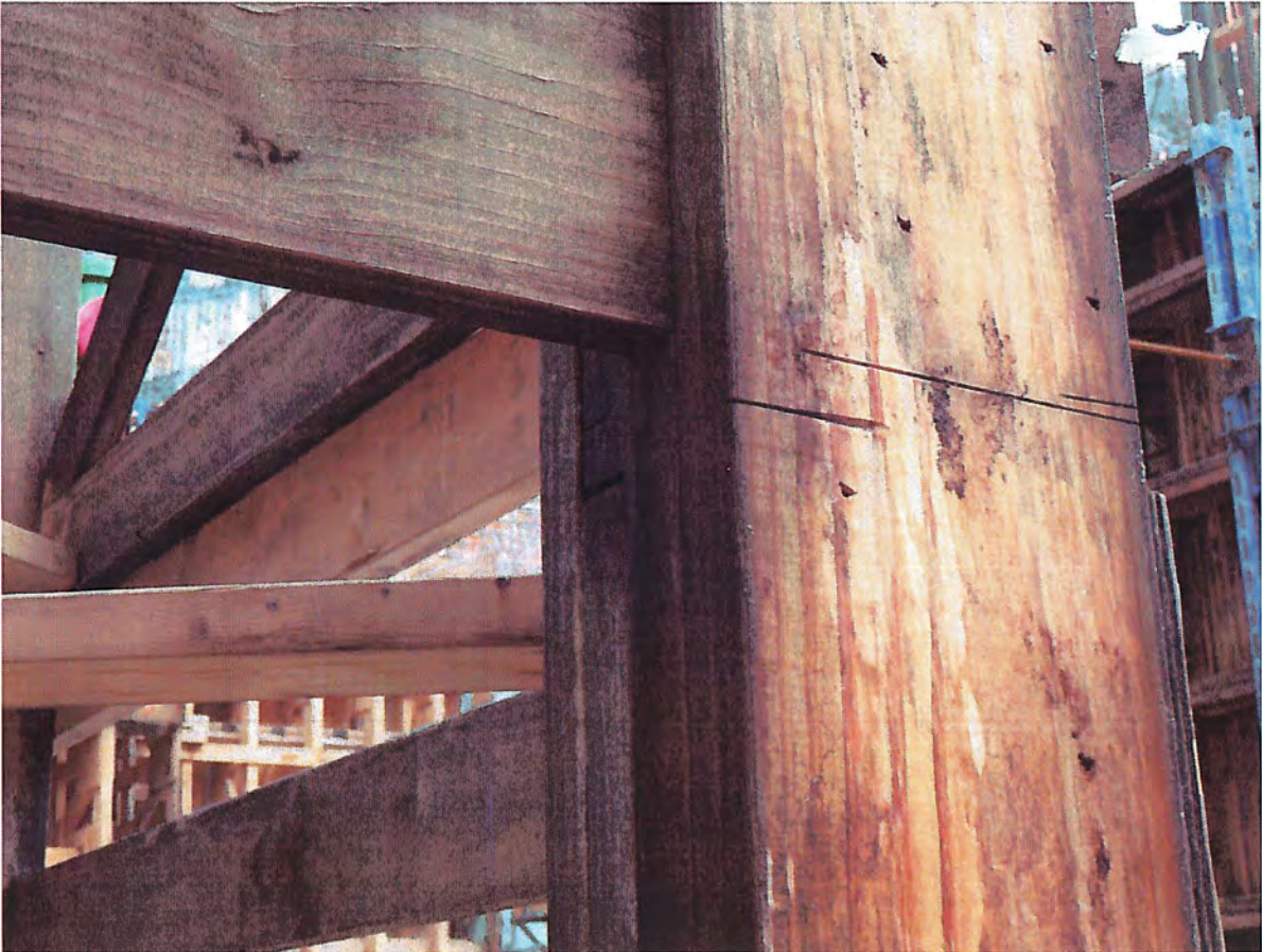
Unit 3 - Saw cut mark in lumber
