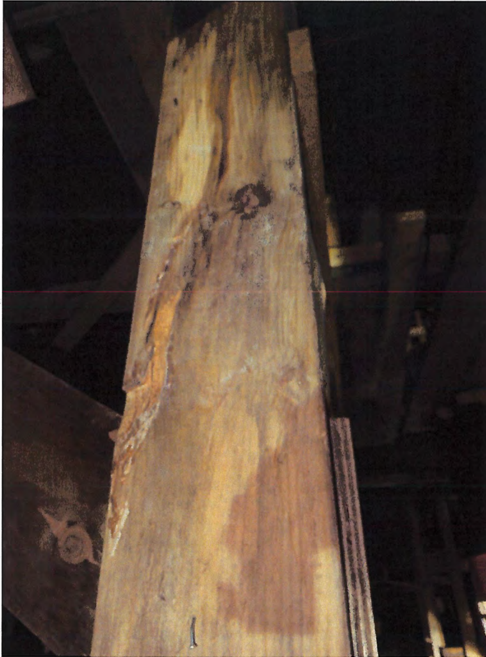
Unit 1 - Fungi growth on lumber of tower B4
