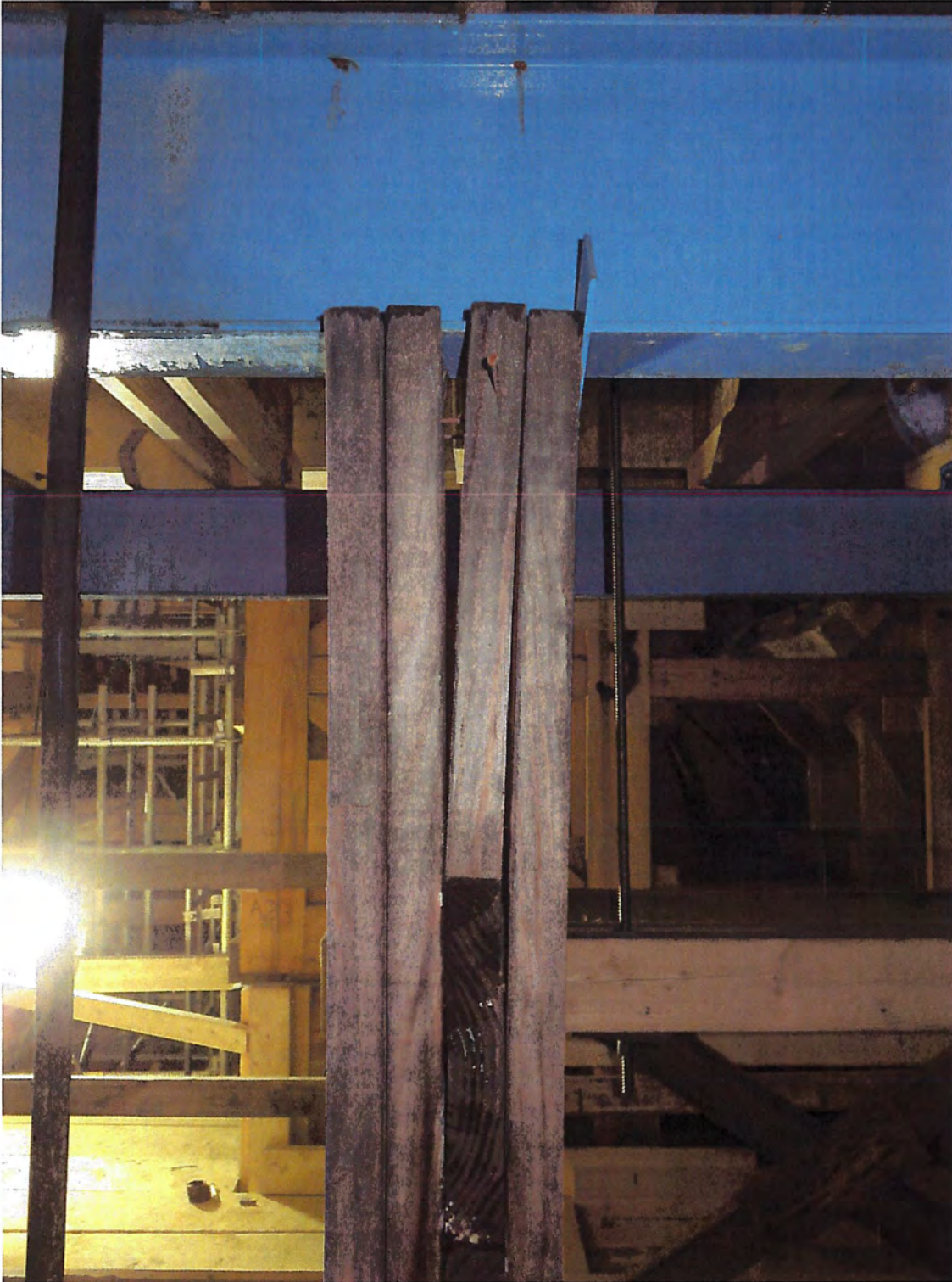
Unit 4 - Damage to tower during formwork or tower alignment
