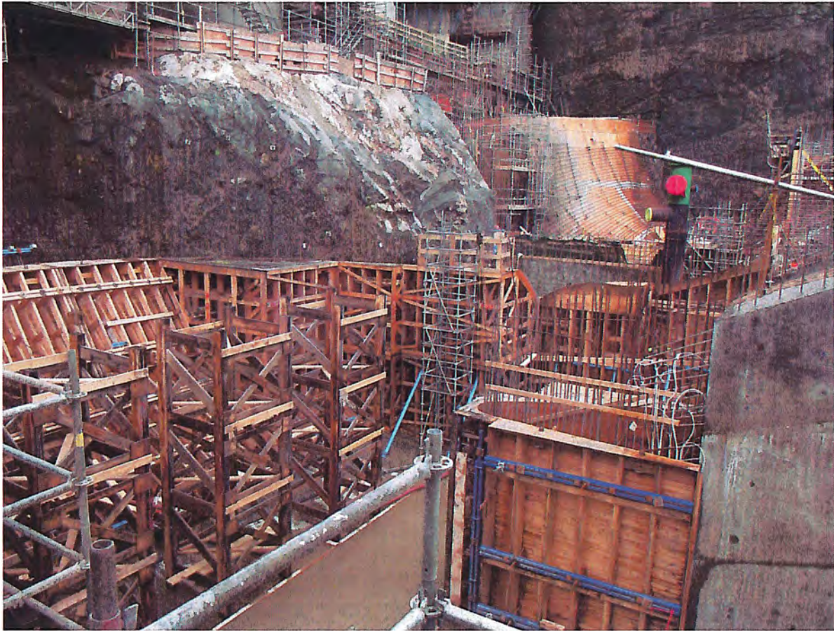
Unit 3 - Installed shoring tower weathering
