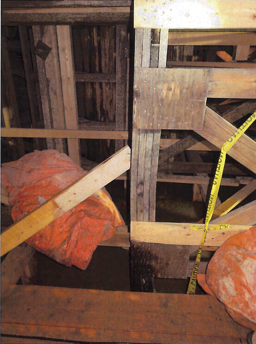
Unit 1 - Tower B3, buckling at bottom of post
