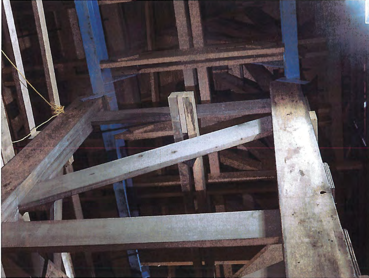
Unit 4 - Tower misaligned with steel beam
