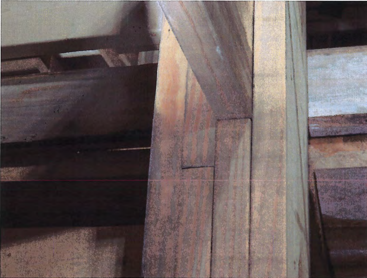
Unit 4 - Inappropriate location for built-up post joint
