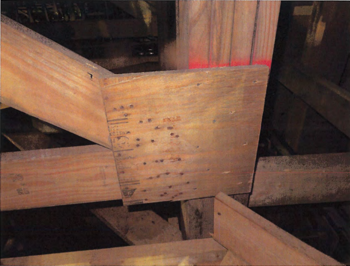
Unit 4 - Tower brace installed on site – Insufficiently nailed
