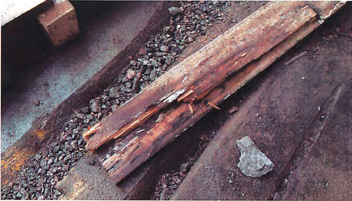
Unit 2 - Shoring tower rotten lumber
