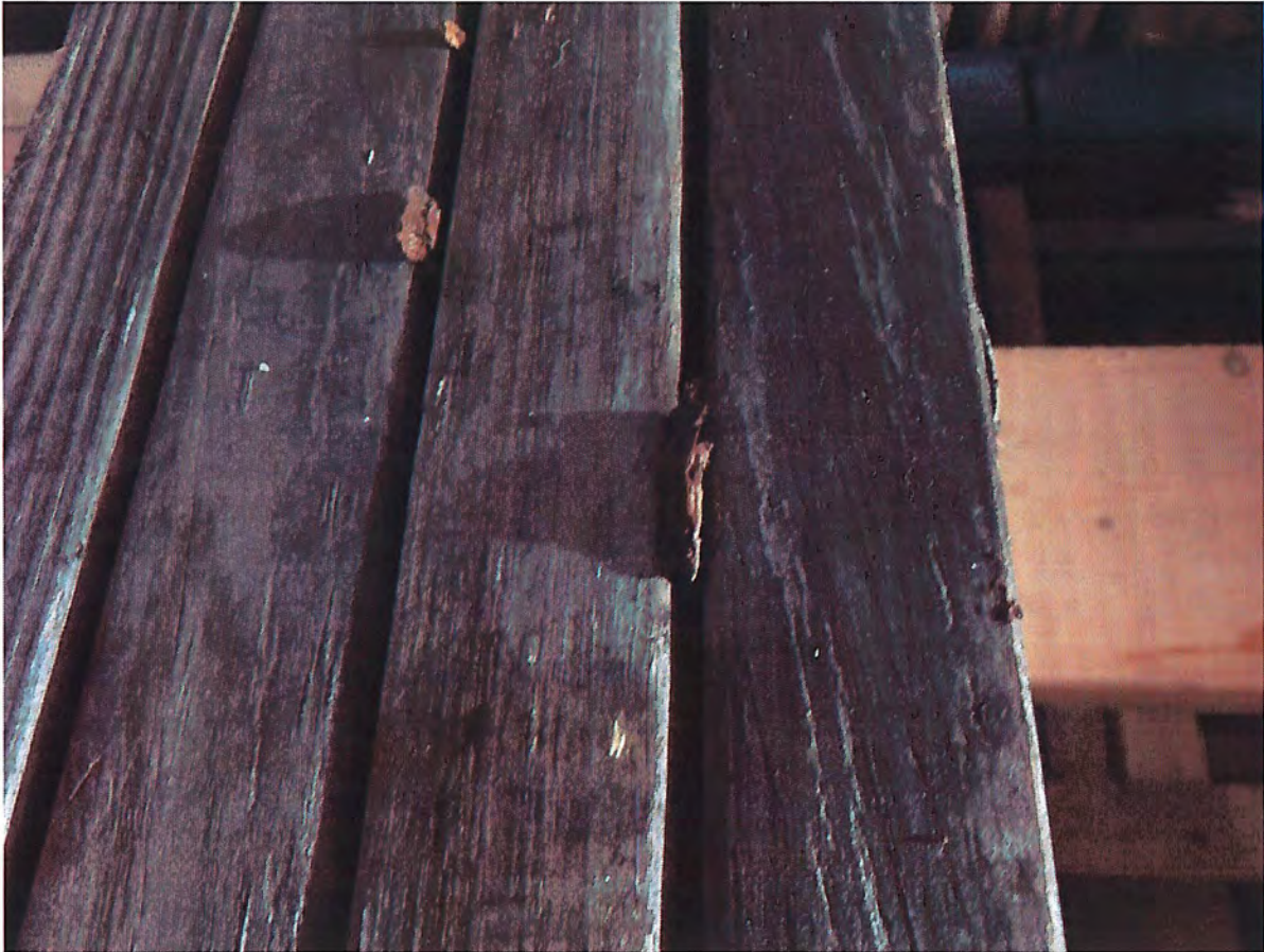
Unit 1 – Mushroom growth on tower B3
