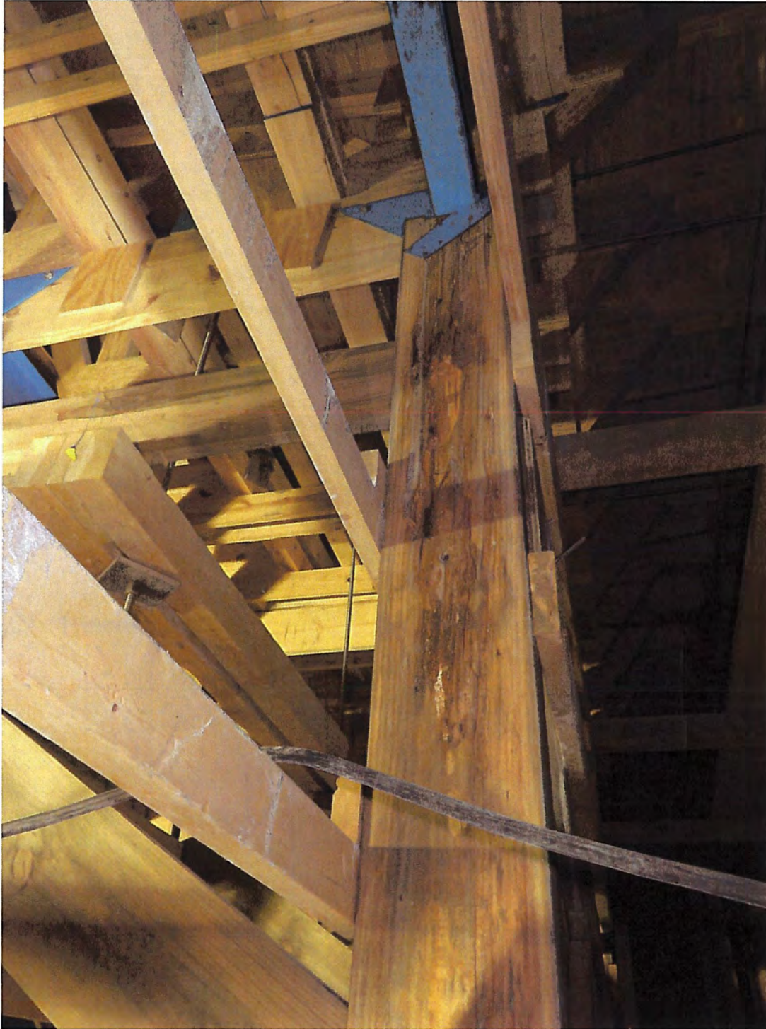
Unit 1 - Decayed wood on tower B2
