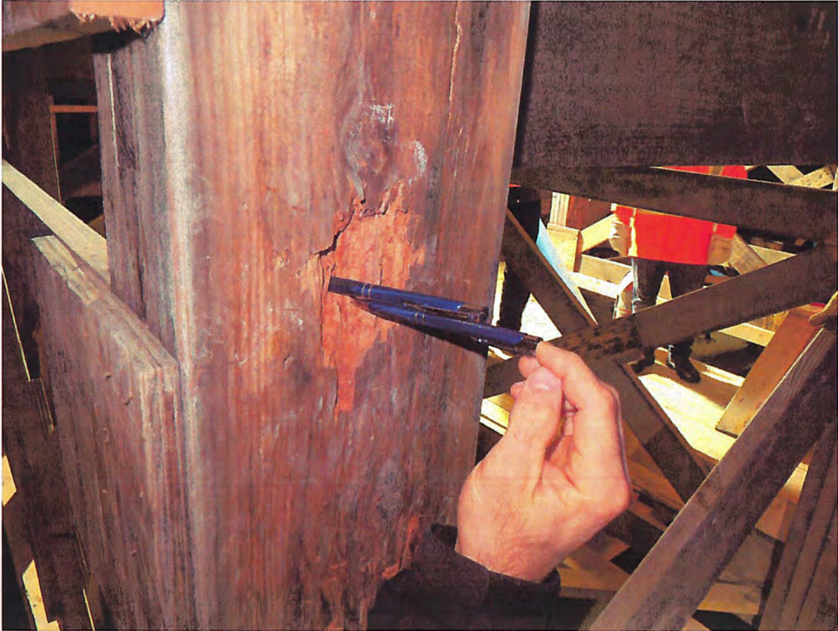
Unit 1 - Dry rot on shoring tower
