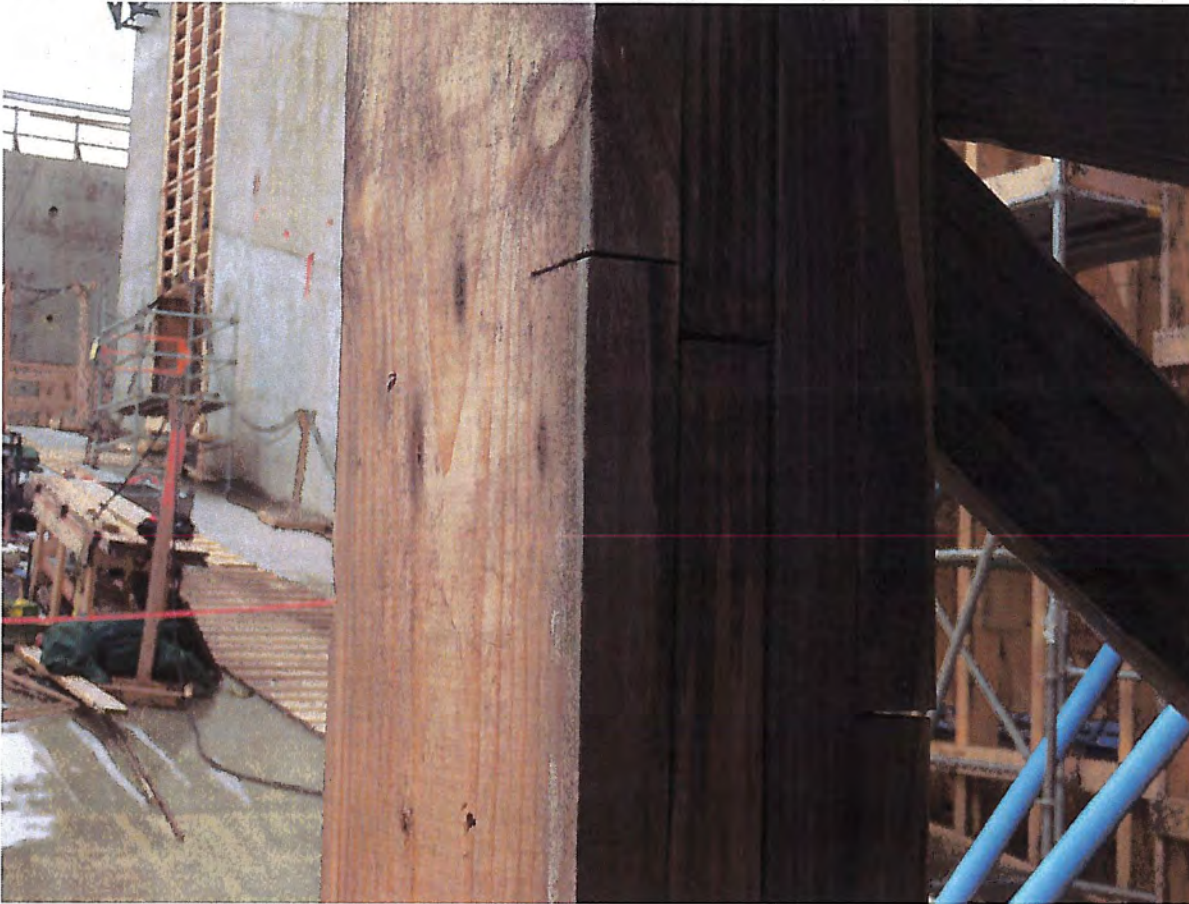
Unit 3 - Saw cut mark in lumber
