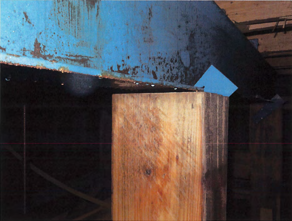
Unit 4 - Missing shim between post and steel beam
