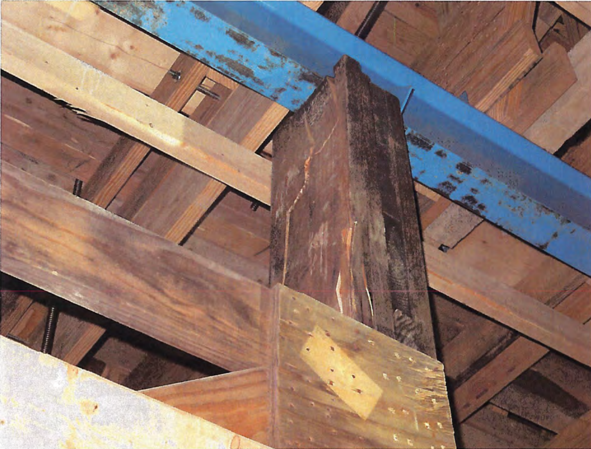
Unit 1 - Tower B5, compression failure below steel beam
