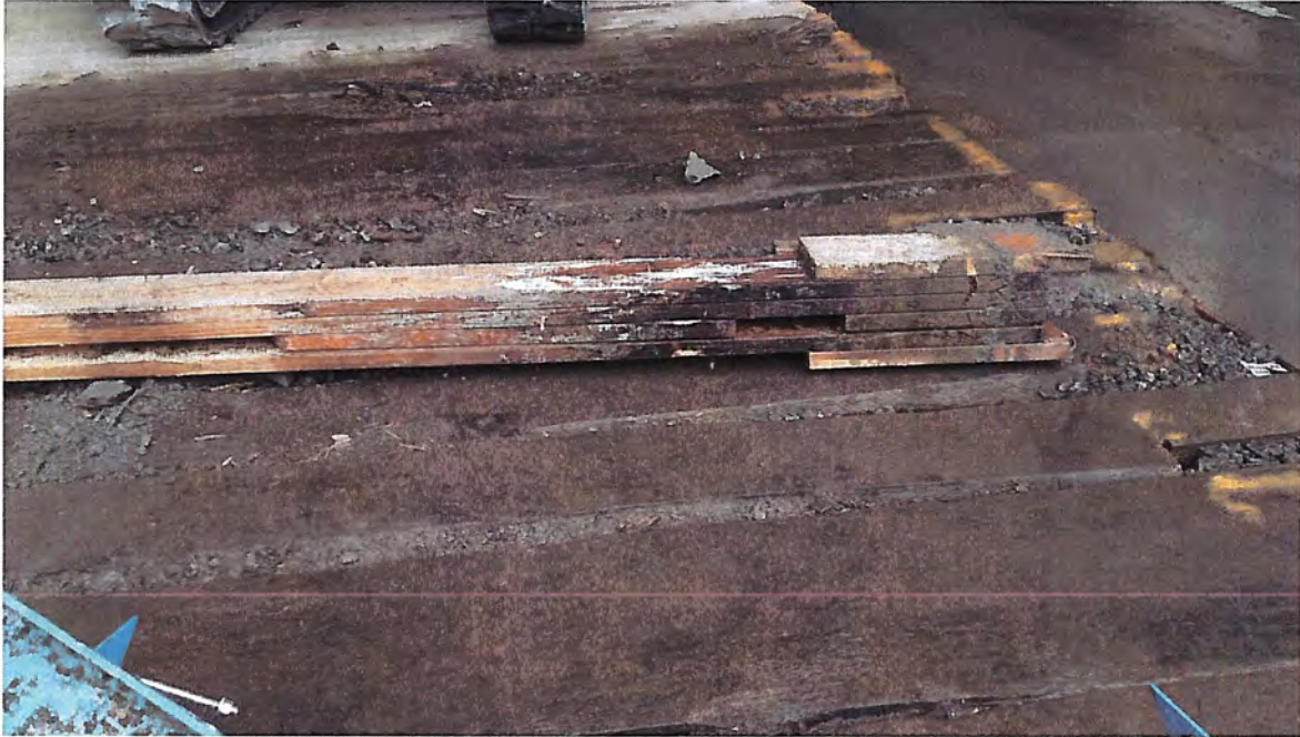
Unit 2 - Shoring Tower weathering
