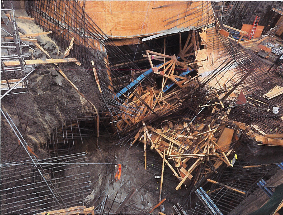
Figure 2: Unit 2 draft tube formwork collapse - view of SE corner of unit
