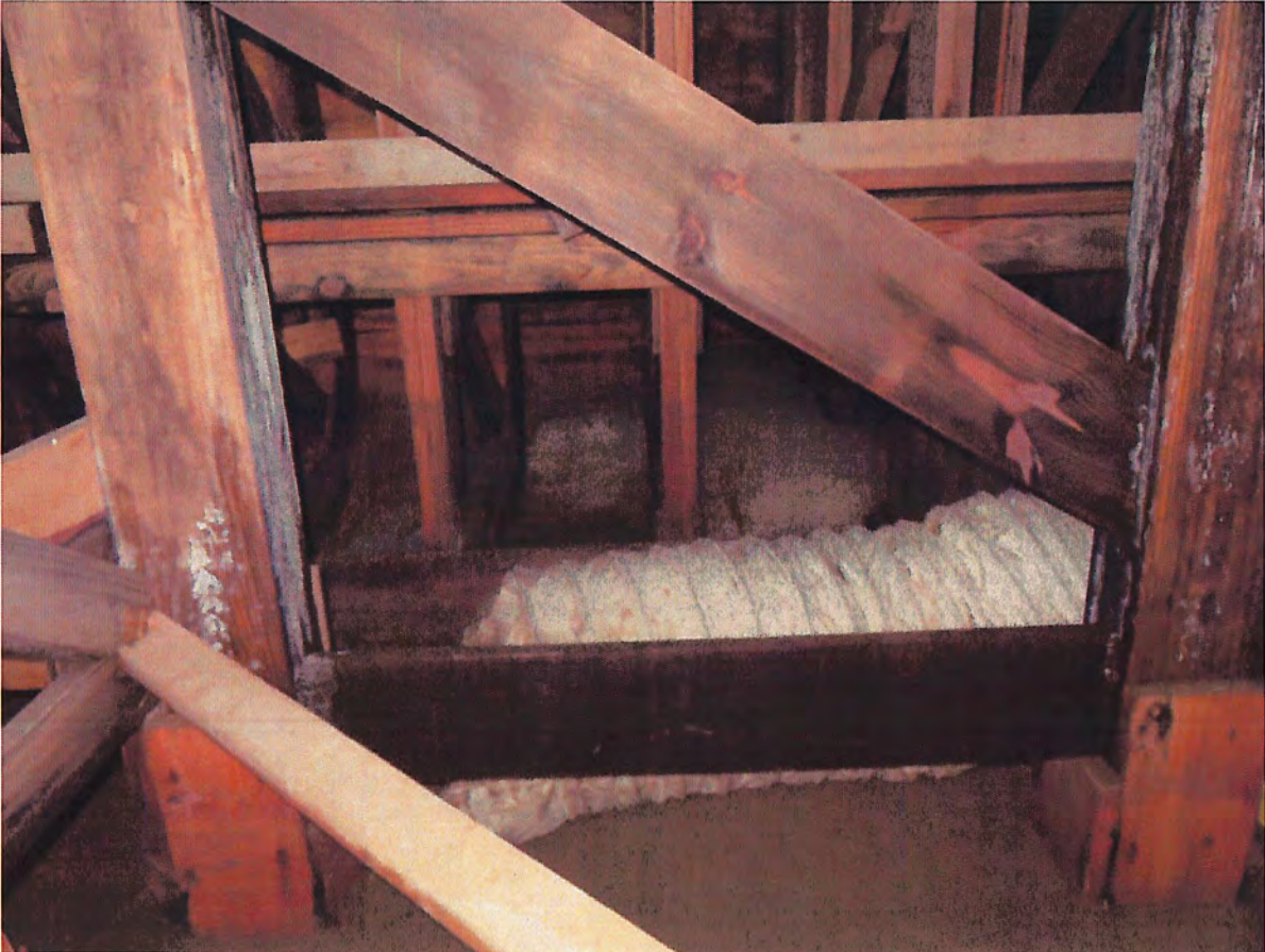
Unit 1 - Fungi growth on lumber of tower B6
