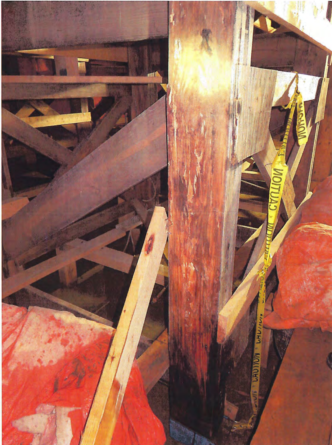
Unit 1 - Decayed wood on tower B3
