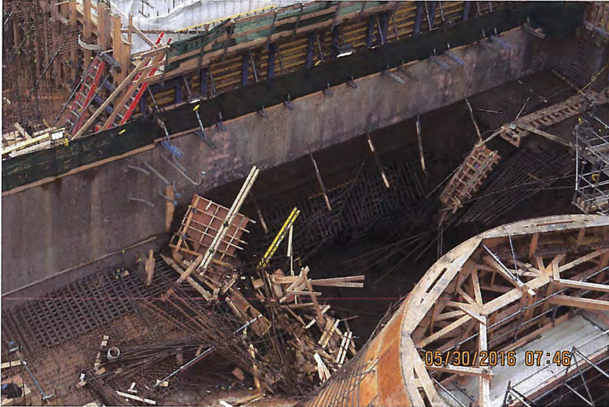
Unit 2 draft tube - View from North West corner of unit, looking below
