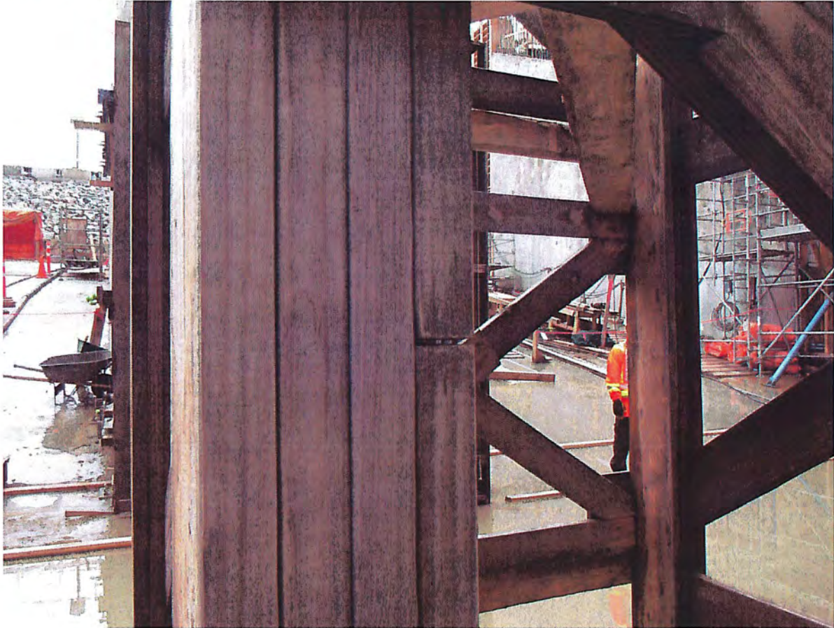
Unit 3 - Built-up tower with a gap between two planks
