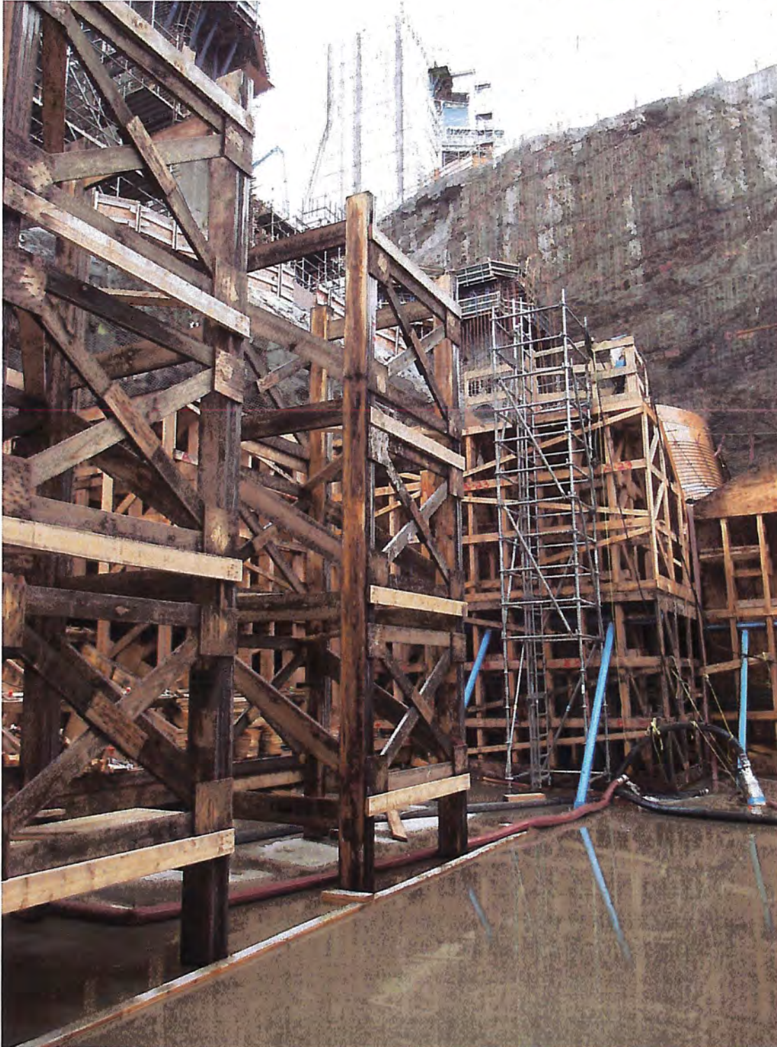
Unit 3 - Installed shoring tower weathering
