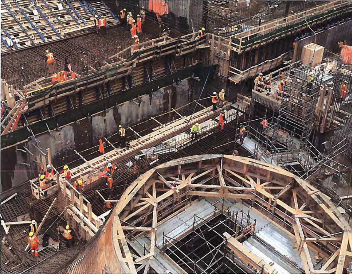
Unit 2 draft tube - View from North West corner of unit, looking below
