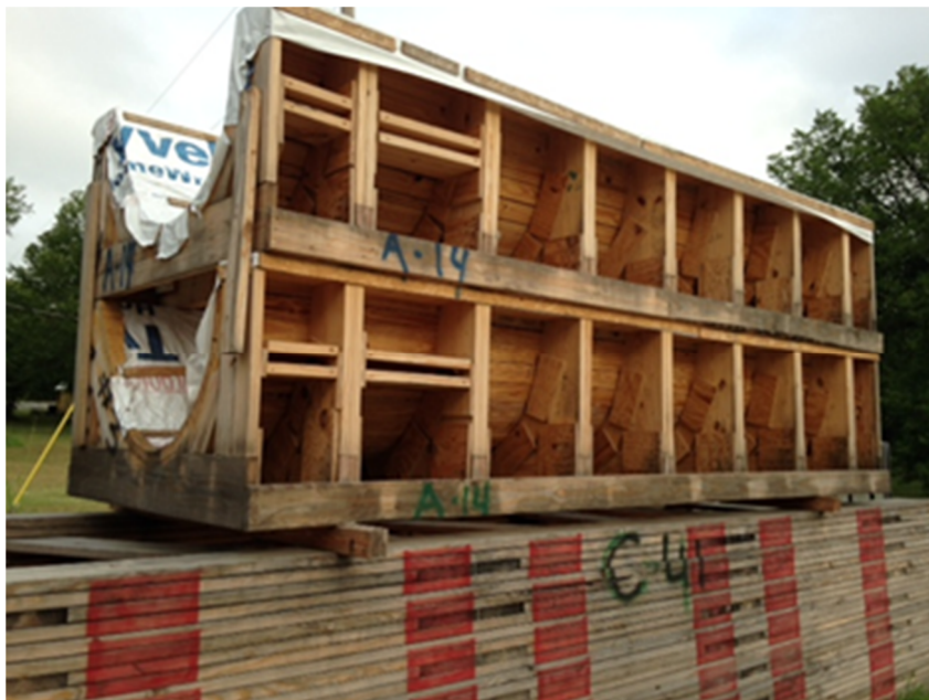
Figure 2: July 23, 2014. Formwork and falsework at CEI facility. Note onset of weathering of wood compared to same material in Figure 1.
