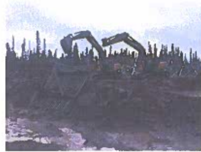
S1-70 Leg C, reclamation of grillage footing, saturated founding base and backfill
