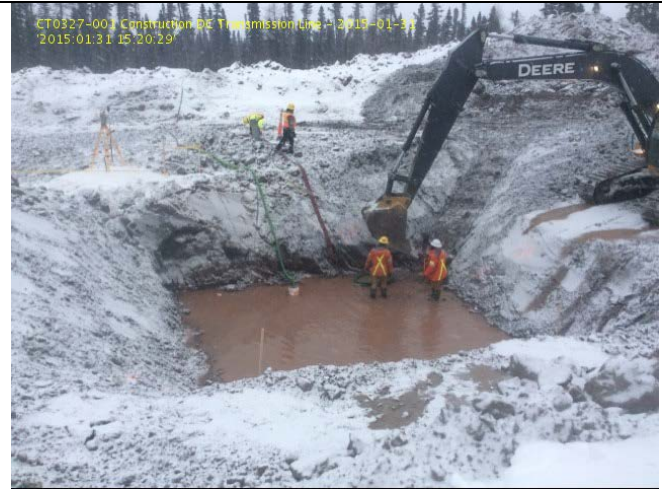
Photo 4: S1-70 Leg D excavation works with inefficient ground water control.
