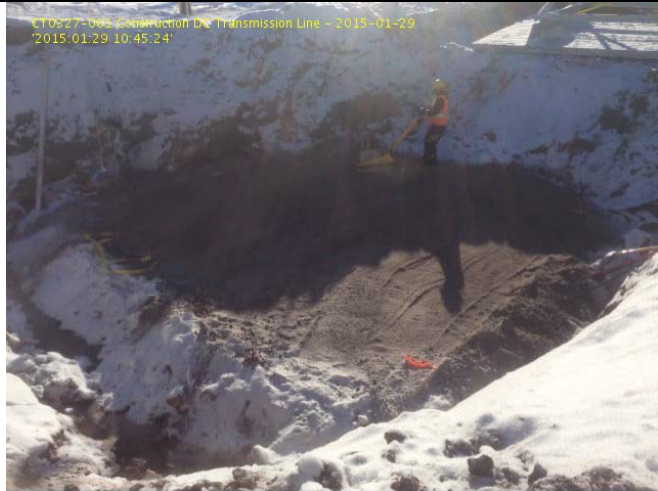
Photo 1: S1-70 Leg A Re-work on base preparation exposed to frost, compaction effort with no verification of test data.
