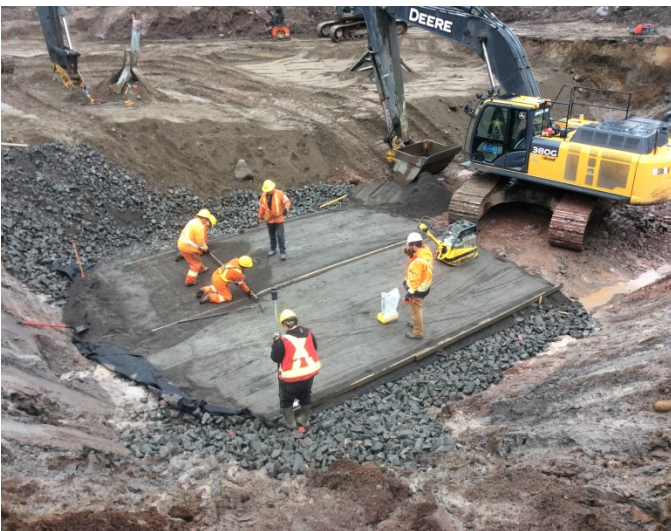
Photo 11: S1-70, Leg D, Grillage placement on prepared founding base with groundwater control.
