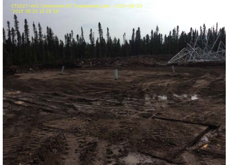
Photo 12: S1-70 completed reinstallation of foundations, general view looking Southeast. Proper grading however no additional mounding.
