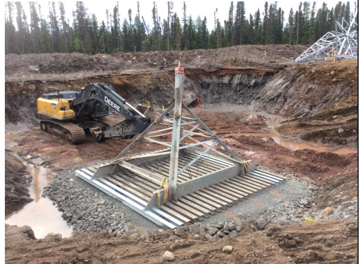
Photo 10: S1-70, Leg A, Grillage Placement on prepared founding base with groundwater control.
