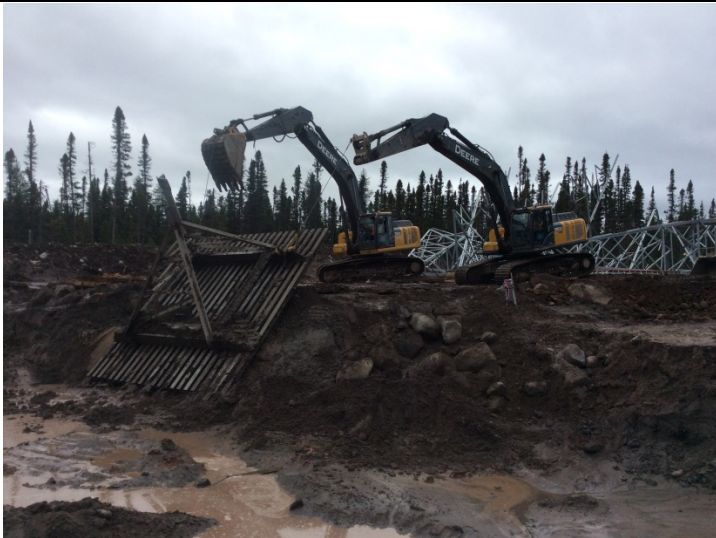
Photo 7: S1-70 Leg C, reclamation of grillage footing, saturated founding base and backfill.
