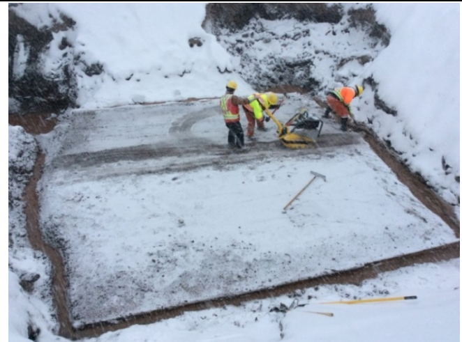
Photo 2: S1-70 Leg B Founding base preparation and compaction effort with no verification of test data.
