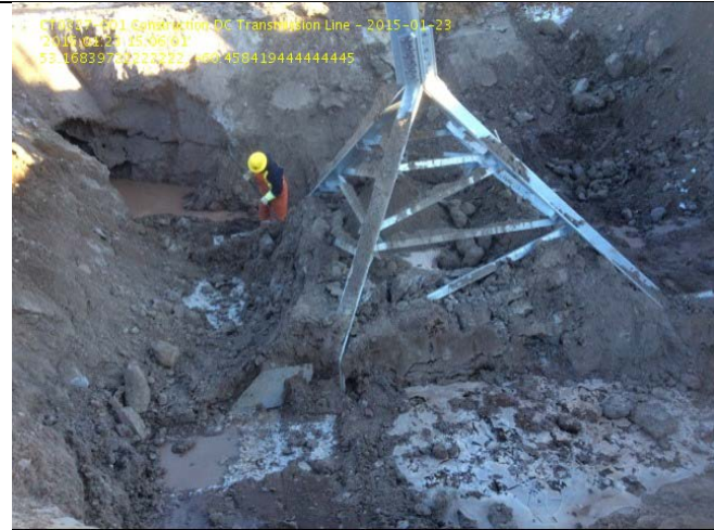
Photo 3: S1-70 Leg C– Reclaim of grillage during initial installation. Frozen founding base and frozen backfill with oversized boulders.
