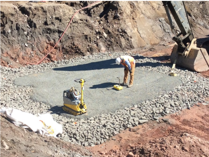
Photo 9: S1-70, Leg A, Groundwater control, found base preparation and compaction effort verification.
