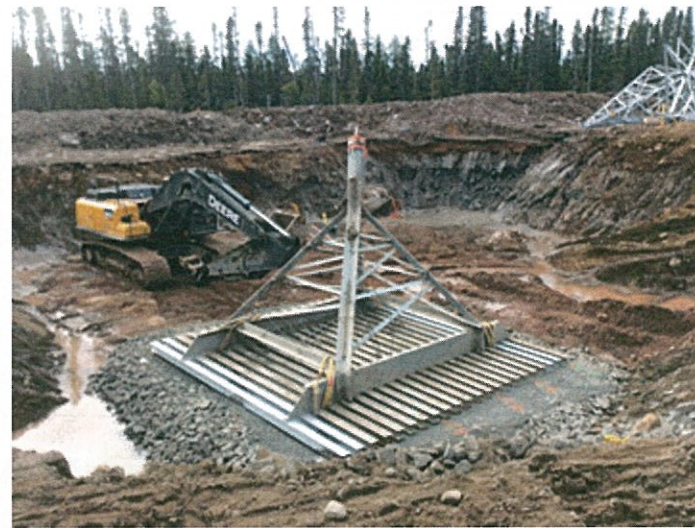
S1-70, Leg A, Grillage Placement on prepared founding base with groundwater control.
