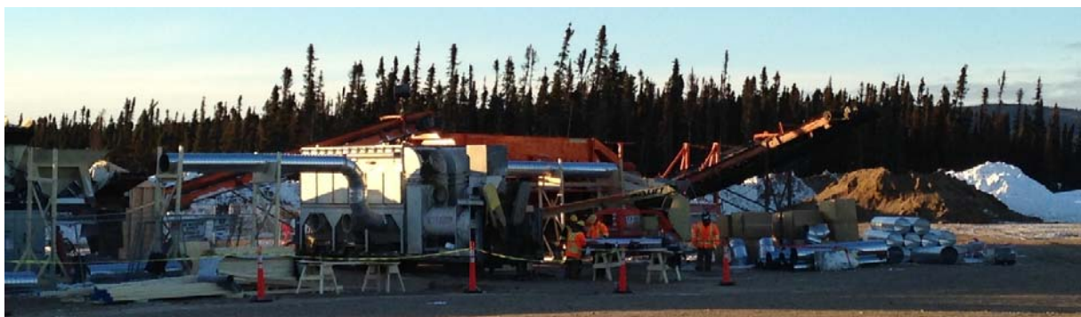
Figure 24: Crusher, dust suppression system – February 2014
