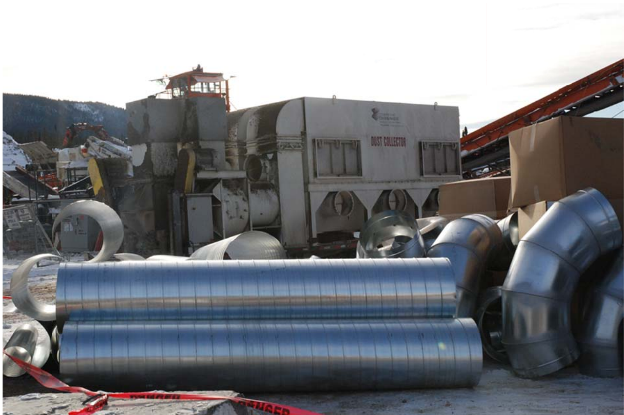
Figure 23: Crusher, dust suppression system – February 2014
