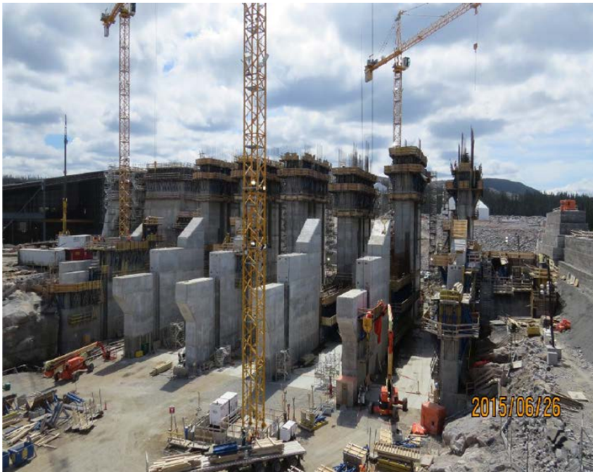
Progress on the Spillway at the Muskrat Falls Site - June 26, 2015 [NTD: NALCOR Can we get more recent picture?]
