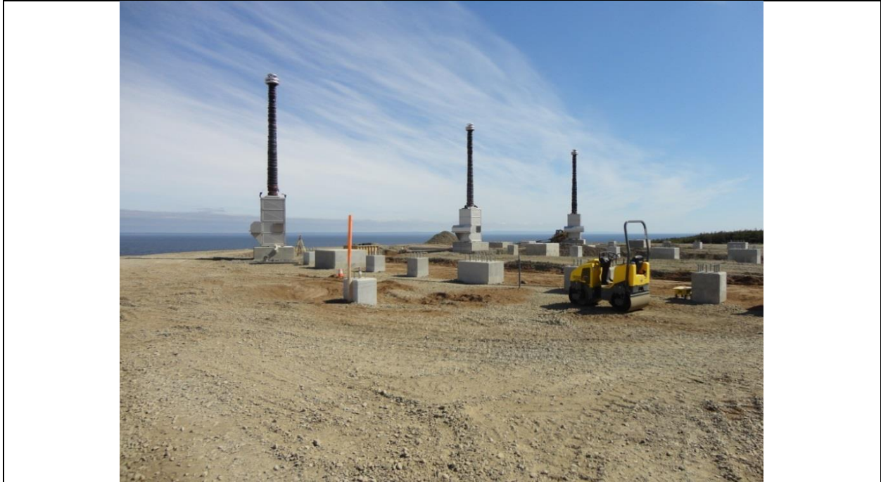
Photo B.5: Transition compound - buried land cables termination points. (July 12, 2016)
