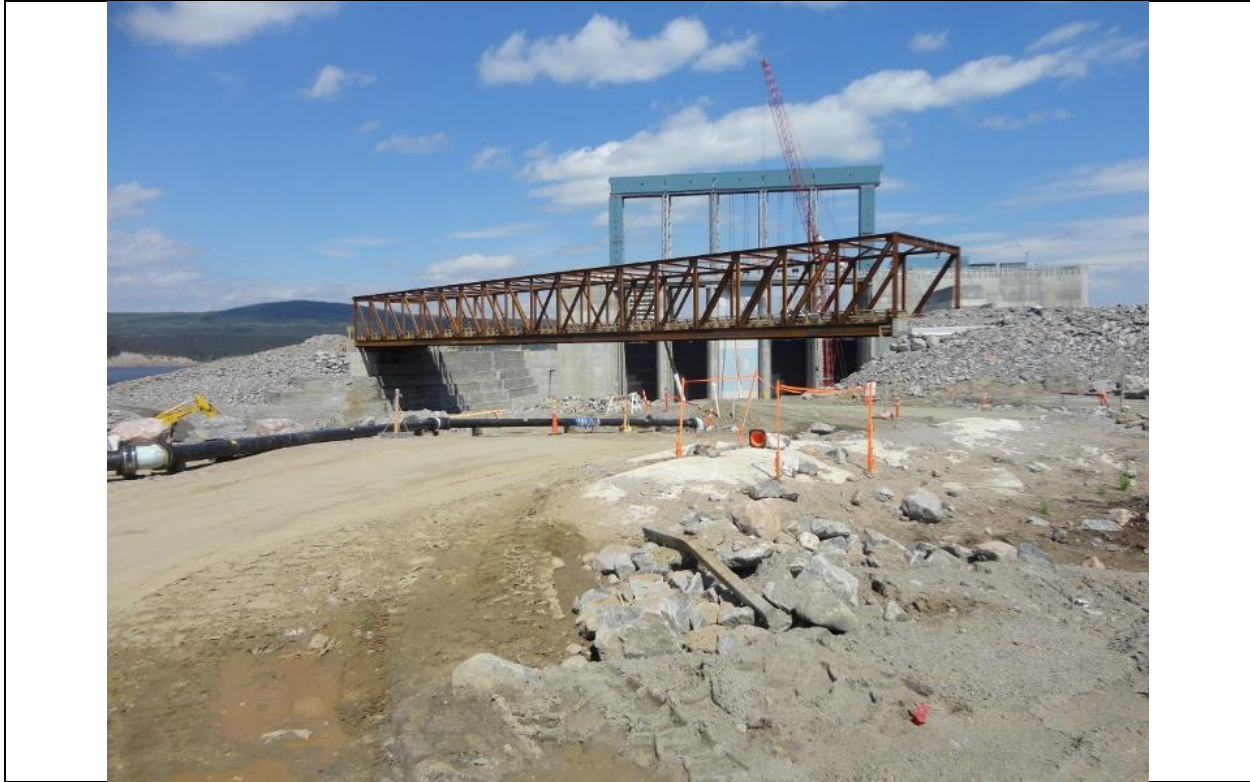
Photo D.9: Spillway intake channel and temporary bridge. View looking downstream. (July 13, 2016)
