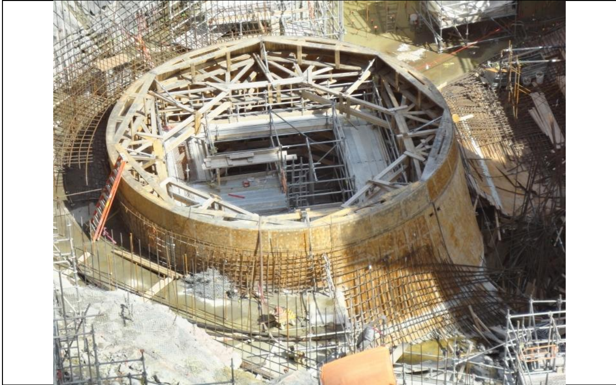
Photo C.11: Unit 2, note collapsed formwork in pyramidal shaped are on right side. (July 13, 2016)
