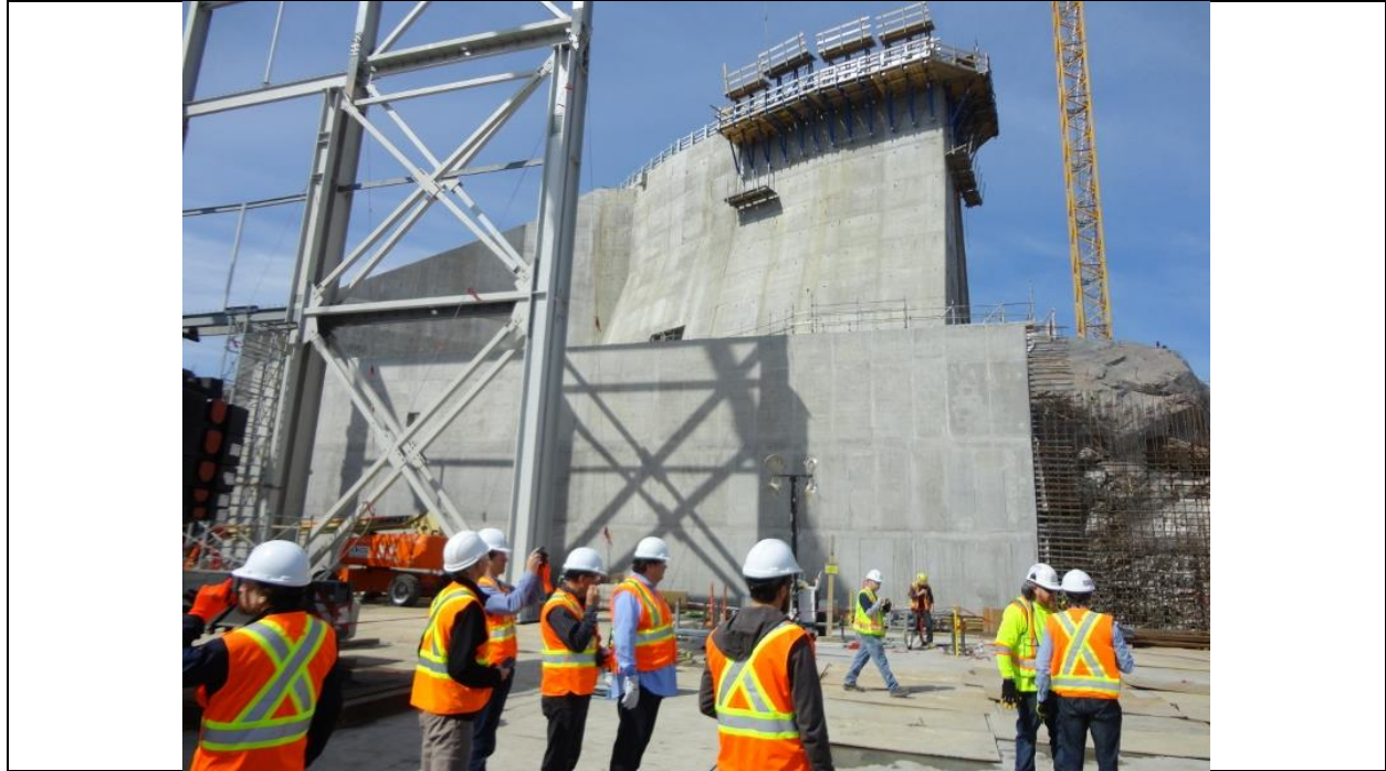
Photo C.16: Powerhouse south service bay with a view towards Central Transition Dam. (July 13, 2016)
