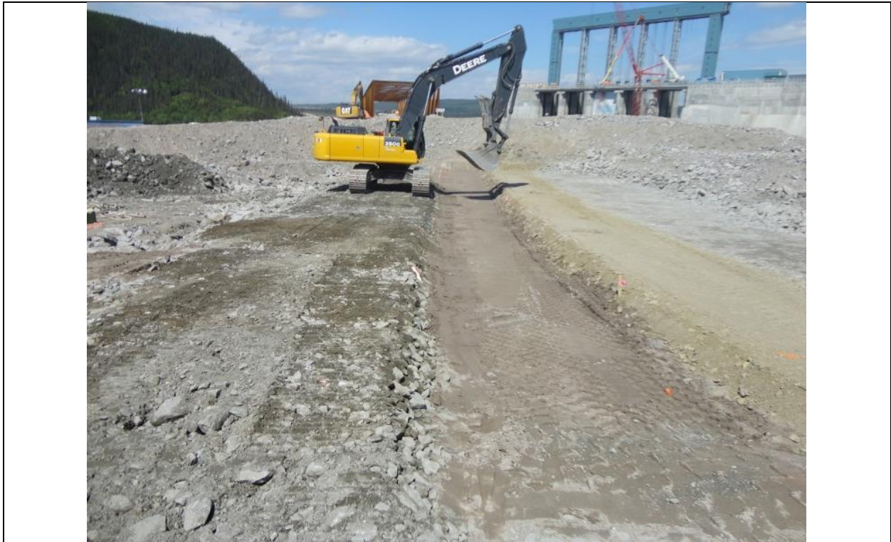
Photo F.5: Intake Diversion Dam. Compacted impervious till core and adjacent transition/filter zones are visible. (July 14, 2016)
