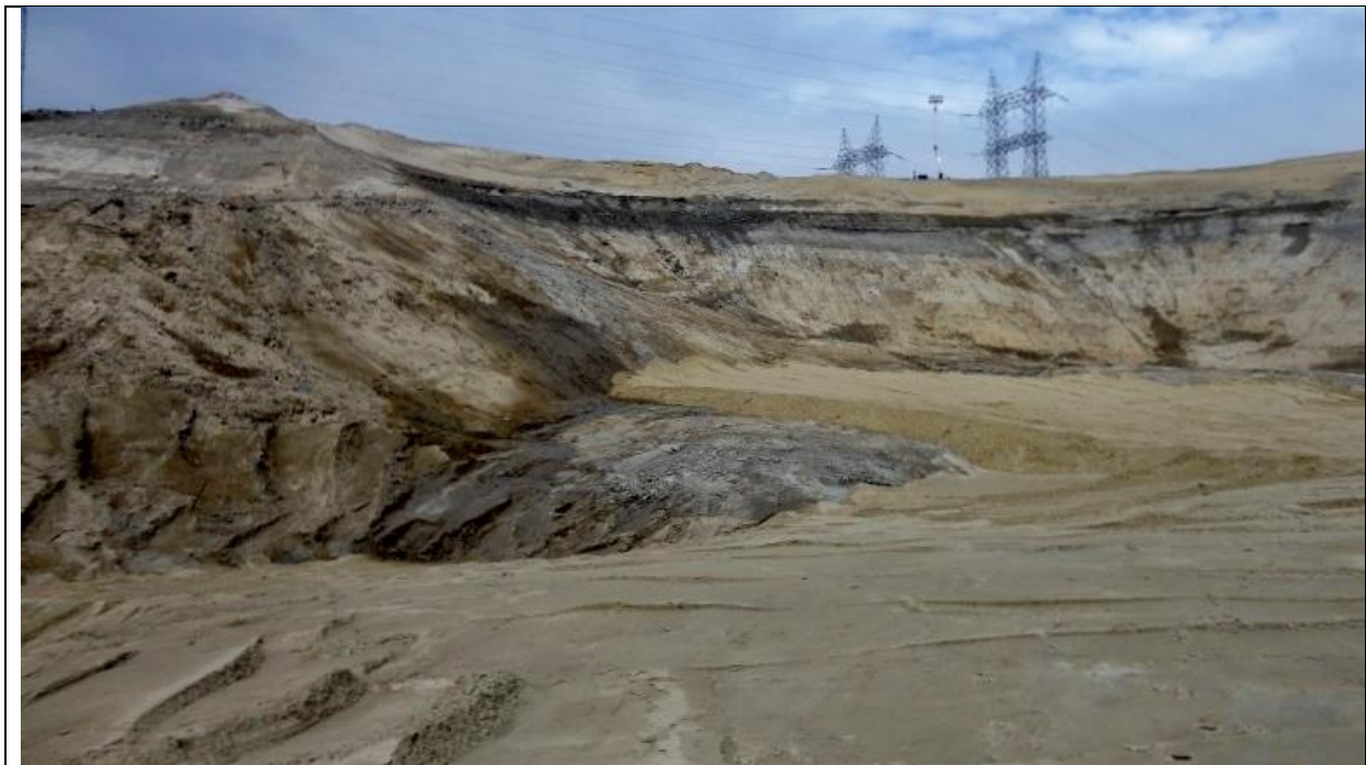
Photo E.4: North Spur, upstream slope. Old gully scar near the intersection of the north and upstream cut-off walls. (July 14, 2016)
