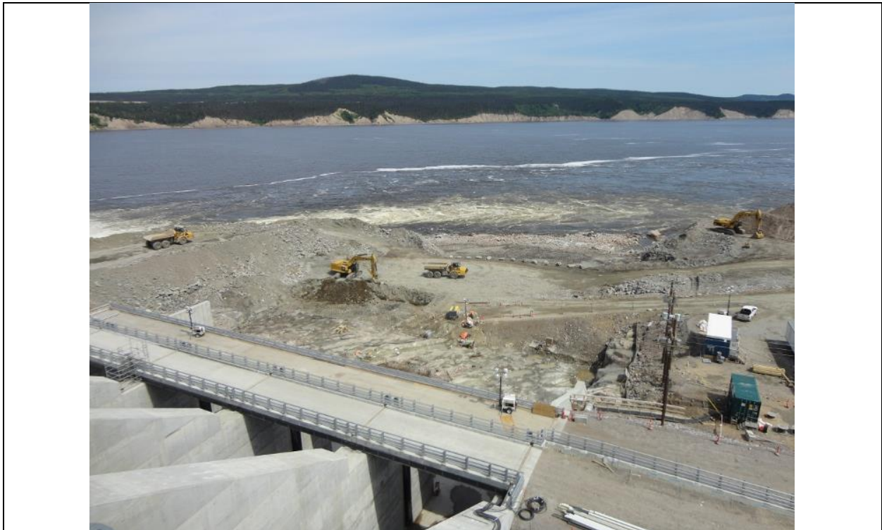
Photo D.12: Spillway apron, removal of cofferdam and preparation of the apron surface. (July 13, 2016)
