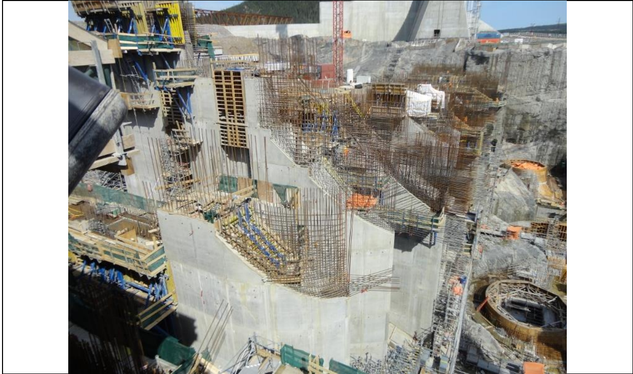
Photo C7: Downstream end of intake piers of Units 1 and 2, view looking north. (July 13, 2016)
