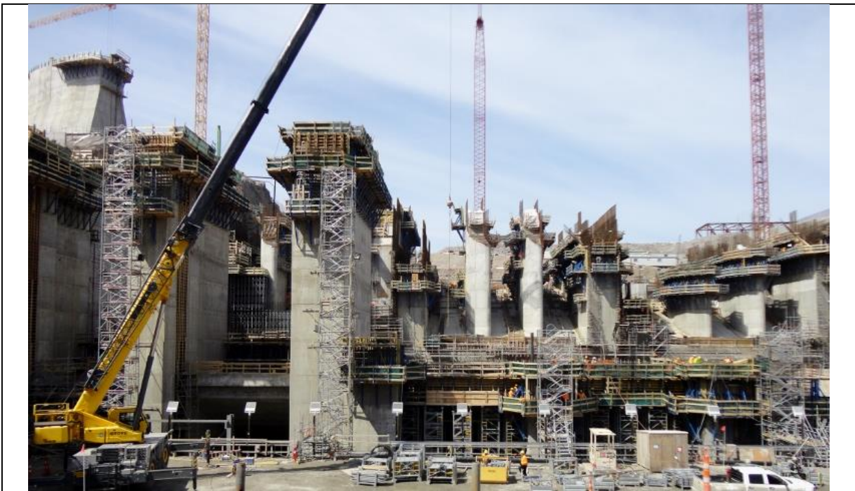
Photo C.4: Units 1, 2 and 3, view looking upstream. (July 13, 2016)
