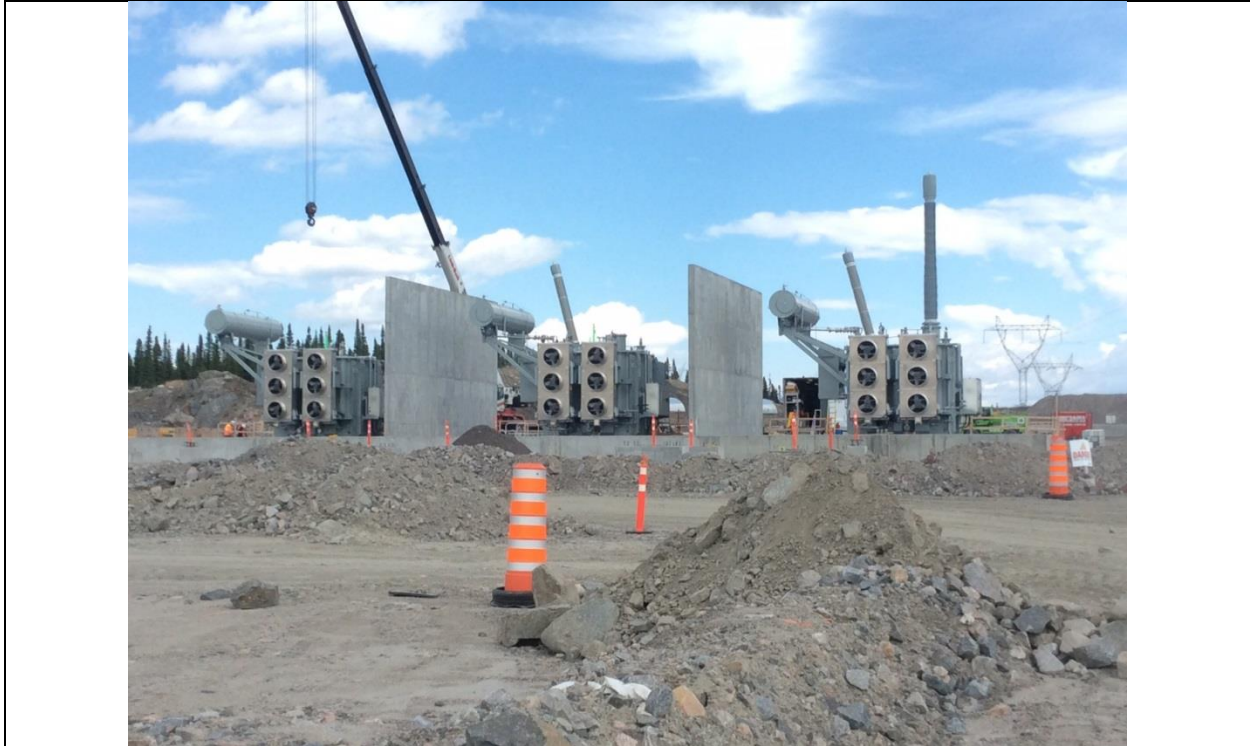
Photo H.3: Transformers already installed on concrete pads within containment pits complete with fire walls. (July 14, 2016)
