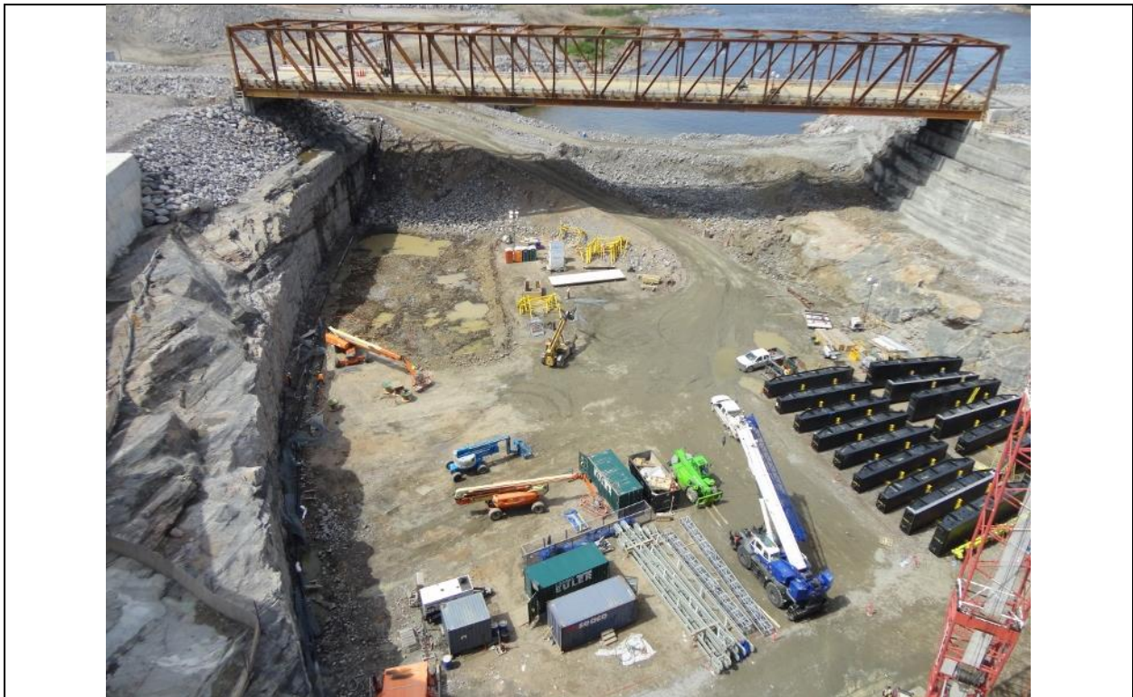
Photo D.8: Spillway intake channel and temporary bridge. View looking towards upstream. (July 13, 2016)
