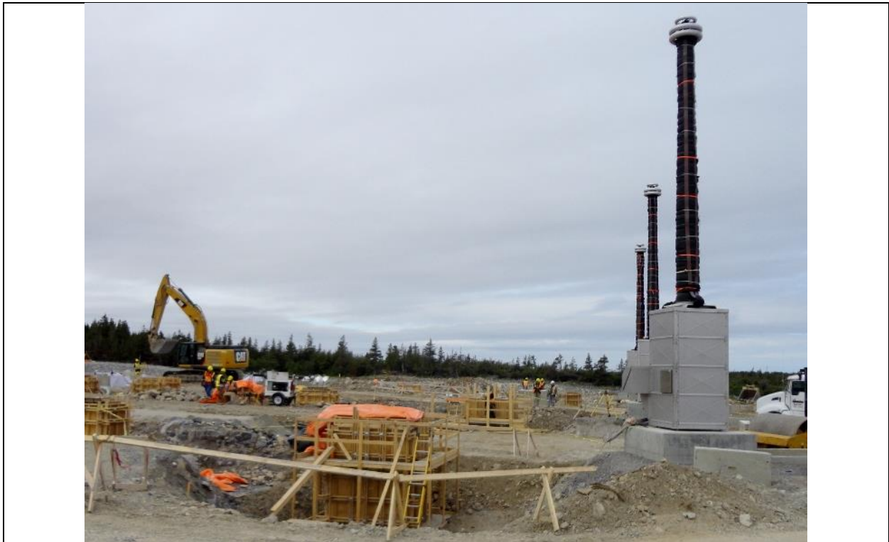
Photo A.12: Shoal Cove Transition compound – buried land cables termination points. (July 12, 2016)
