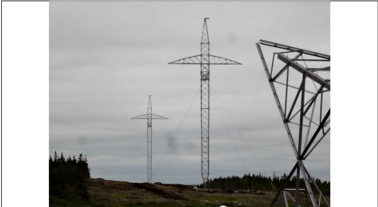
Photo A.9: DC transmission towers immediately east of the Shoal Cove facilities. (July 12, 2016)
