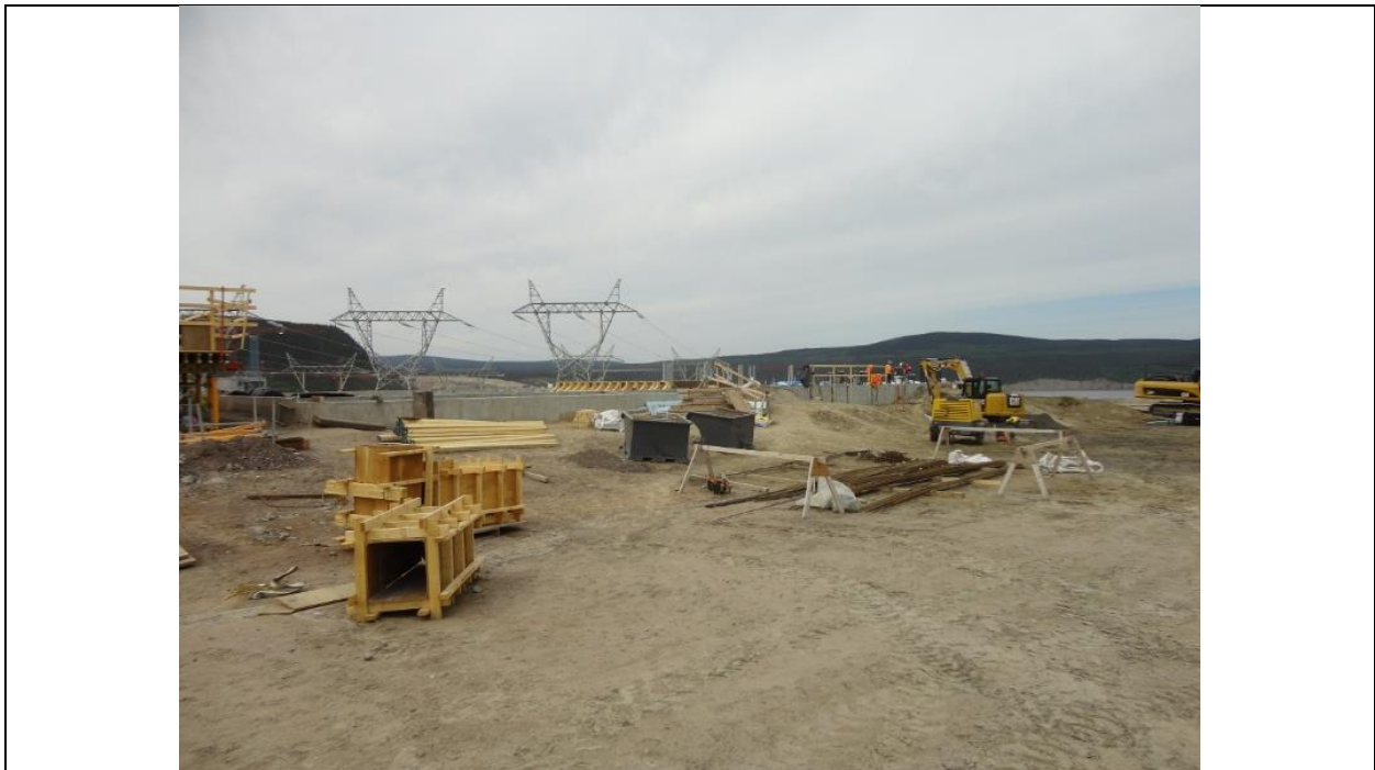
Photo G.6: Control building foundations ready for the pre-engineered building erection. (July 13, 2016)
