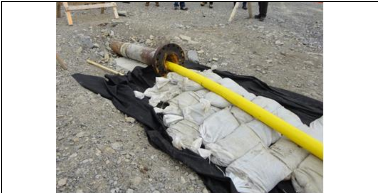
Photo A.2: Cable No. 1 at Shoal Cove; exit from the inclined borehole on the Shoal Cove shore. (July 12, 2016)
