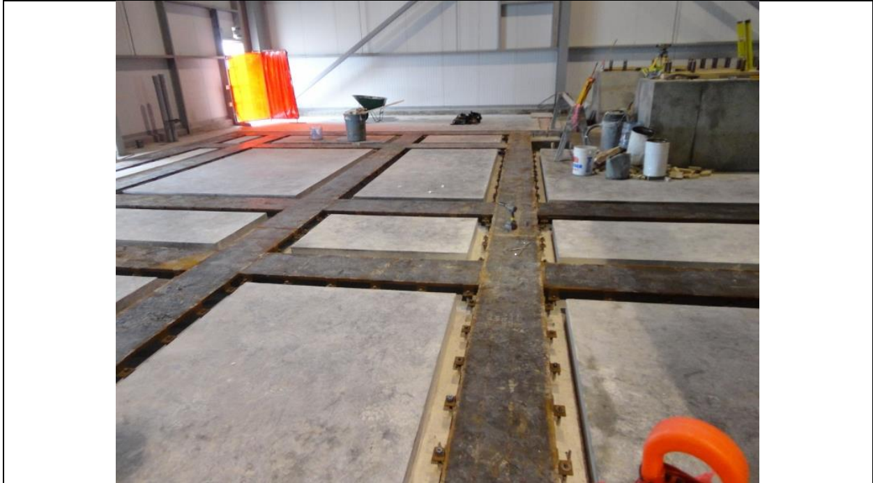
Photo I.15: Soldiers Pond – Close-up of embedment plates at unit 1 bay, ready for grouting. (July 15, 2016)
