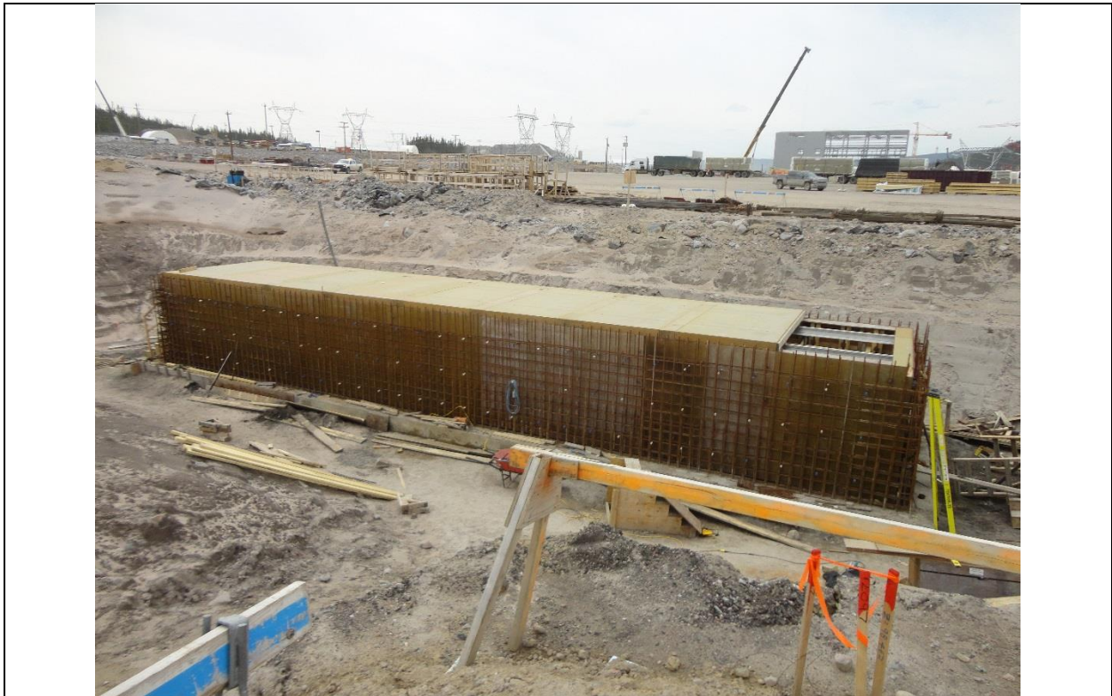
Photo G.2: Converter station oil / water separator – work ongoing on reinforcement and formwork erection. (July 13, 2016)
