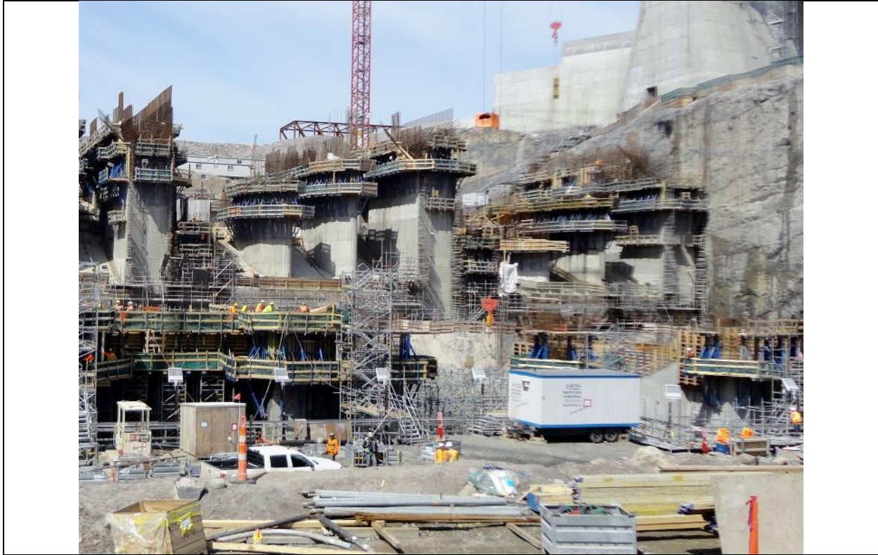
Photo C.5: Units 3 and 4, view looking upstream. (July 13, 2016)
