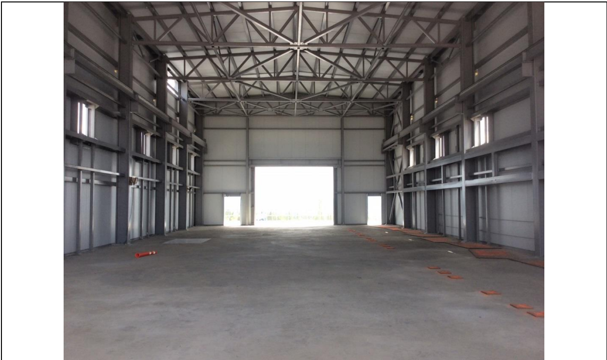
Photo H.6: Interior view of GIS Building. (July 14, 2016)
