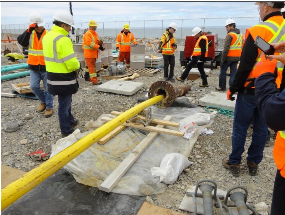
Photo A.4: Cable No 2 emerging from the casing of the inclined borehole. (July 12, 2016)
