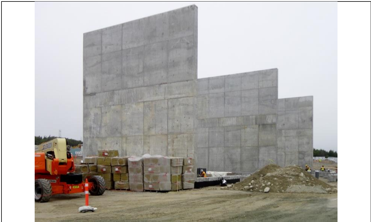
Photo I.4: Soldiers Pond Converter Transformers fire walls. (July 15, 2016)
