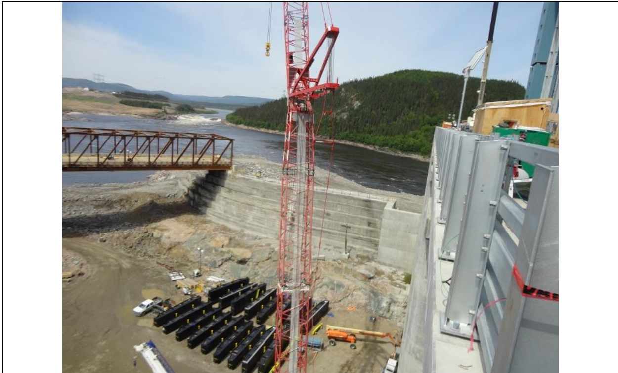
Photo D.10: Left side of the spillway intake channel. Note the black stop log segments stored on the bases of the channel in the foreground. (July 13, 2016)
