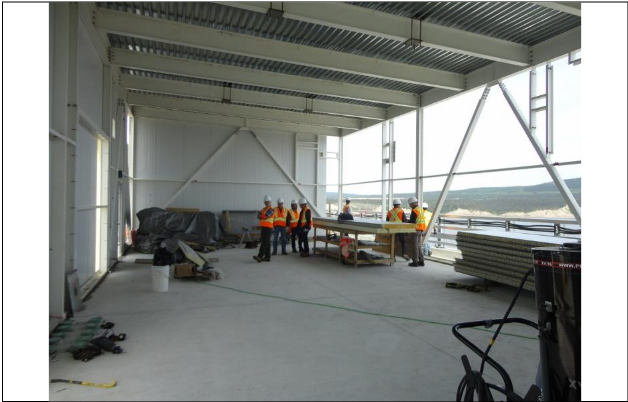
Photo D.6: Control room on top of the spillway gate structure. (July 13, 2016)
