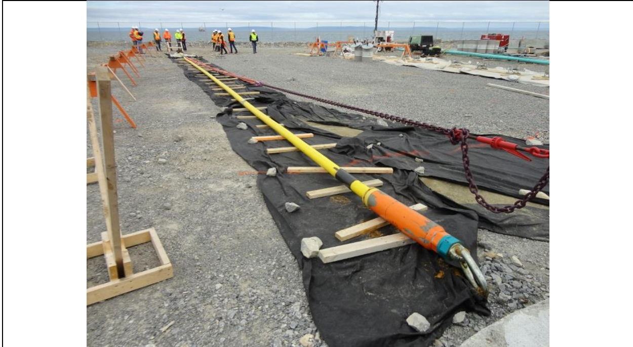
Photo A.1: Land end of Cable No. 1 on the Shoal Cove shoreline. (July 12, 2016)
