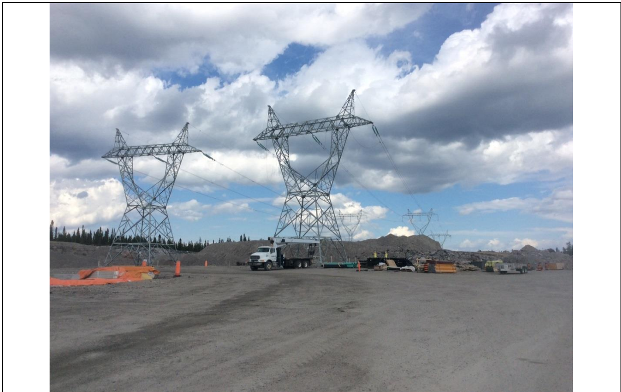
Photo H.8: Dead-end towers of the HVAC 315 kV transmission line at the line's entrance into the Switchyard. (July 14, 2016)
