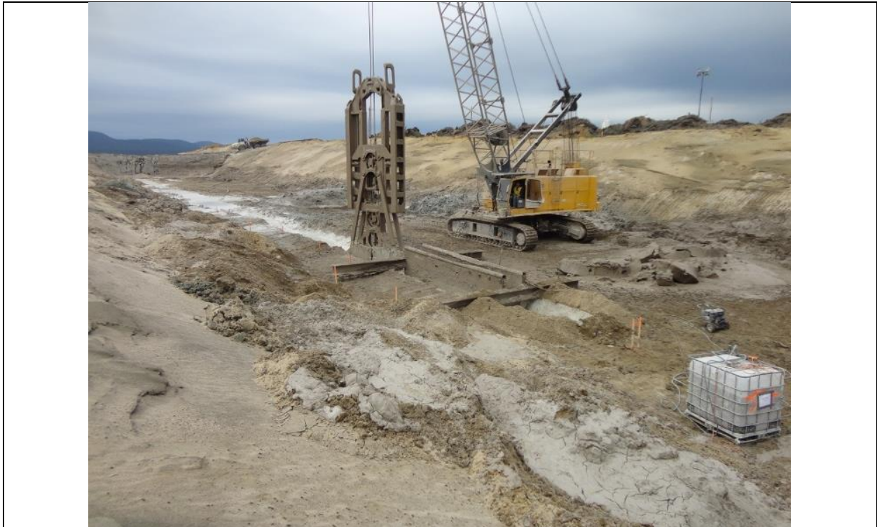
Photo E.14: Excavation of the North Cut-off, in the area east of the road crossing. (July 14, 2016)
