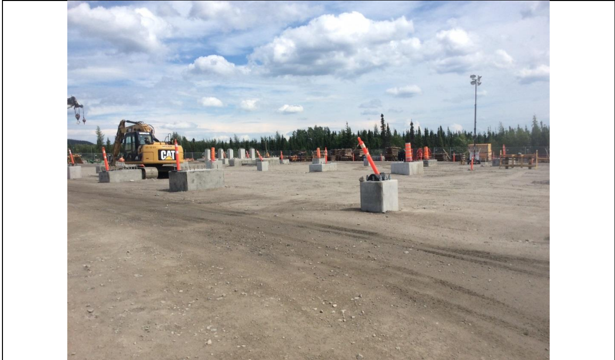
Photo H.9: Extension of the new Switchyard for interconnection to the existing Churchill Falls Switchyard. (July 14, 2016)
