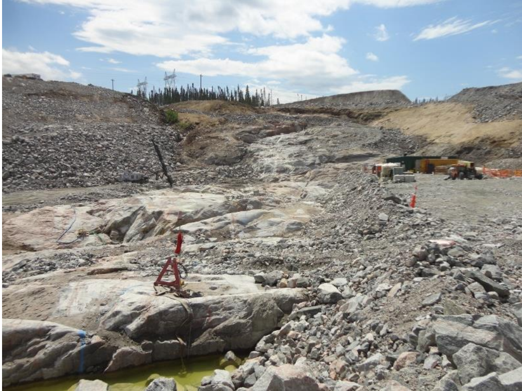
Photo F.1: South Dam foundations, cleaned granitic gneiss rock along the impervious core footprint. View looking south up the abutment. Note the irregular surface. (July 14, 2016)
