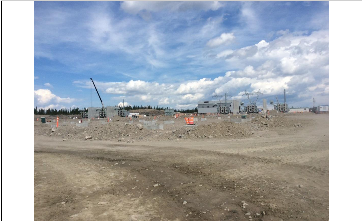
Photo H.1: Overall view of Switchyard with installed transformers and GIS Building on background. (July 14, 2016)
