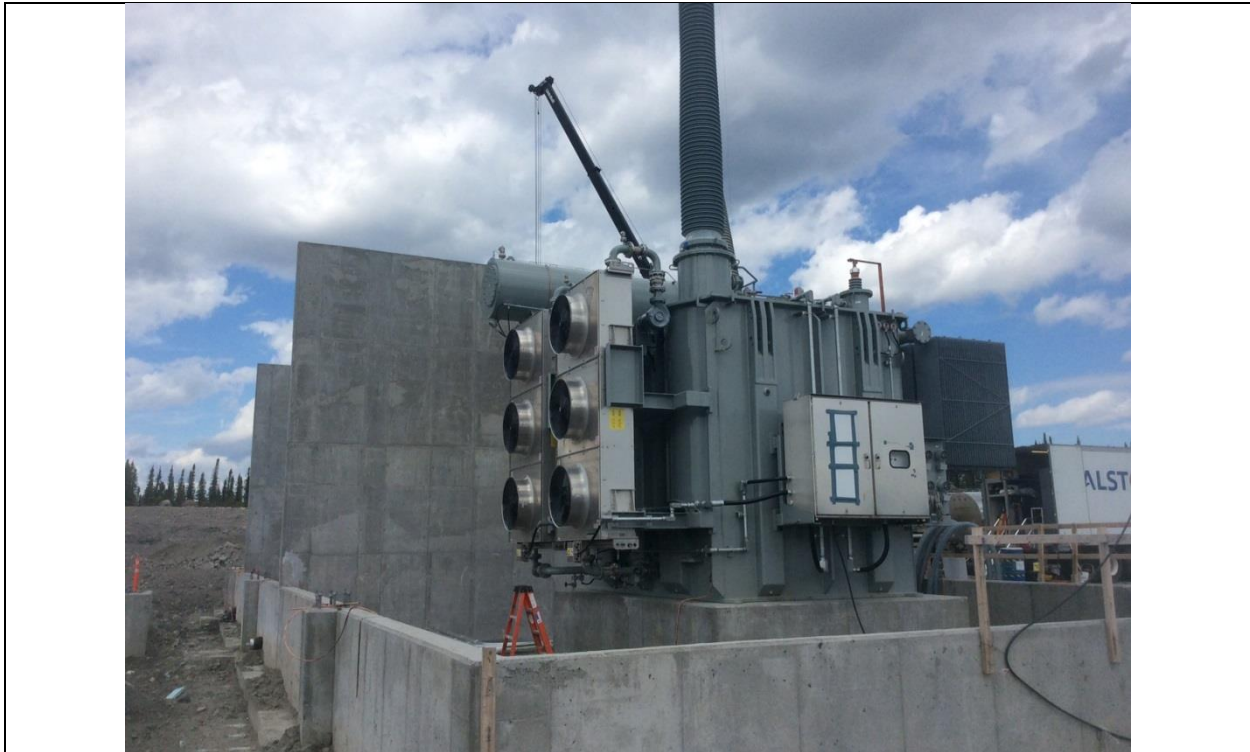
Photo H.4: Close-up of assembled transformer. (July 14, 2016)
