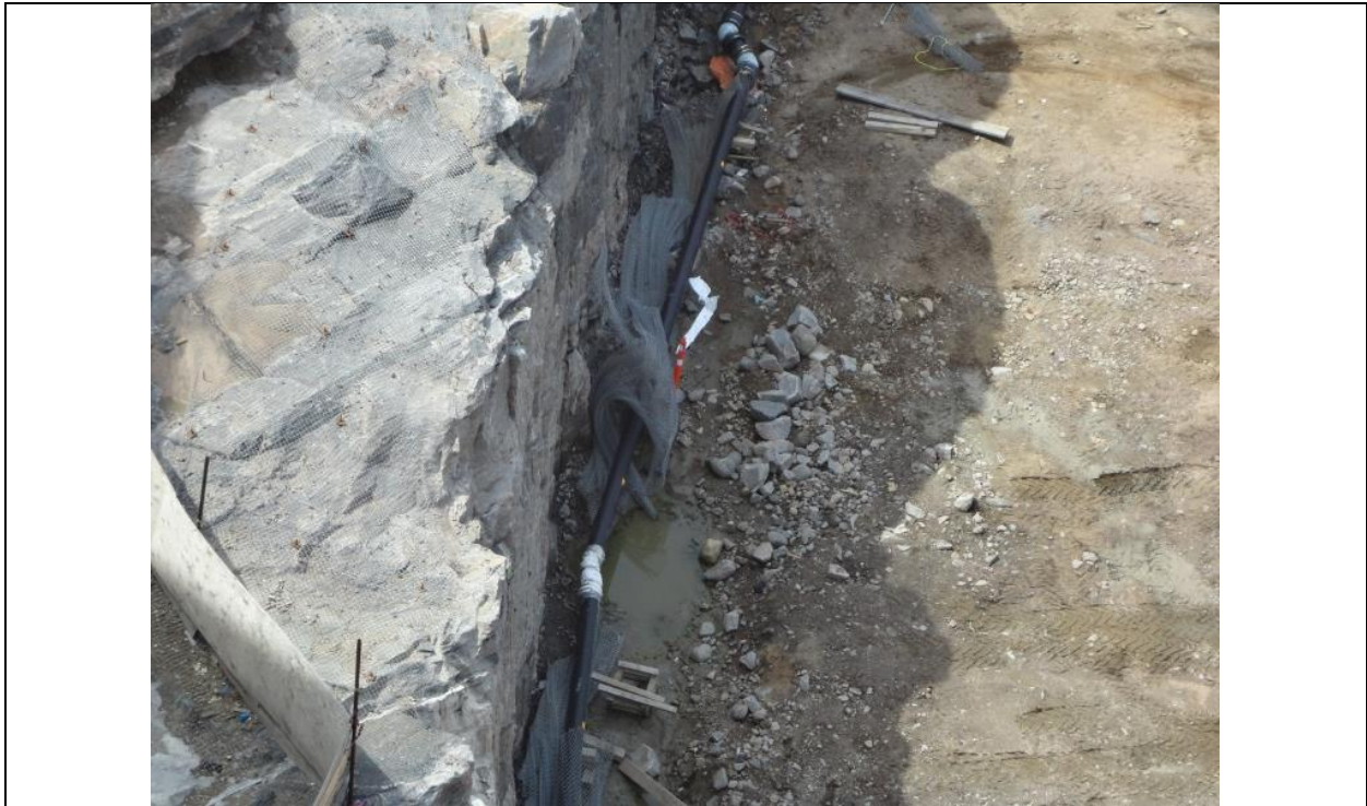
Photo D.11: Spillway approach channel. Removal of steel mesh from the left side rock face. (July 13, 2016)
