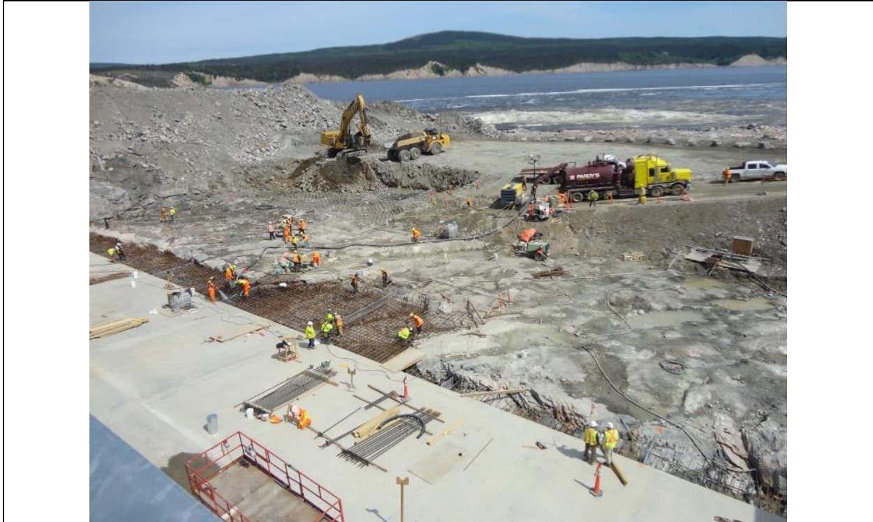
Photo D.13: Spillway apron, removal of cofferdam and preparation of the apron surface. Steel reinforcement mats are being placed in rock depressions adjacent to the concrete apron, in preparation for placement of dental concrete. (July 13, 2016)
