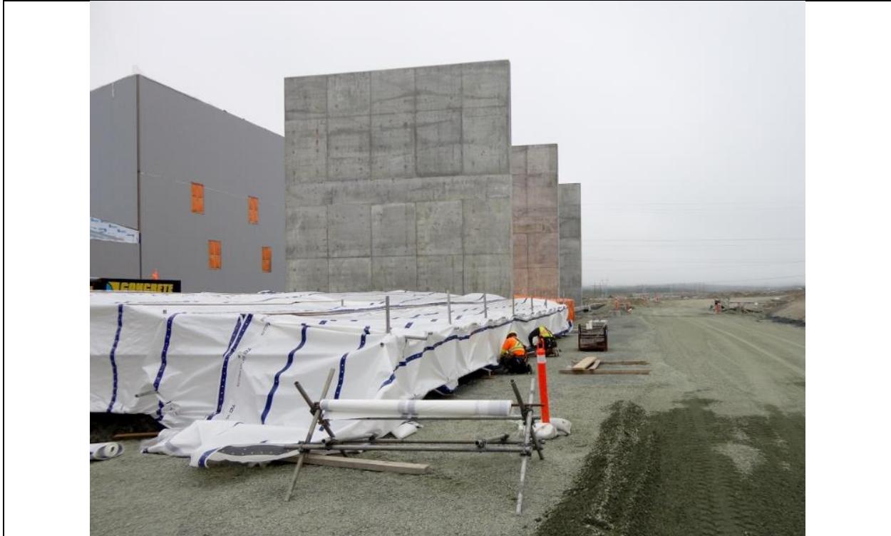
Photo I.5: Soldiers Pond – Converter transformer containment pit covered for curing the finished protective coating of the pit floor and walls. Separation fire walls and Converter Station on the background. (July 15, 2016)
