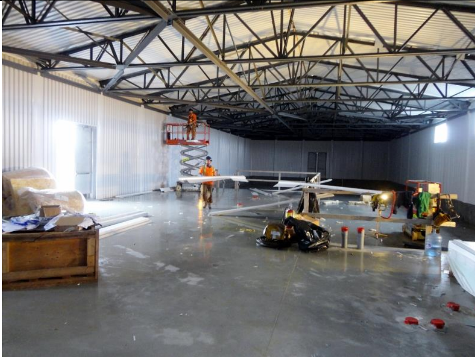
Photo I.11: Soldiers Pond – Interior view of Control Building. (July 15, 2016)
