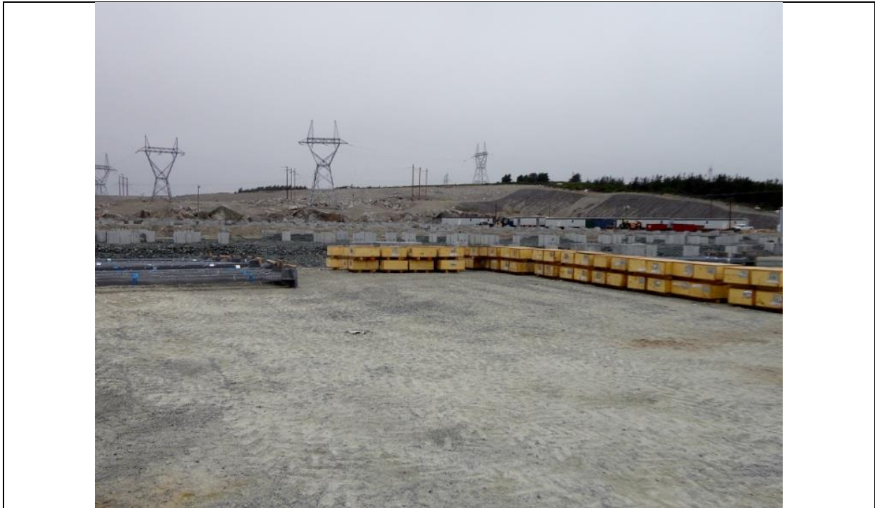
Photo I.9: Soldiers Pond – AC switchyard with completed gantry and posts foundations. Structural steel members and boxes with equipment stored on site and ready for installation. (July 15, 2016)
