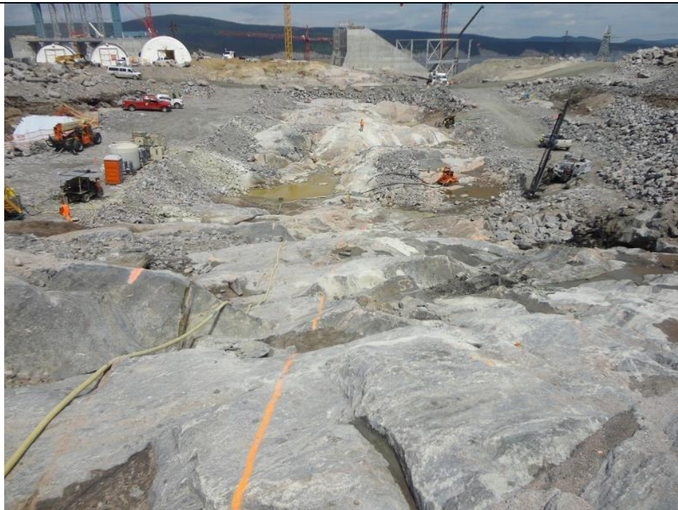
Photo F2: South Dam foundation, cleaned rock along the impervious core footprint. View looking north down the abutment. (July 14, 2016)
