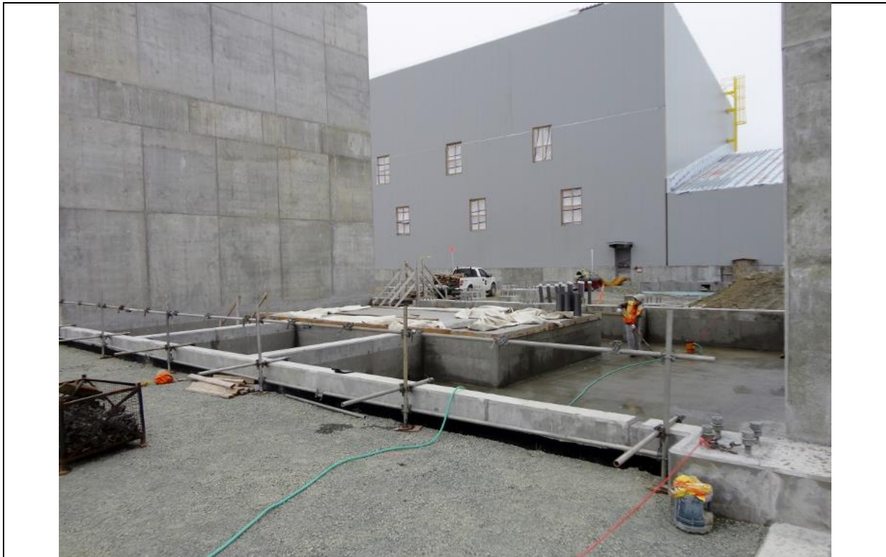
Photo I.6: Soldiers Pond – Converter transformer pad, fire walls and containment pit in preparation for final protective coating application. (July 15, 2016)
