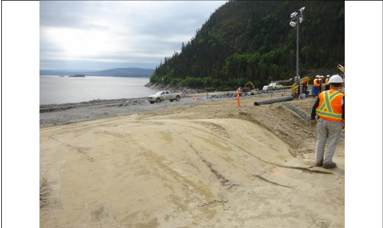
Photo E.13: Excavation and fill placement for finger drain at the south end of the downstream slope. (July 14, 2016)
