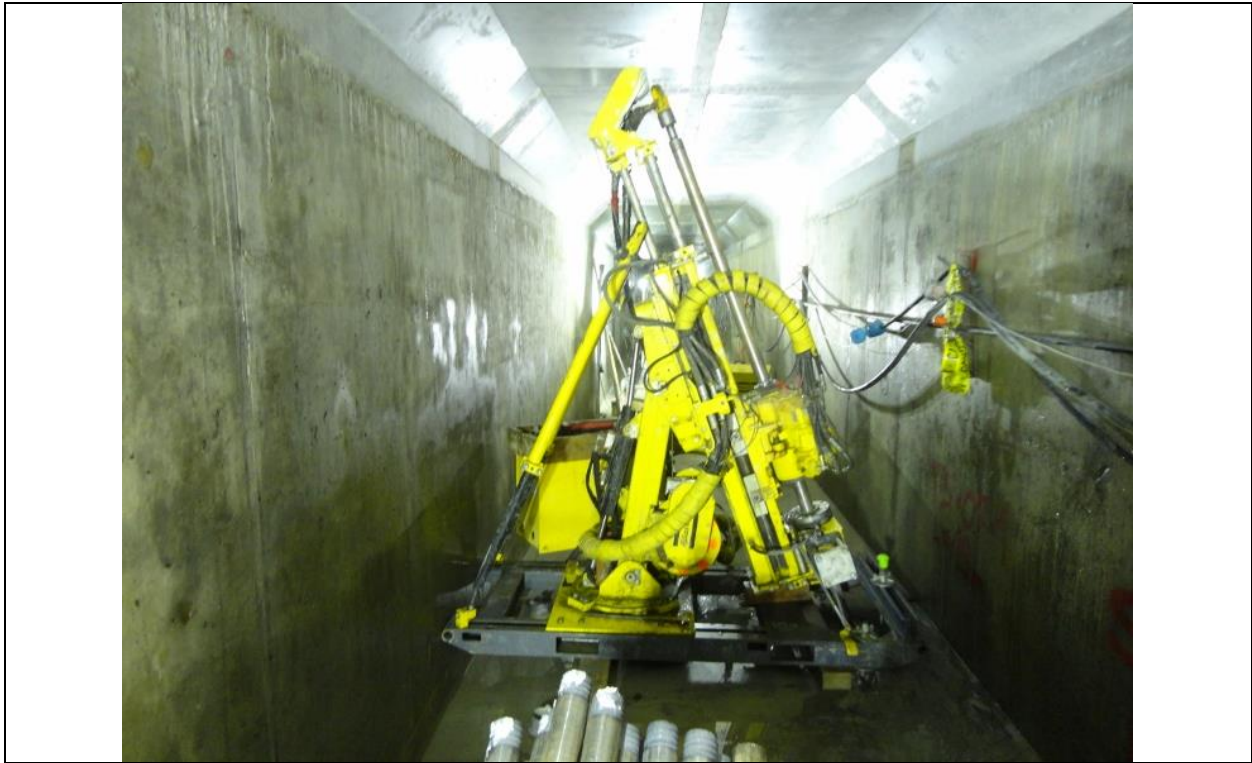
Photo F.7: Powerhouse Intake grouting gallery. Drill rig boring cored, inclined grout holes. (July 14, 2016)
