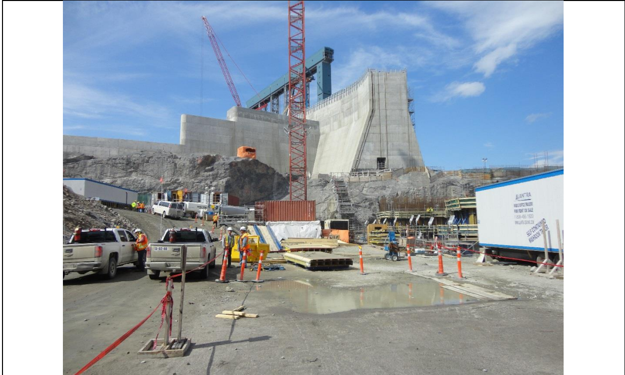
Photo D.3: South side of spillway, Powerhouse/Transition dam shown on the right. (July 13, 2016)
