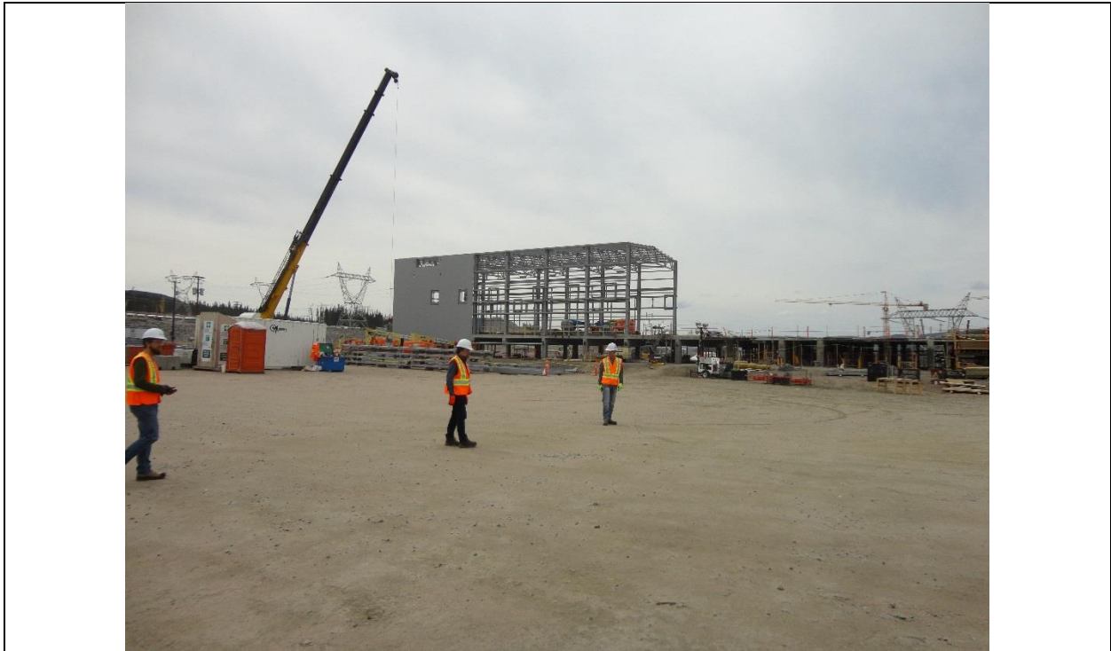
Photo G.3: GIS building- Partially installed structural steel frame. Steel erection will recommence upon completion of foundations (at right) repair work. (July 13, 2016)
