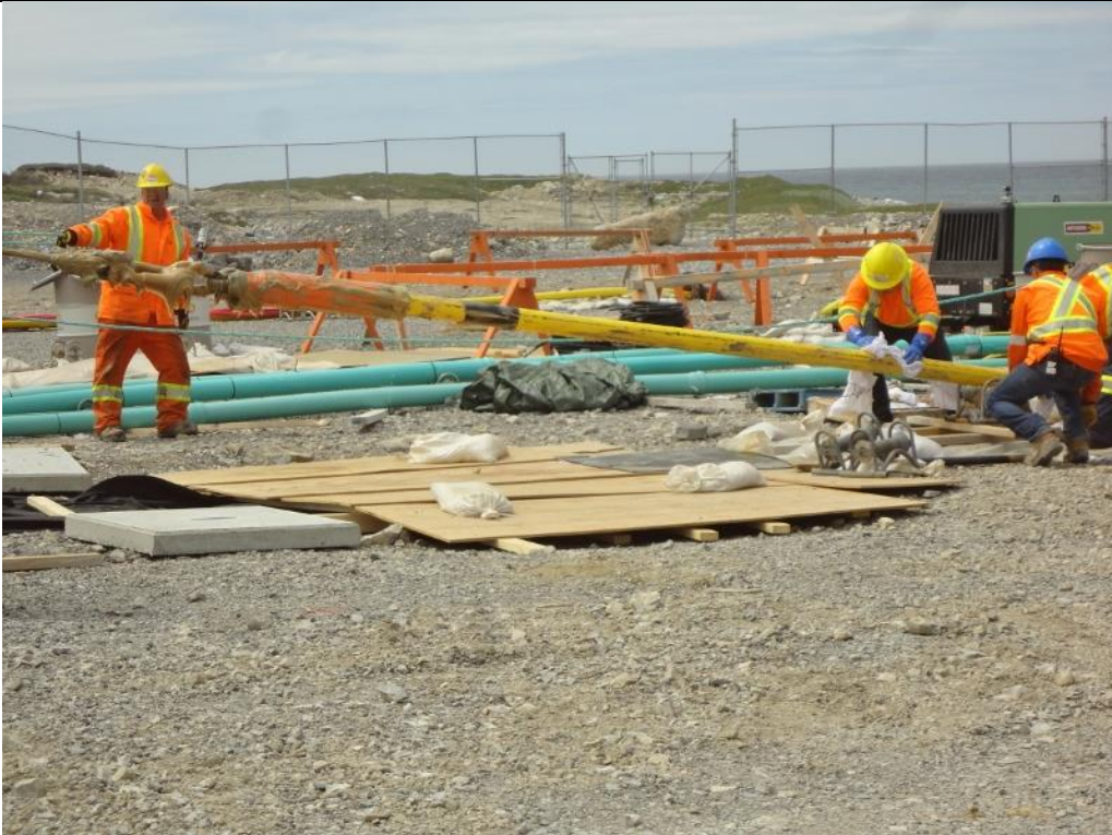
Photo A.3: Cable No 2 emerging from the casing of the inclined borehole. Note coating of lubricant grease. (July 12, 2016)
