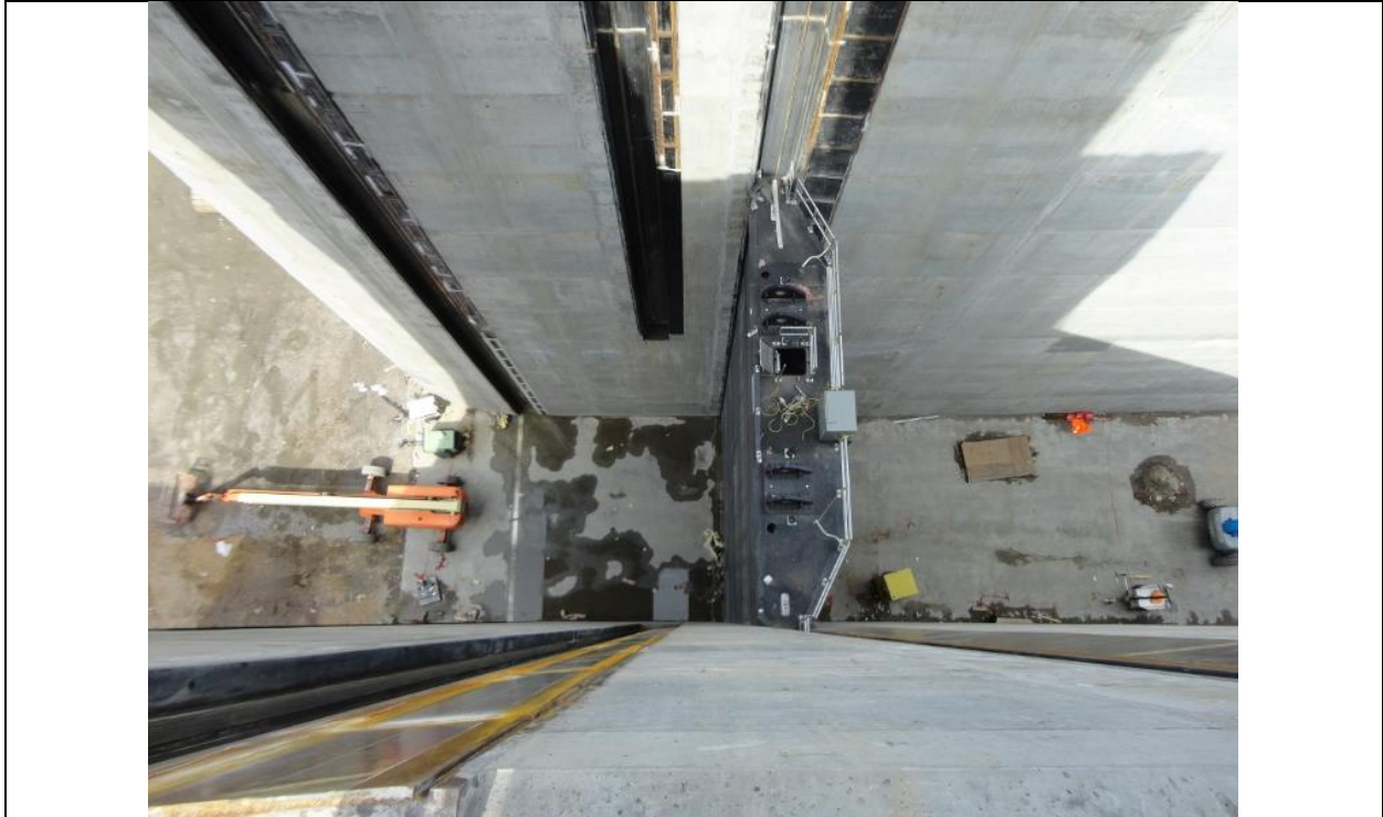
Photo D.7: Top of gate No. 1, view from the top of the spillway gate structure. (July 13, 2016)
