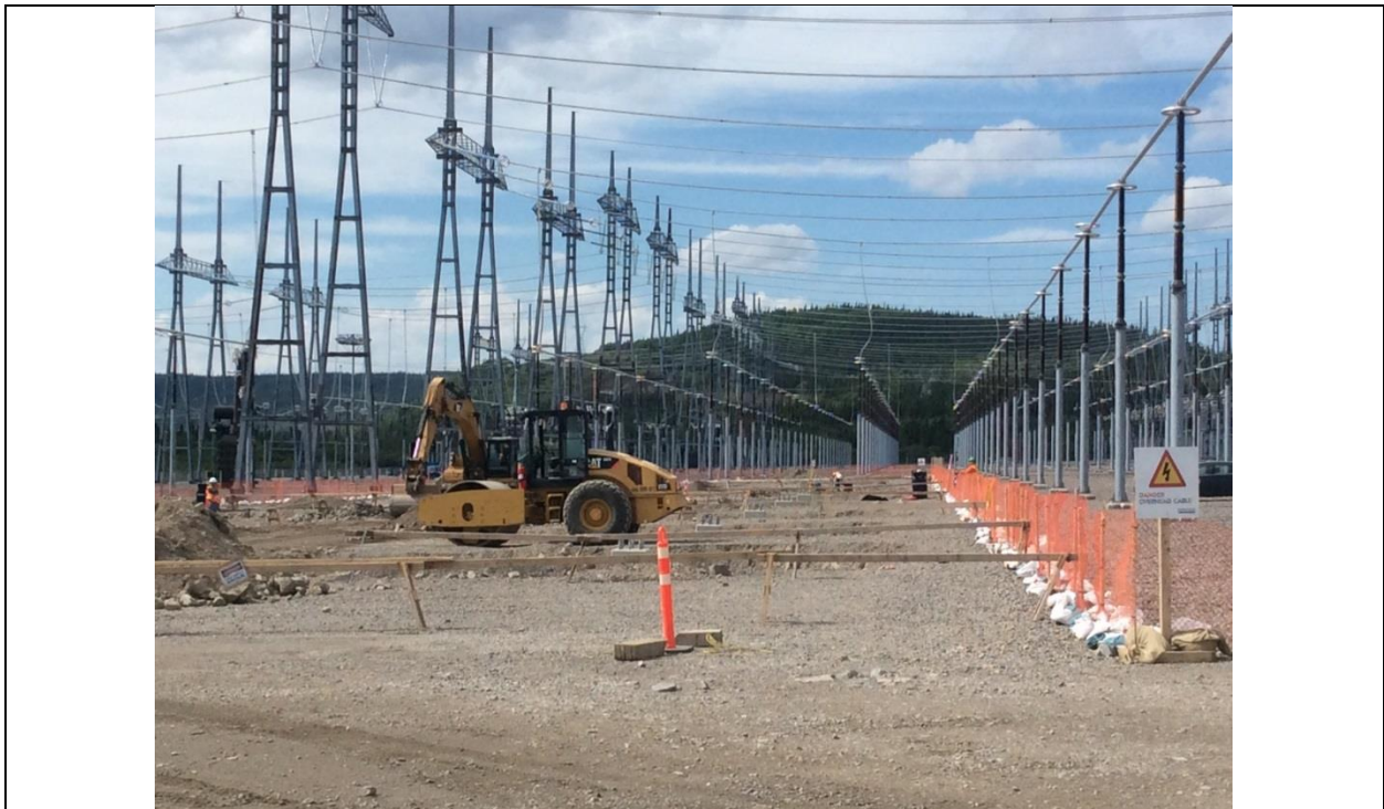
Photo H.10: Newly installed precast footings for bus and equipment supports at interface location between the new and the existing Churchill Falls Switchyards. (July 14, 2016)
