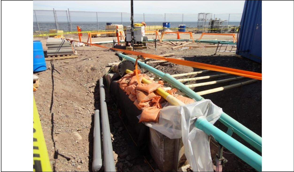
Photo B.1: Cable #1 (yellow cable) at the inclined borehole and anchor point. (July 12, 2016)
