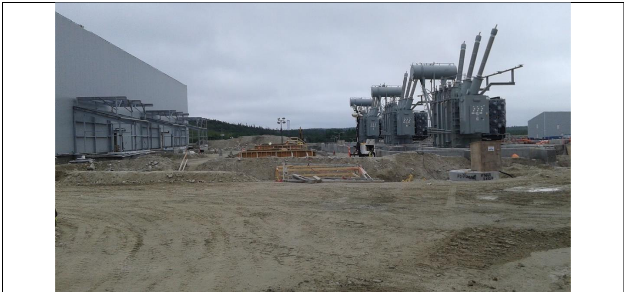
Photo I.16: Soldiers Pond – Synchronous Condensers transformers and the building on the background. (July 15, 2016)
