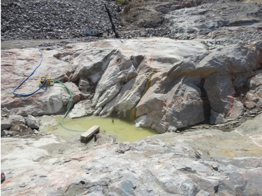
Photo F.3: Irregular granitic gneiss foundation surface. Dental excavation and concrete/mortar backfilling required in many areas. (July 14, 2016)
