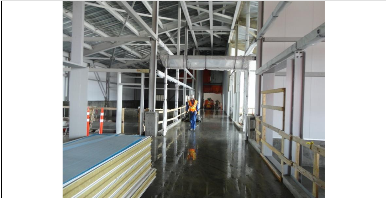
Photo I.3: Soldiers Pond – Converter Station control room interior steel frames and wall panels. (July 15, 2016)
