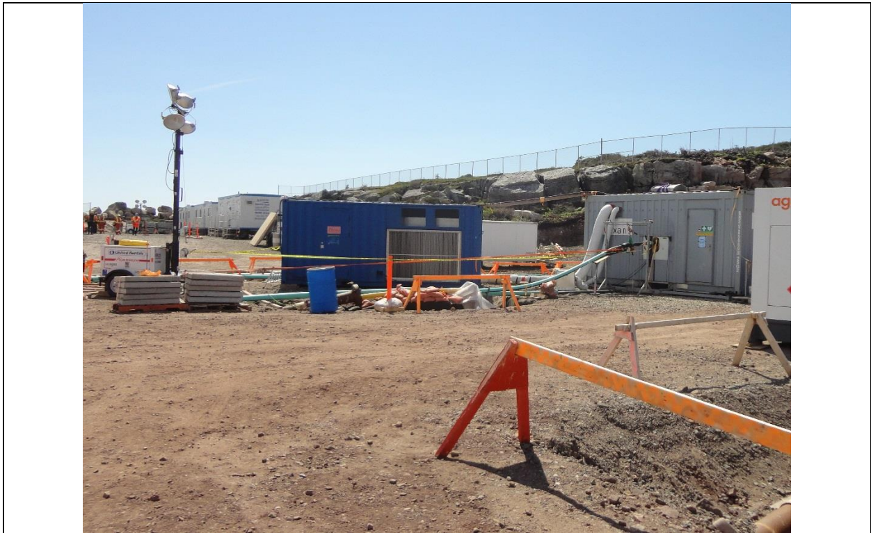
Photo B.2: Cable #1 at the cable jointing facility. (July 12, 2016)
