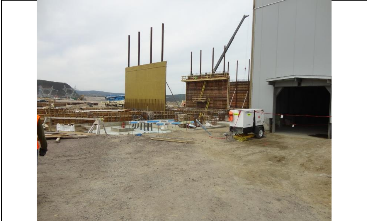
Photo G.1: Muskrat Falls Switchyard – Converter Transformers pads and containment pits with ongoing work on fire walls formwork and reinforcement erection. (July 13, 2016)
