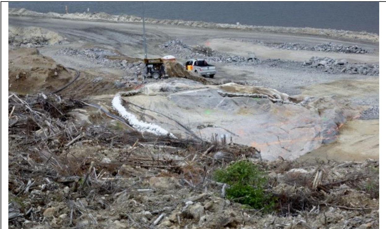
Photo E.6: North Spur, upstream slope. Exposed bedrock at the south end of the slope. (July 14, 2016)
