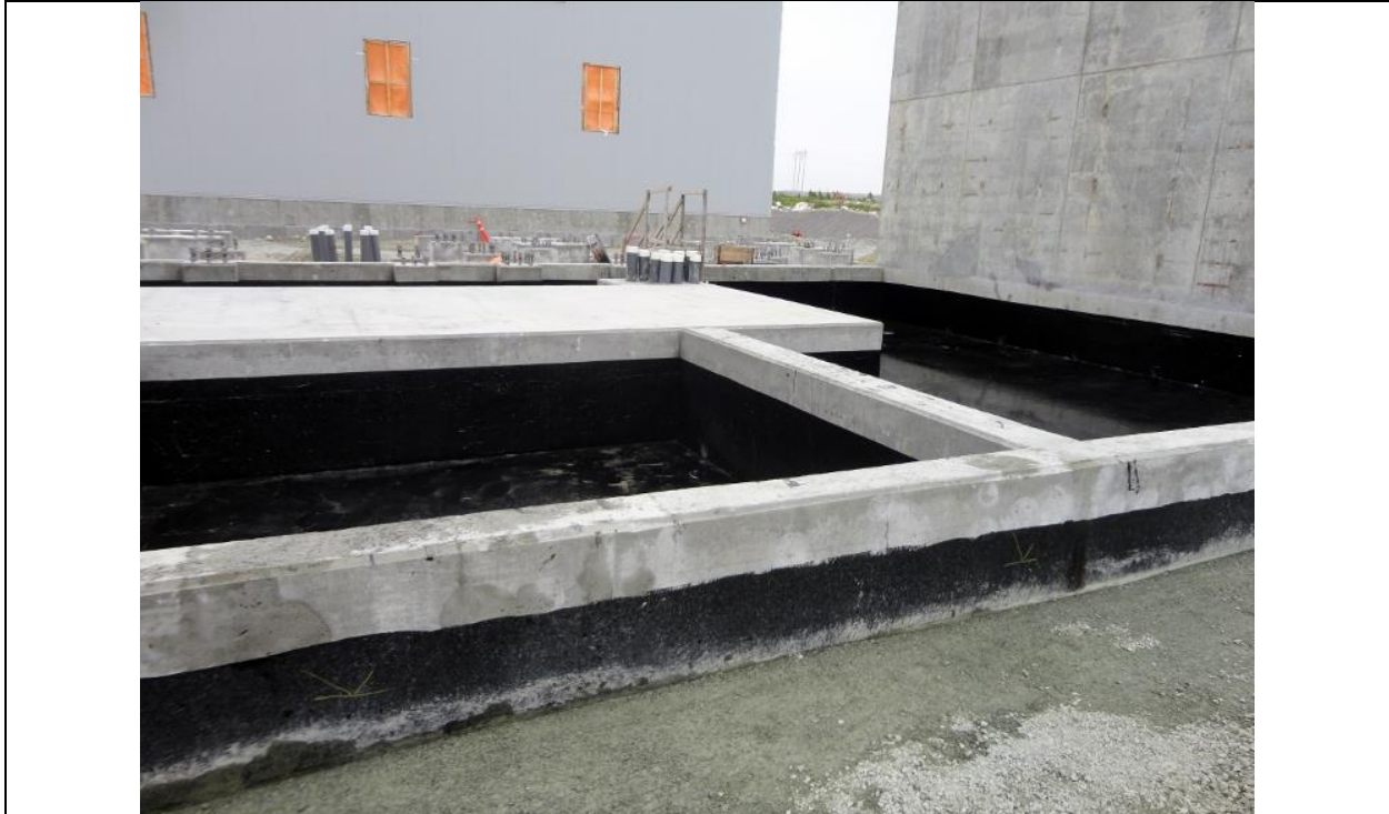
Photo I.7: Soldiers Pond– Converter Transformer concrete pad and containment pit with protective compound applied and cured. (July 15, 2016)
