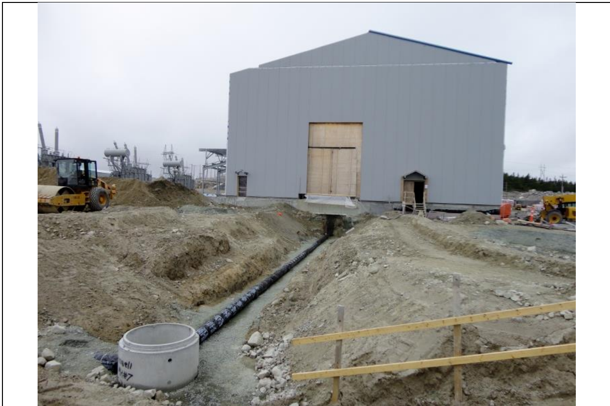
Photo I.18: Soldiers Pond – Synchronous Condenser building, drainage pipe connected to man hole 7 and ready for backfill. (July 15, 2016)
