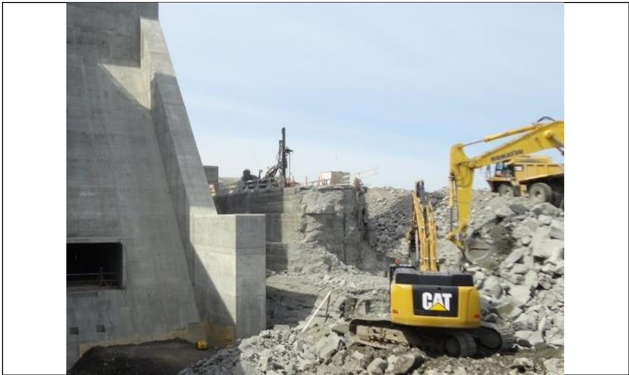
Photo D.4: RCC cofferdam being demolished with a hydraulic hoe ram. (July 13, 2016)
