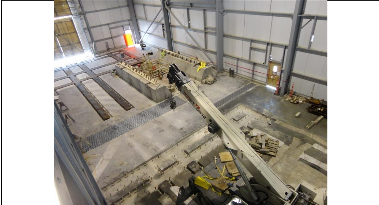
Photo I.13: Soldiers Pond – Synchronous Condensers building- interior view of machine hall with completed footings for unit 1. Floor embedment parts at unit 1 bay are ready for grouting and are yet to be installed at unit 2 bay. (July 15, 2016)
