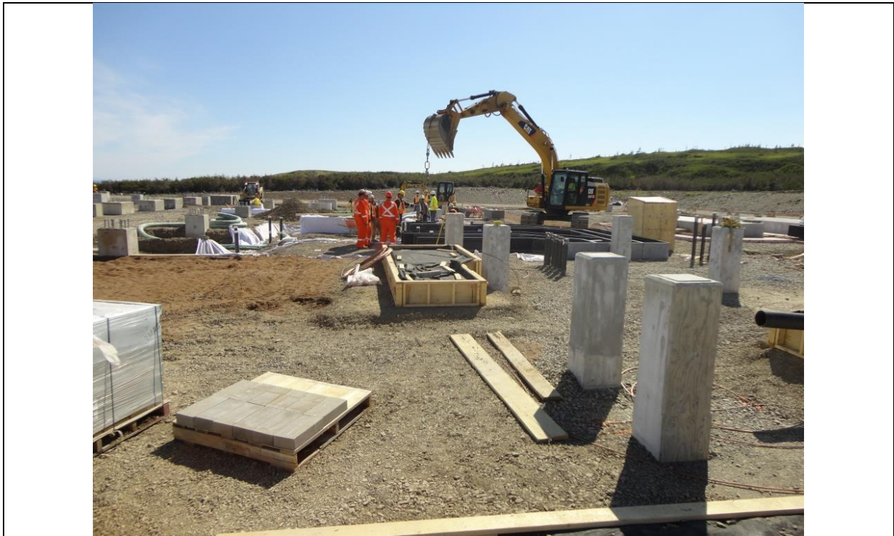
Photo B.6: Transition compound – ongoing work on concrete foundations for gantries and equipment. (July 12, 2016)
