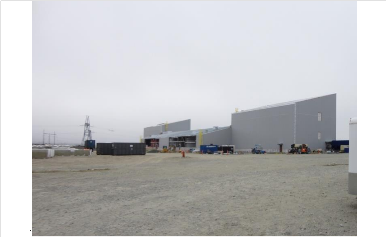
Photo I.1: Soldiers Pond - Converter Station and HVdc yard. (July 15, 2016)
