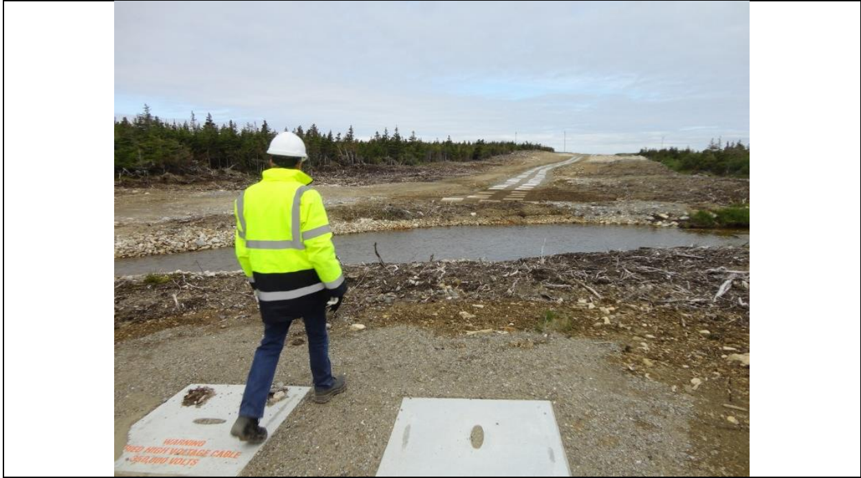
Photo A.7: Creek crossing over the buried cables near the midway point. Further erosion control works are planned to protect the buried cables. (July 12, 2016)
