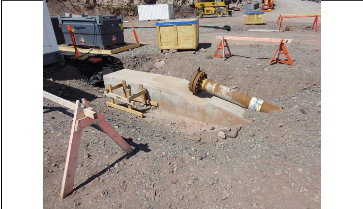
Photo B.3: Anchor point for Cable #2. (July 12, 2016)
