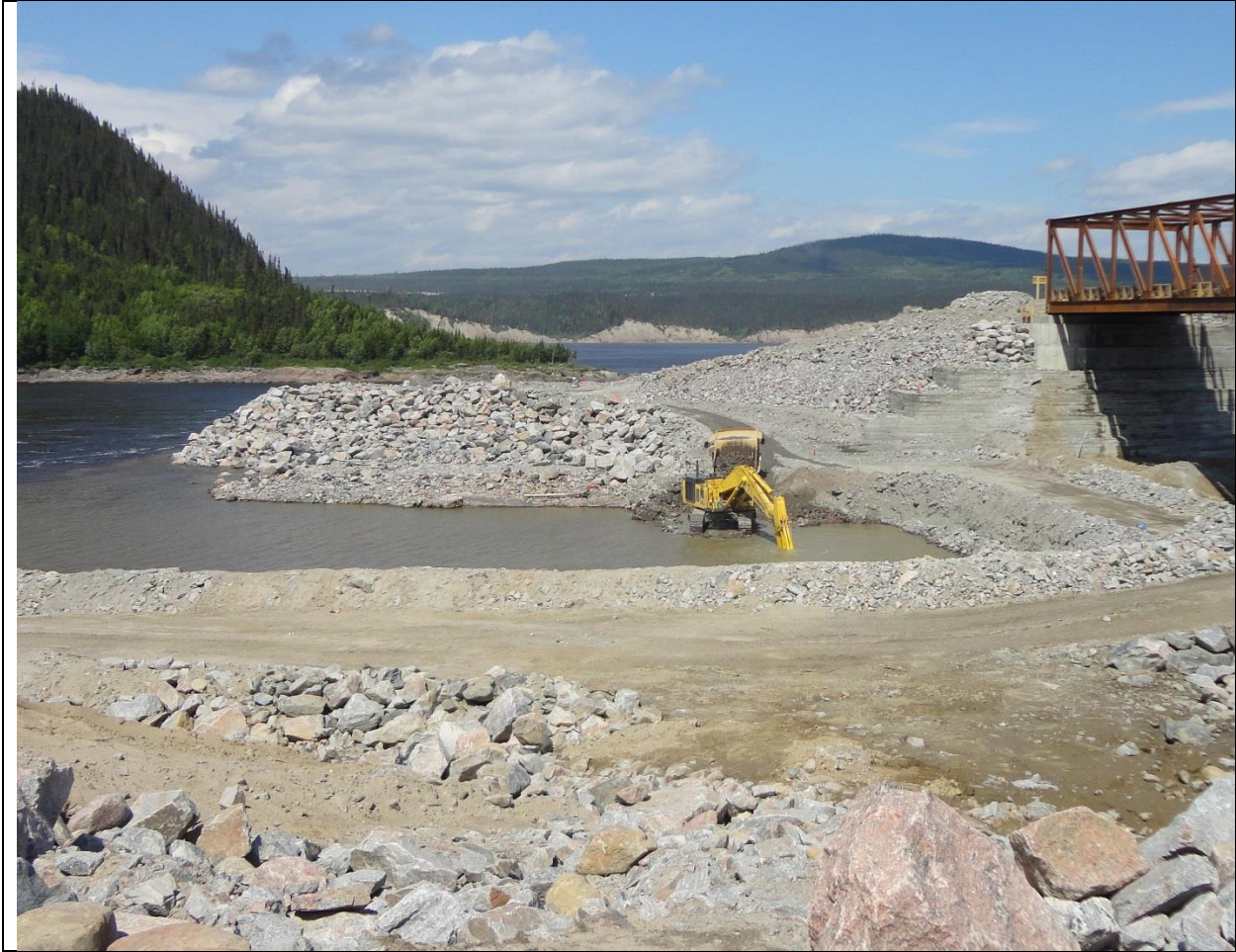
Photo D.15: Preparation of the left starter dyke of the Upstream Cofferdam. (July 13, 2016)
