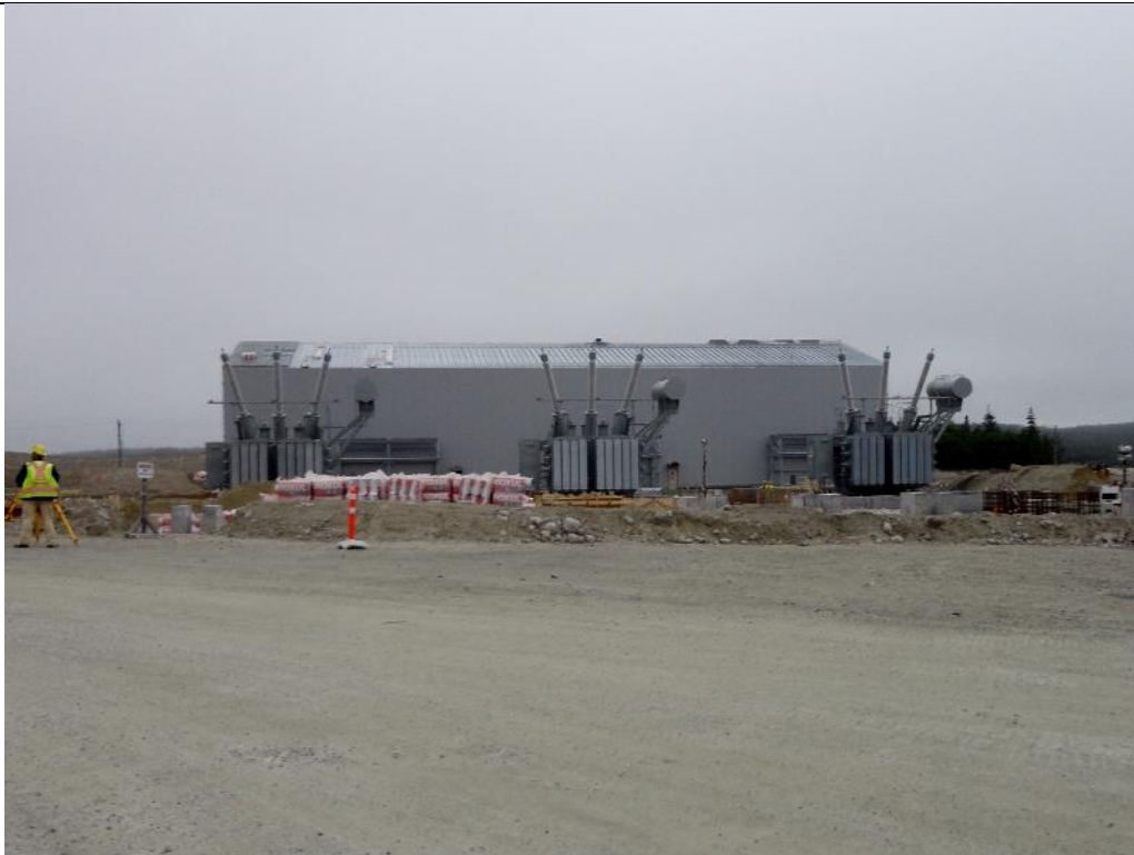
Photo I.12: Soldiers Pond – Synchronous Condensers transformers and the building on the background. (July 15, 2016)
