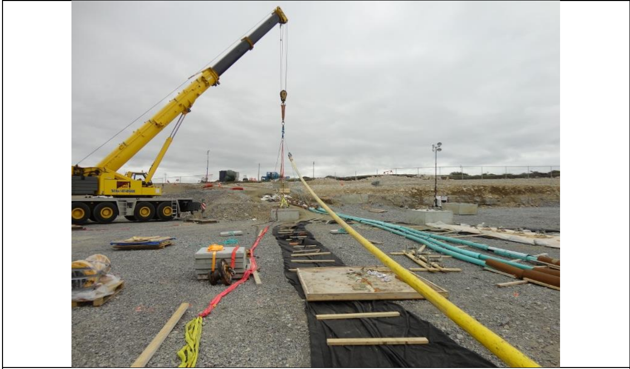
Photo A.5: Cable No.2; final pull work to emplace the cable along the Shoal Cove shoreline work area. (July 12, 2016)
