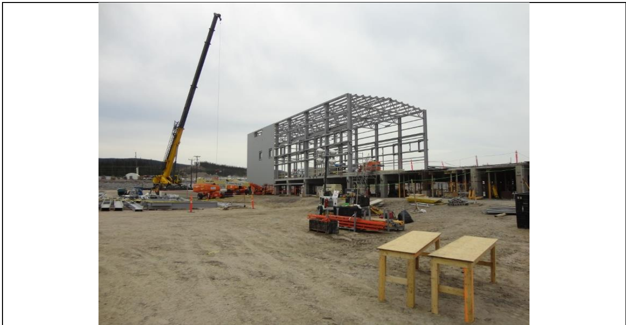
Photo G.4: GIS building with partially erected steel frame. Repair work on the building foundations (at right) was ongoing. (July 13, 2016)
