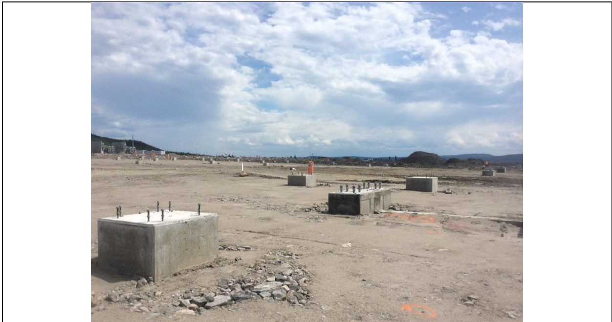
Photo H.2: Complete cast-in-place gantry foundation and pre-cast pole insulator footings – backfilled and ready for equipment installation. (July 14, 2016)
