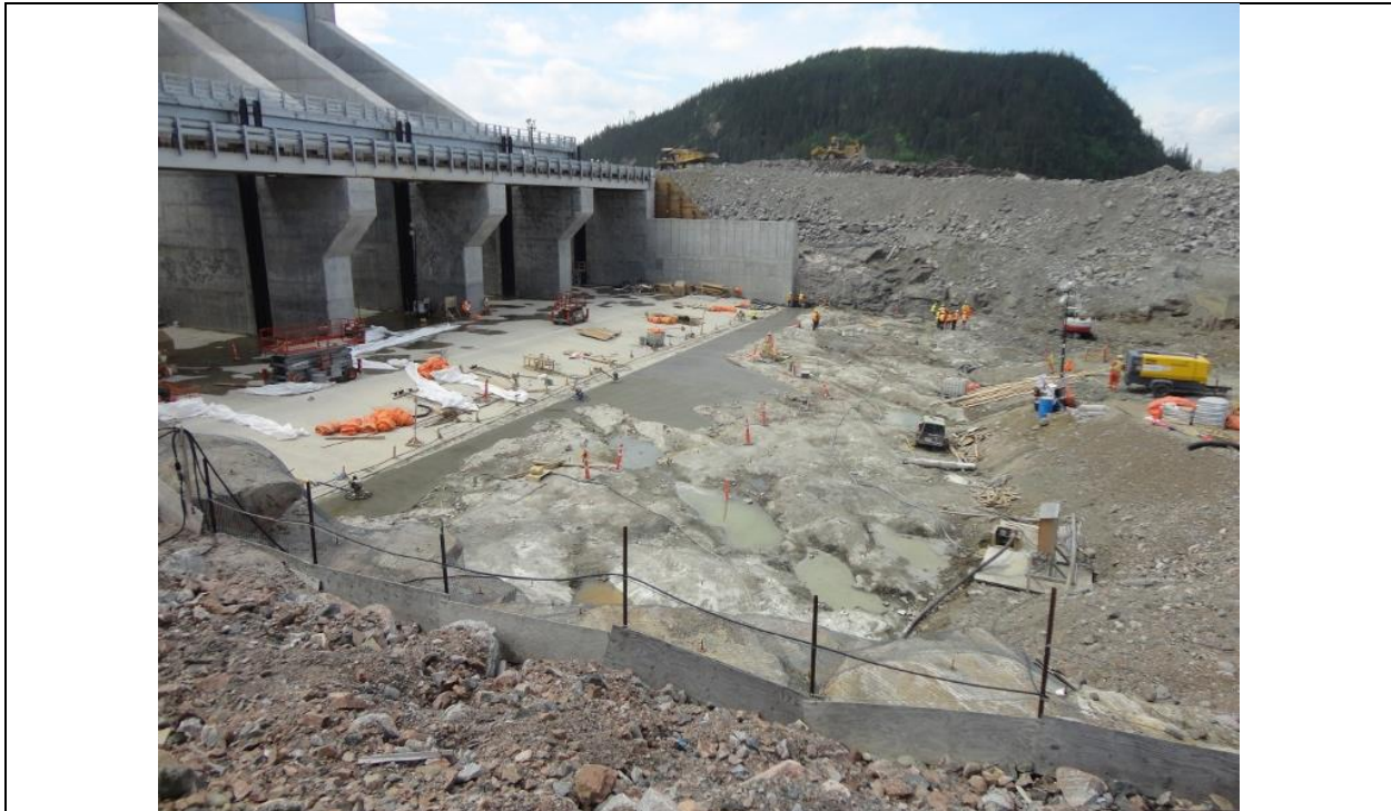
Photo D.14: Preparation of the Spillway apron surface. Dental concrete (dark colored) has been placed in the steel reinforced depressions adjacent to the concrete apron. (July 13, 2016)
