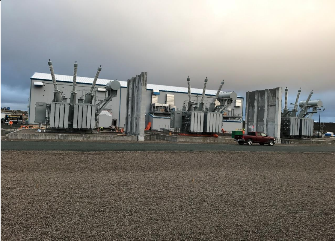
Photo A.7: Main synchronous condenser transformers - fully installed. (November 29, 2016)
