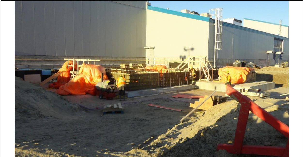
Photo F.6: Foundation preparation works for DC switchyard next to AC/DC converter building. (November 30, 2016)
