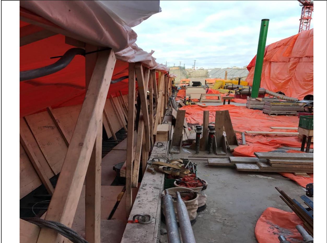
Photo B.13: Unit 1 – top of downstream wall with anchor bolts installed and ready for steel frames erection. (November 30, 2016).
