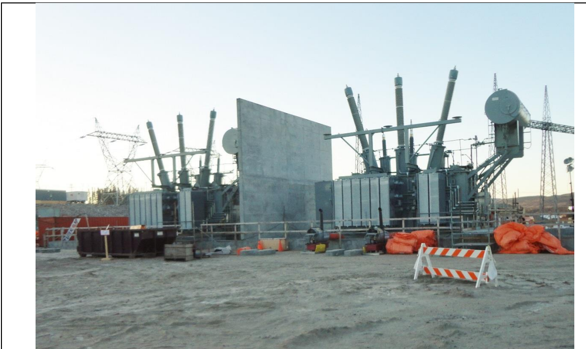
Photo F.12: Installed transformers for future power supply to Goose Bay, (November 30, 2016)
