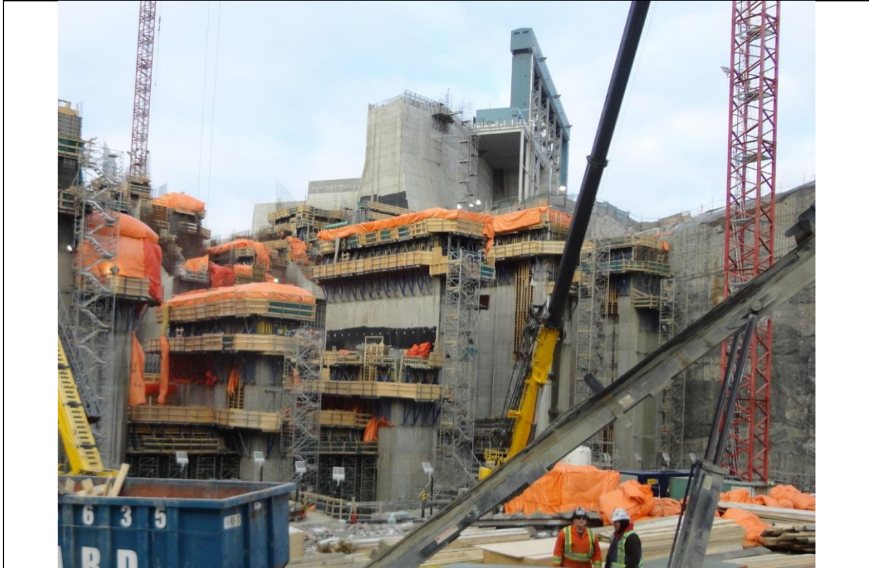
Photo B.3: Looking upstream at the powerhouse; Units 3 and 4 are visible with the Central transition dam and Spillway in the background. (November 30, 2016)
