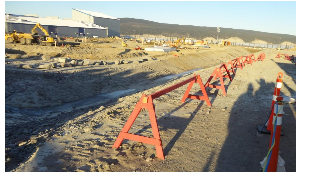
Photo F.4: Foundation preparation works for DC switchyard next to AC/DC converter building. (November 30, 2016)
