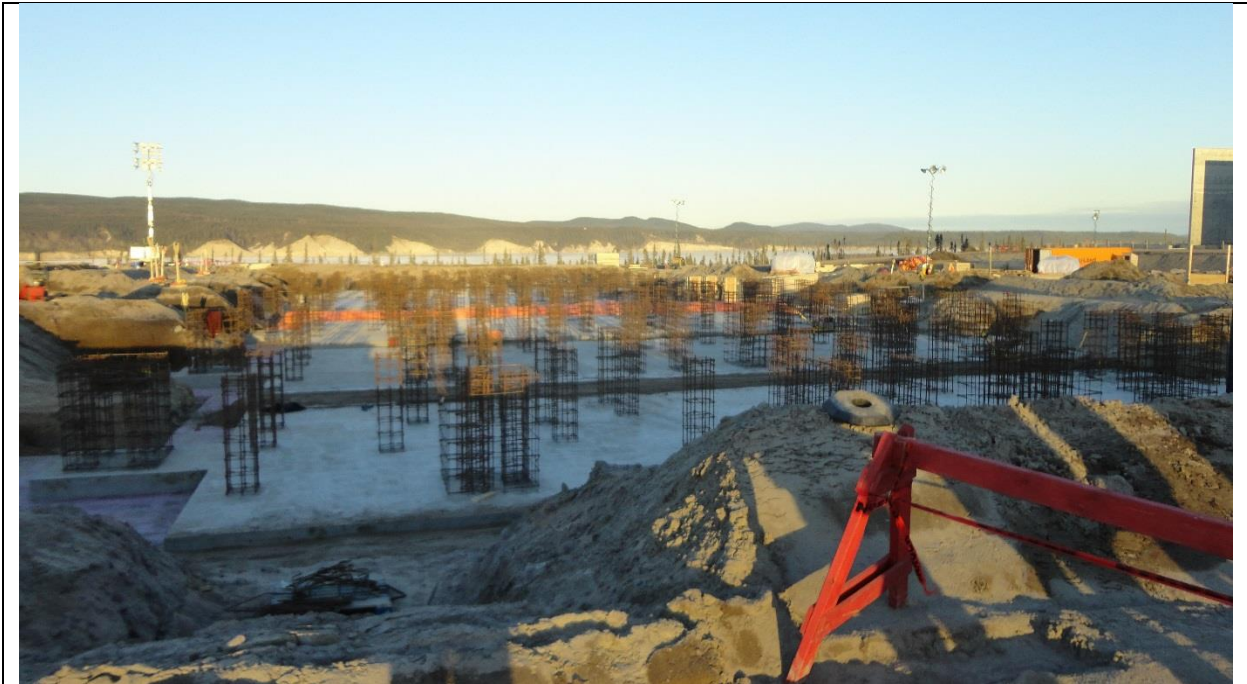
Photo F.7: Foundation works for AC filters equipment next to AC/DC converter building. (November 30, 2016)
