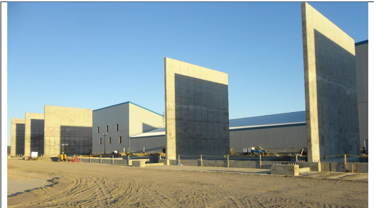
Photo F.8: Blast walls between the converter transformers containment pits at the AC/DC converter building. (November 30, 2016)
