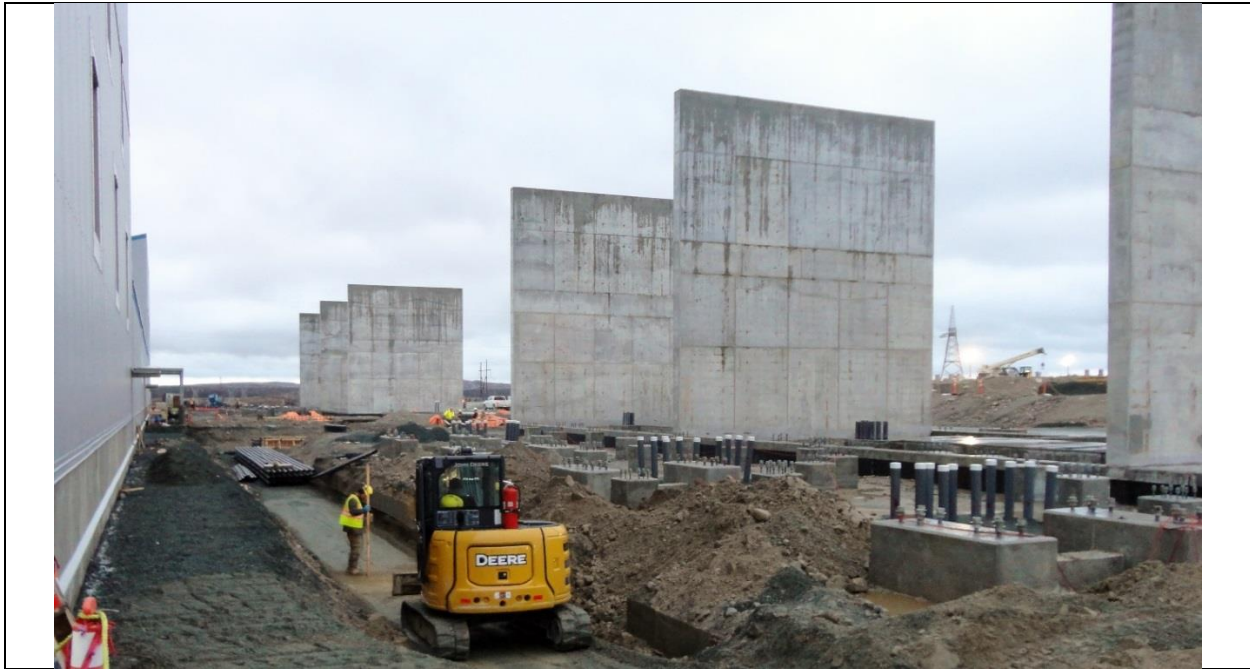
Photo A.13: Transformer blast walls at the converter site. (November 29, 2016)
