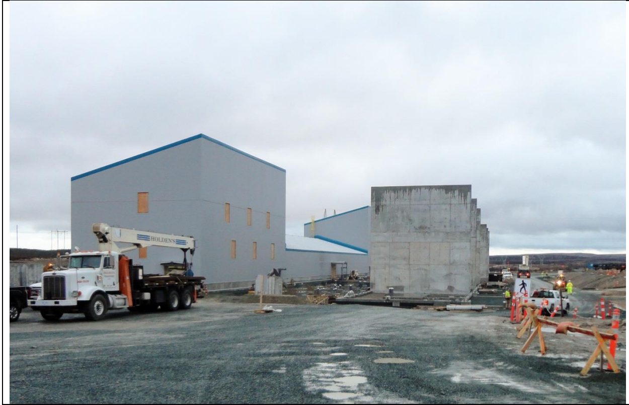
Photo A.11: Converter station building. (November 29, 2016)
