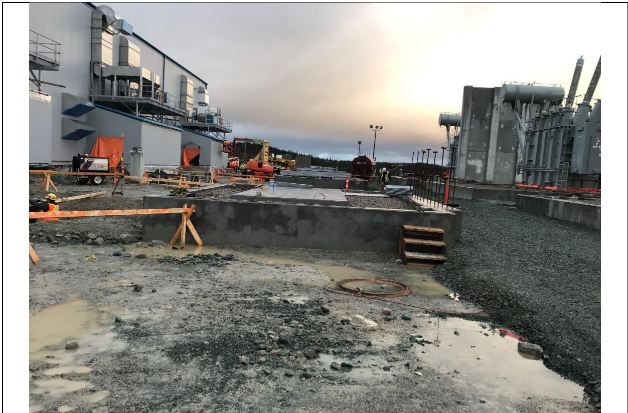
Photo A.10: Containment pits and foundation pads of excitation transformers. (November 29, 2016)
