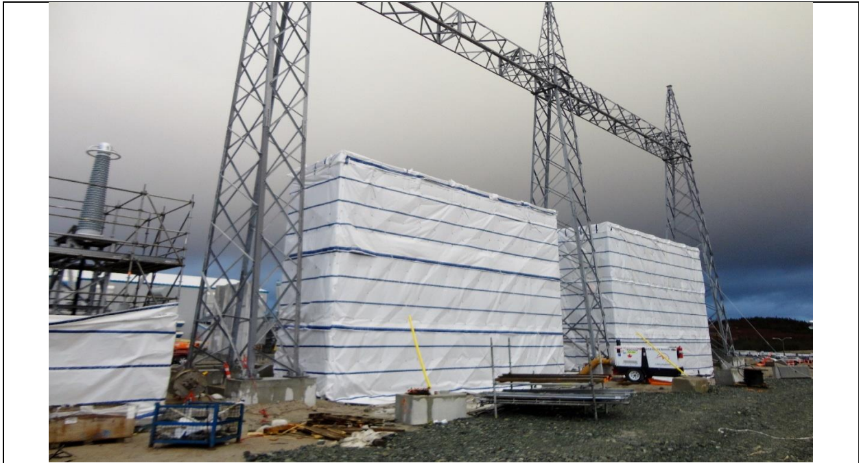
Photo A.9: Gantry for 230kV feeders to SC transformers. (November 29, 2016)
