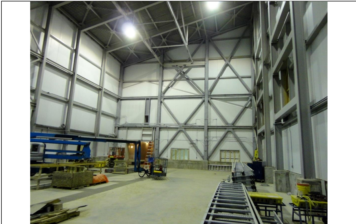
Photo A.12: Interior of the converter building. (November 29, 2016)
