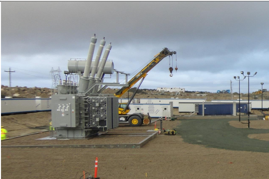
Photo A.8: Spare transformer near the synchronous condenser building. (November 29, 2016)
