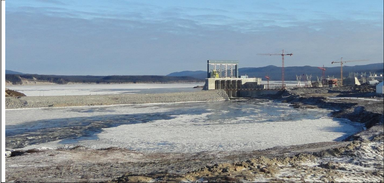
Photo C.3: Upstream pond and spillway approach channel to the right. (November 30, 2016)
