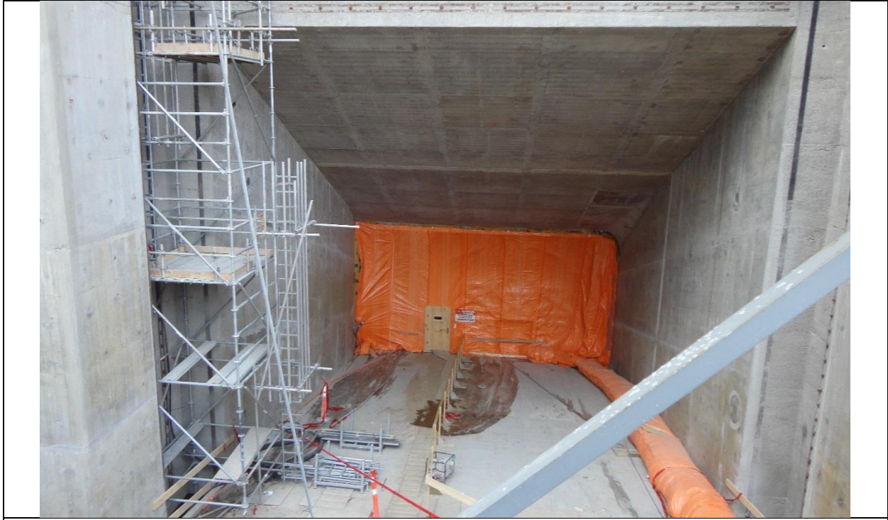
Photo B.5: Unit 2 draft tube water passage. (November 30, 2016)
