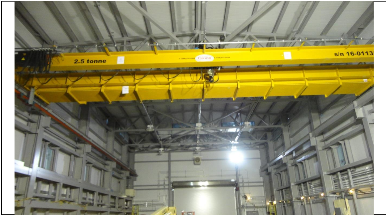
Photo F.9: Overhead crane in the GIS building. (November 30, 2016)
