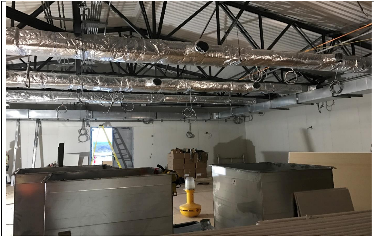
Photo A.4: Interior of switchyard control building – BOP work in progress. (November 29, 2016)
