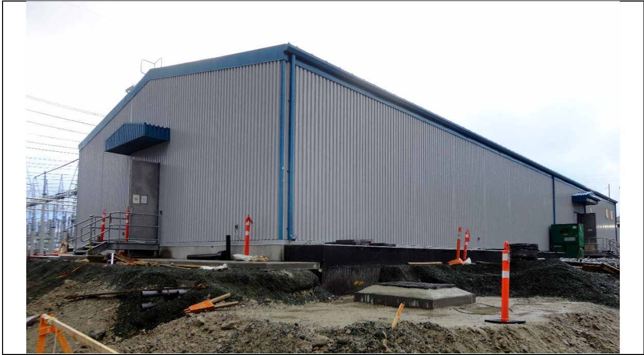
Photo A.3: AC switchyard control building. (November 29, 2016)
