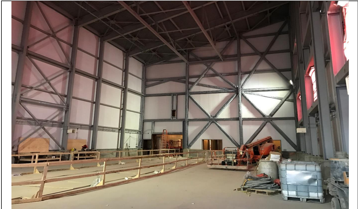
Photo F.3: AC/DC Converter Building - valve hall interior. (November 30, 2016)
