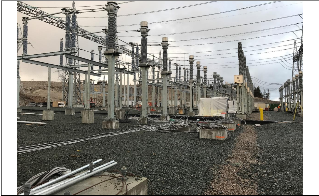
Photo A.2: AC switchyard. (November 29, 2016)
