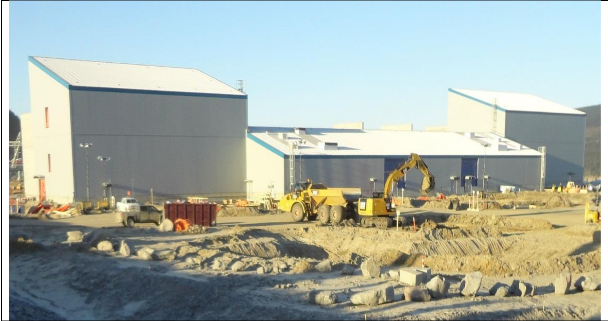
Photo F.1: AC/DC Converter Building, view from the south. (November 30, 2016)
