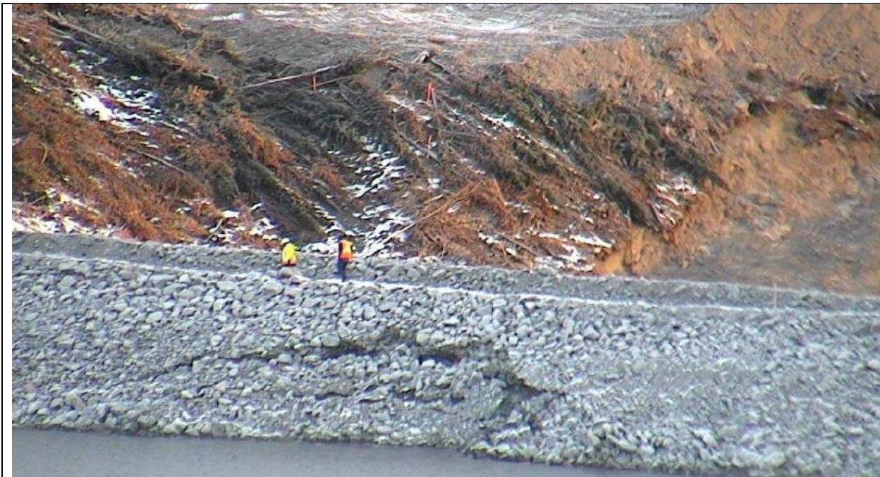
Photo D.2: Slumped area in the upstream face. (Nalcor photo taken shortly after November 15, 2016)
