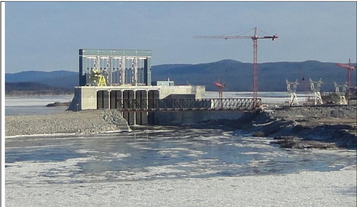
Photo C.4: Closer view of the Spillway approach channel and upstream temporary bridge. (November 30, 2016)
