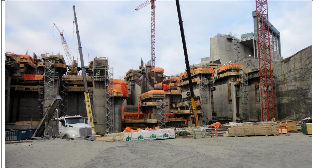
Photo B.1: Looking upstream at the powerhouse; structures of Units 2, 3 and 4 are visible. (November 30, 2016)
