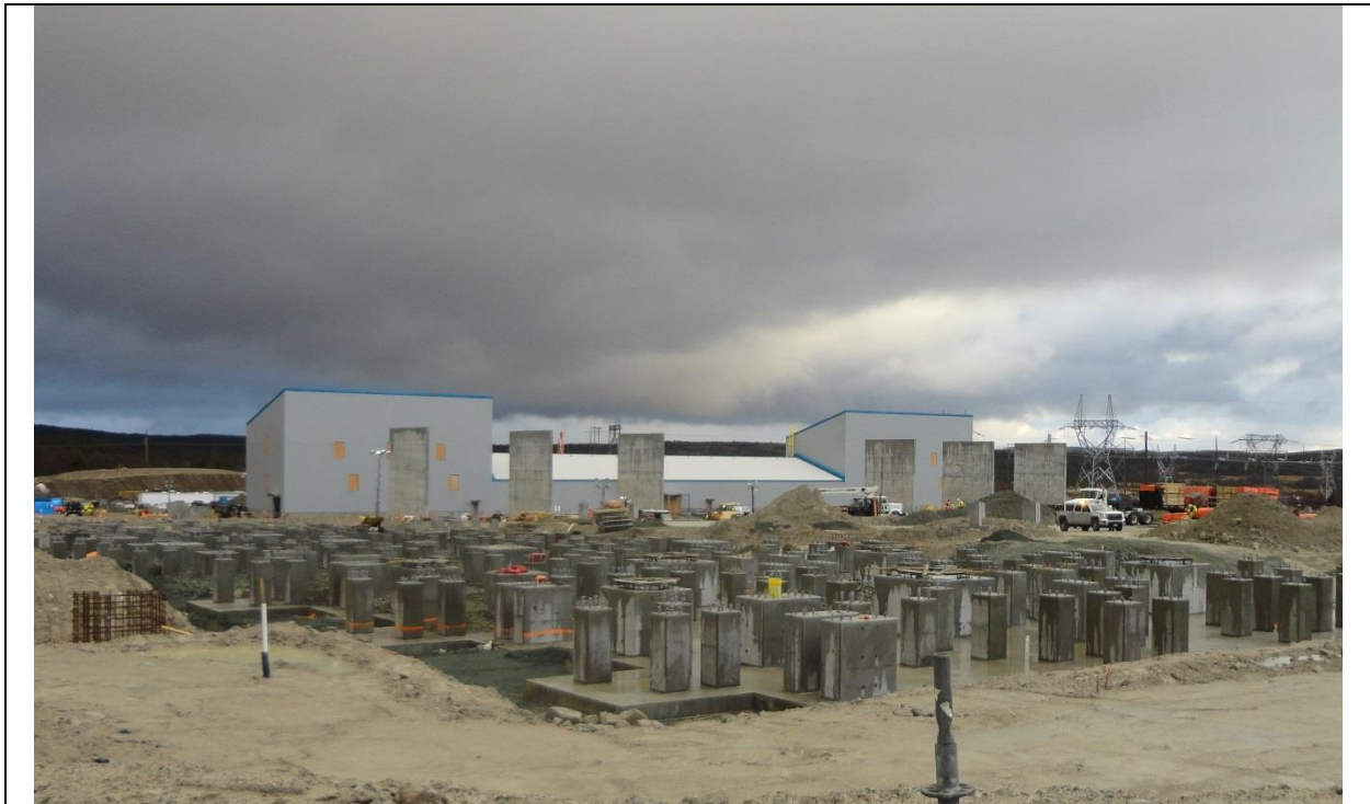
Photo A.14: Converter station - footings for DC (filters) yard in the foreground. (November 29, 2016)
