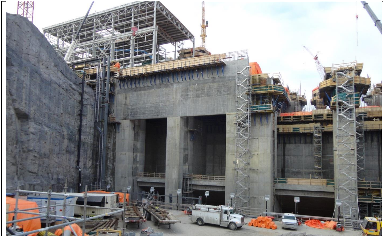
Photo B.2: Looking upstream at the powerhouse; service bay steel framework and concrete structures of Units 1 and 2 are visible. (November 30, 2016)
