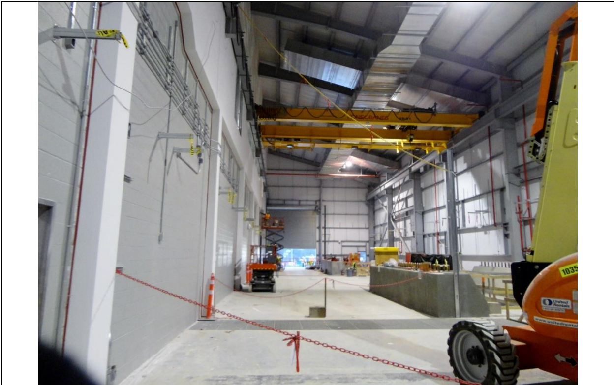
Photo A.6 Interior of synchronous condenser building. (November 29, 2016)
