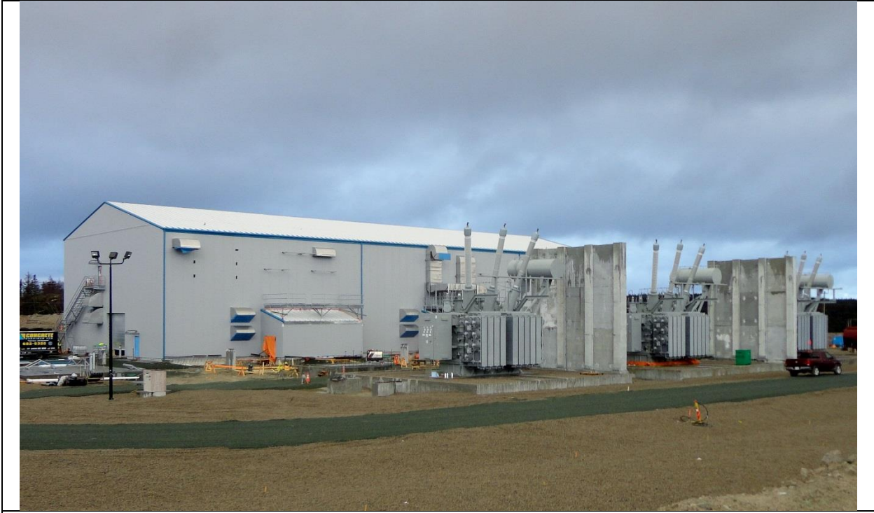
Photo A.5: Synchronous condenser building and transformers. (November 29, 2016)
