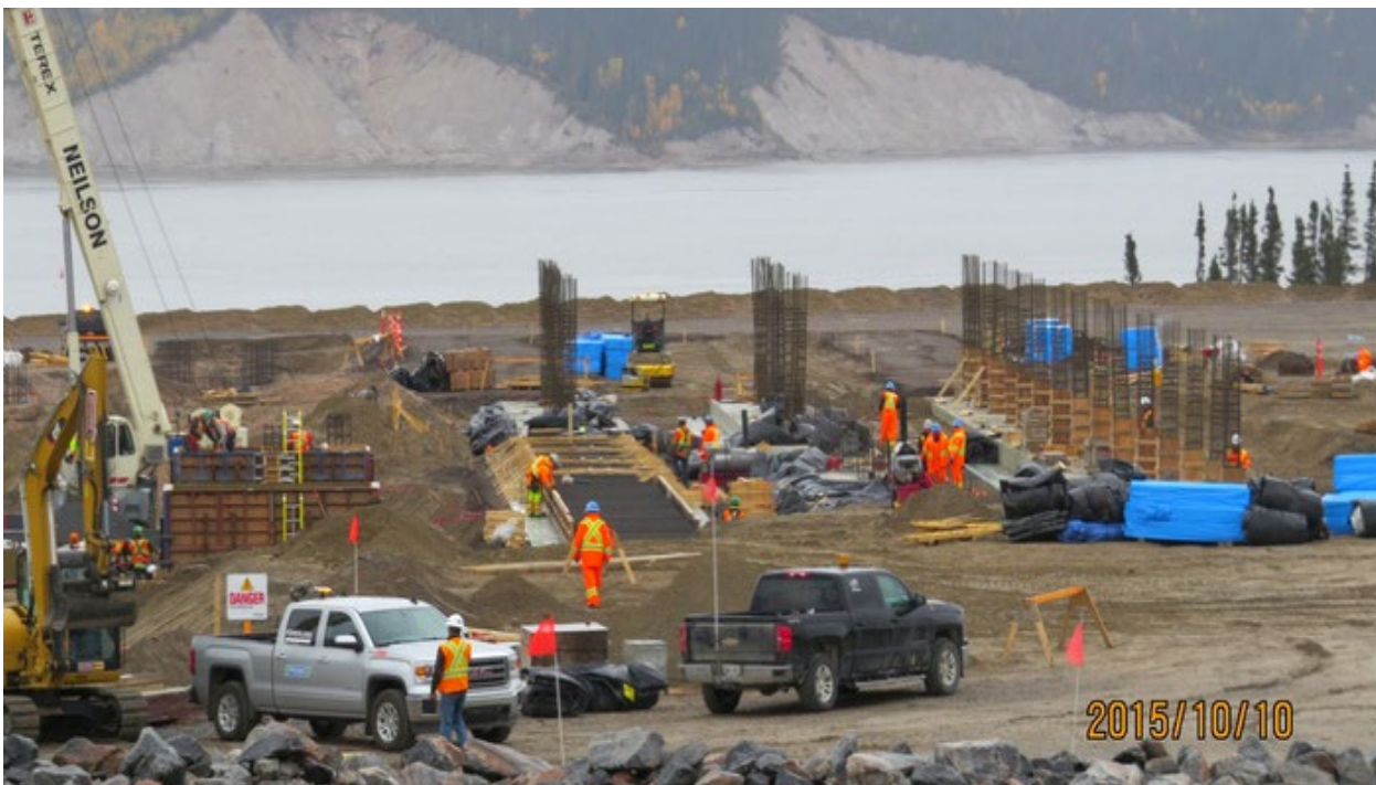
Muskrat Falls Switchyard – October 2015
