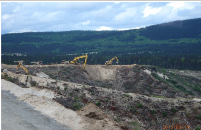
CH0008: Construction of North Spur Stabilization Works- Overview of overburden excavation works on upper slopes of the downstream
