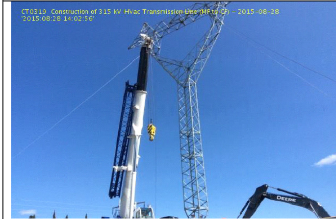
CT0319: Construction of HVac Transmission Line-Erection crew lowering tower on access AT 90
