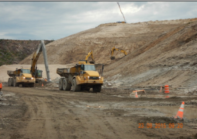
CH0008: Construction of North Spur Stabilization Works- Upstream cement bentonite cut-off wall panel installation works
