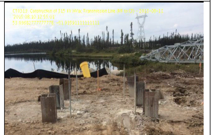
CT0319: Construction of HVac Transmission Line: Installation of piles and anchors, foundations A,B,C,D, on structure 248 L2
