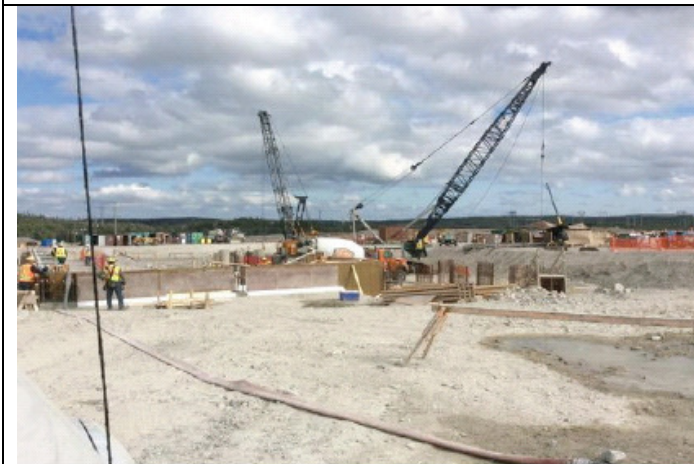
Ongoing construction of switchyard, synchronous condenser and converter station at Soldier's Pond
