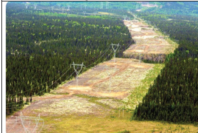
CT0319: Towers erected and power line conductor strung along the HVac Transmission Line between MF and CF
