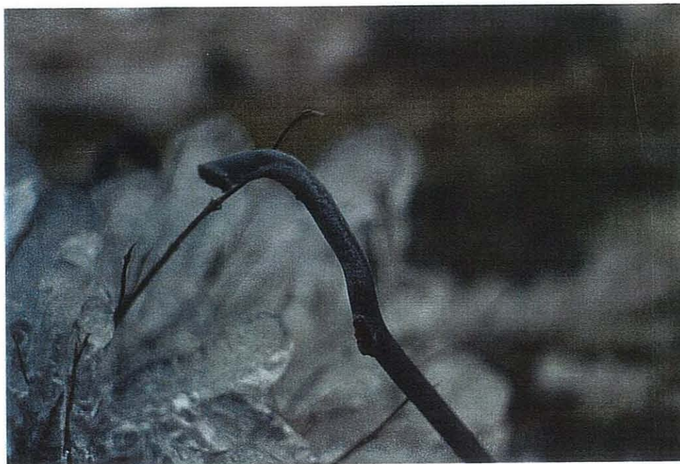
Photo No. 2-2 April 1984 Failed single eye Anchor Rod ( TL-217 )
