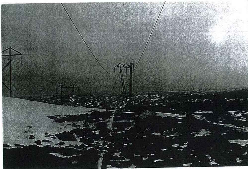
Photo No. 2-3 April 1988 Failure of bridge on Suspension Tower (TL-217) at Hawke Hill
