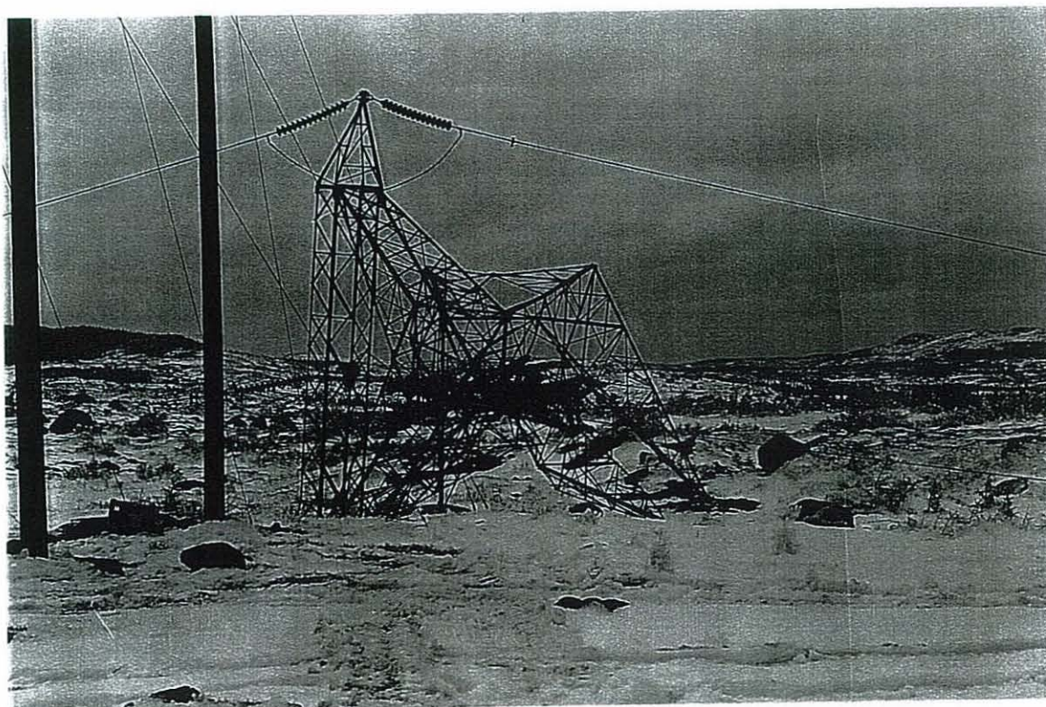
Photo No. 2-4 April 1988 "C" Tower (Heavy Angle) Failure on TL-217
