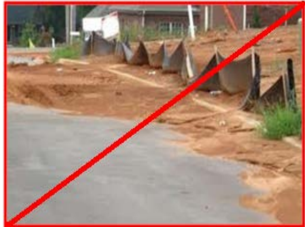
Figure 5-37: Examples of poorly installed silt fences
