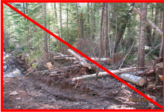
Figure 5-1: Poorly cut and piled wood
