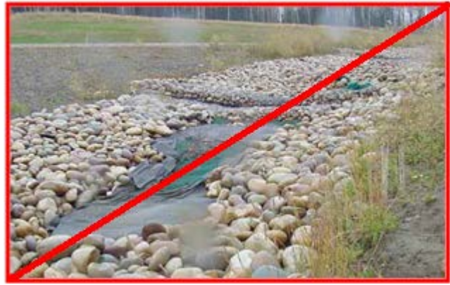
Figure 5-28: Photograph of failed Rip Rap Protection
