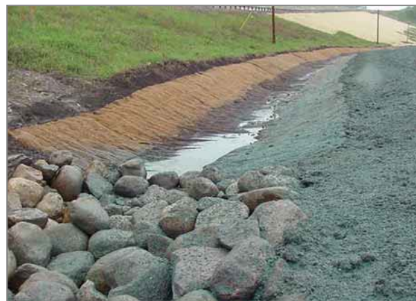
Figure 5-26: Photograph shows erosion control blanket on slope and erosion control mat in channel
