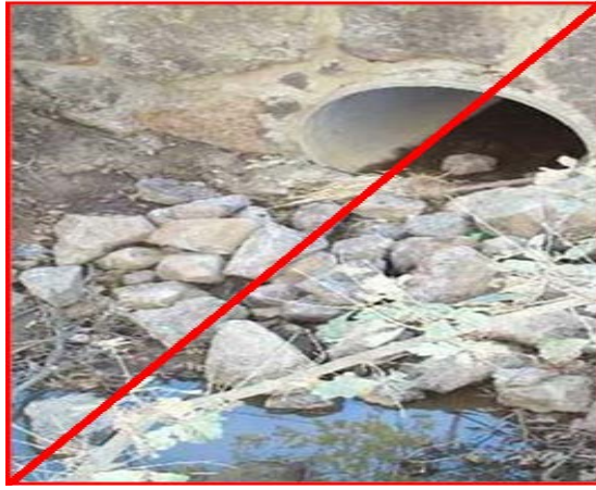
Figure 5-32: Incorrect Construction of Rock Energy Dissipaters
