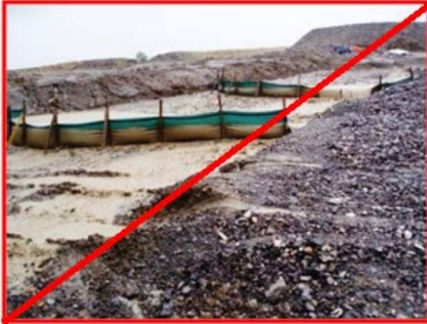
Figure 5-36: Examples of poorly installed silt fences
