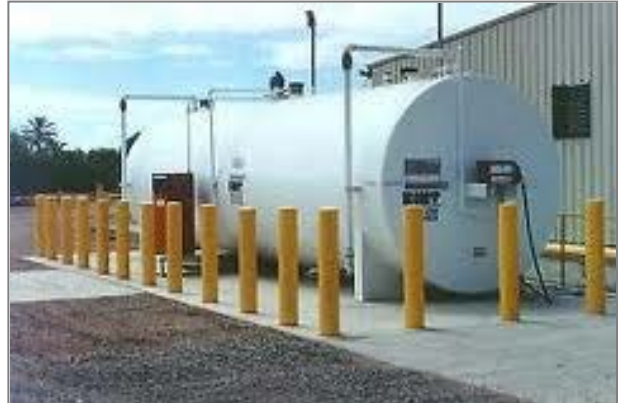
Figure 5-6: Fuel storage on concrete pad
