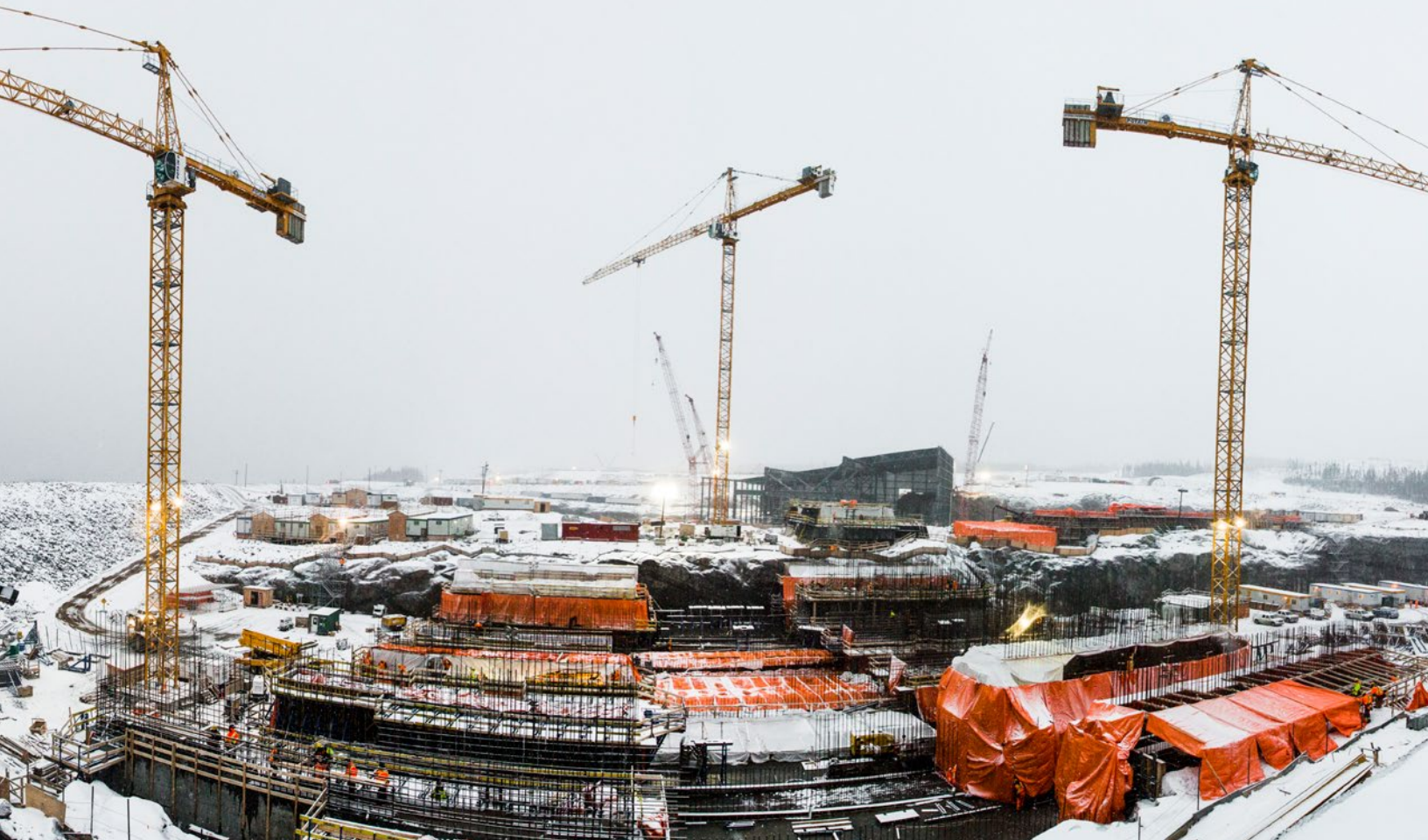
Construction of the Muskrat Falls hydroelectric generating facility in Labrador. Now in the third year of construction, the project is generating significant employment and business benefits for Newfoundland and Labrador.
